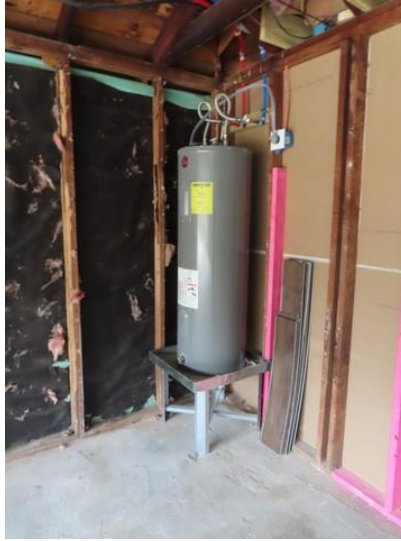
Temperature relief lines/valves.
