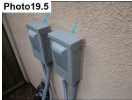
Penetration Sealants/ Maintain
