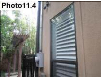
Penetration Sealants/ Maintain
