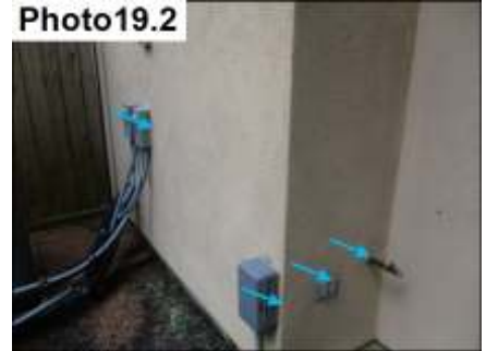
Penetration Sealants/ Maintain
