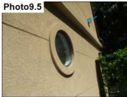
Penetration Sealants/ Maintain
