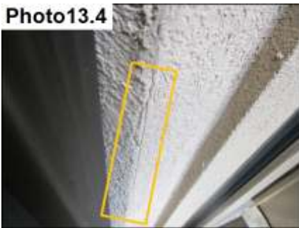
Control Joint Cracks/ Seal
