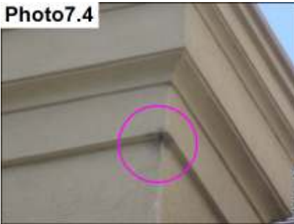
Water Stains/ Clean
