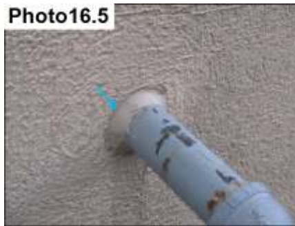
Penetration Sealants/ Maintain
