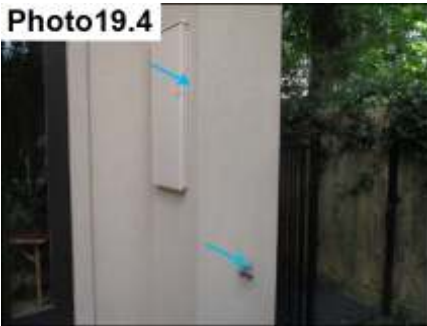
Penetration Sealants/ Maintain
