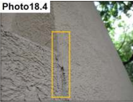
Cracks/ Seal Or Repair
