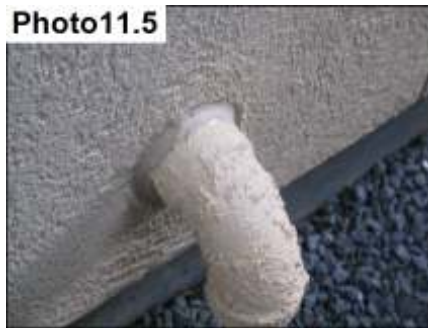
Penetration Sealants/ Maintain
