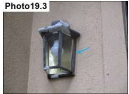
Penetration Sealants/ Maintain
