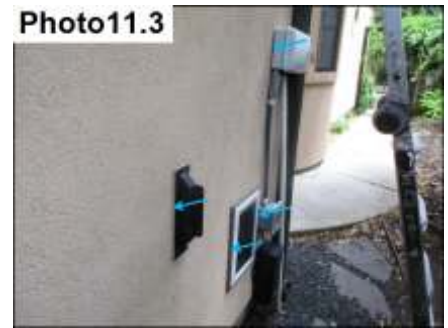
Penetration Sealants/ Maintain
