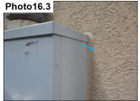
Penetration Sealants/ Maintain
