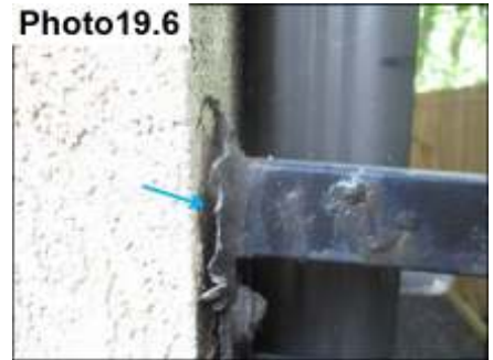
Penetration Sealants/ Maintain
