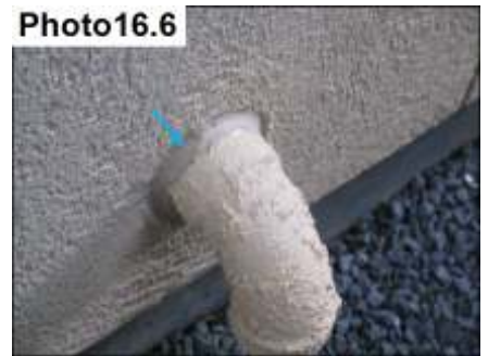
Penetration Sealants/ Maintain
