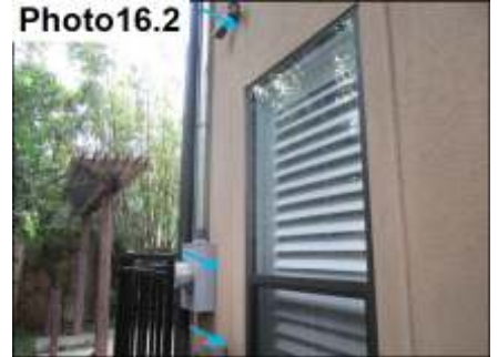
Penetration Sealants/ Maintain
