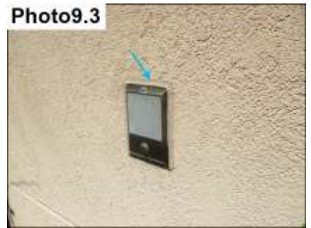
Penetration Sealants/ Maintain
