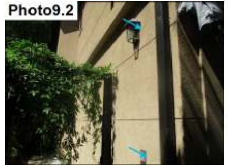
Penetration Sealants/ Maintain
