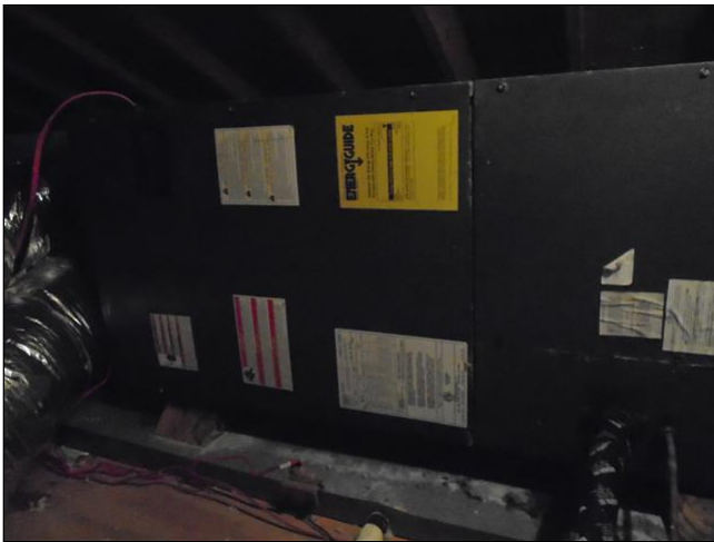
A. Item 1(Picture) Heating Unit
