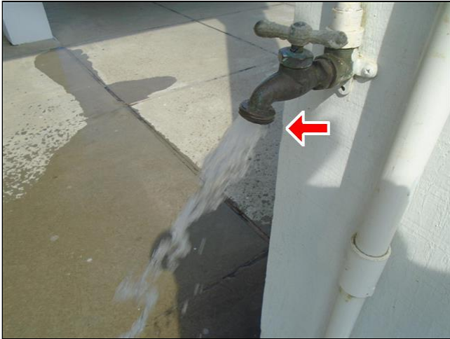
A. Item 6(Picture) No back flow preventer
