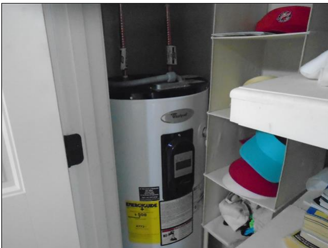
C. Item 1(Picture) Water Heater
