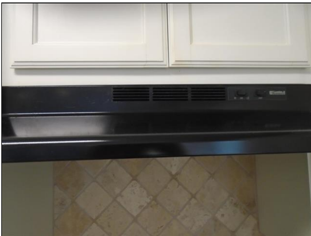
C. Item 1(Picture) Range Hood
