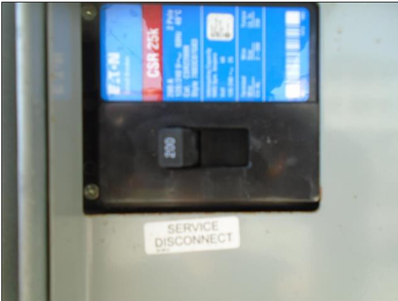
A. Item 1(Picture) Main Breaker
