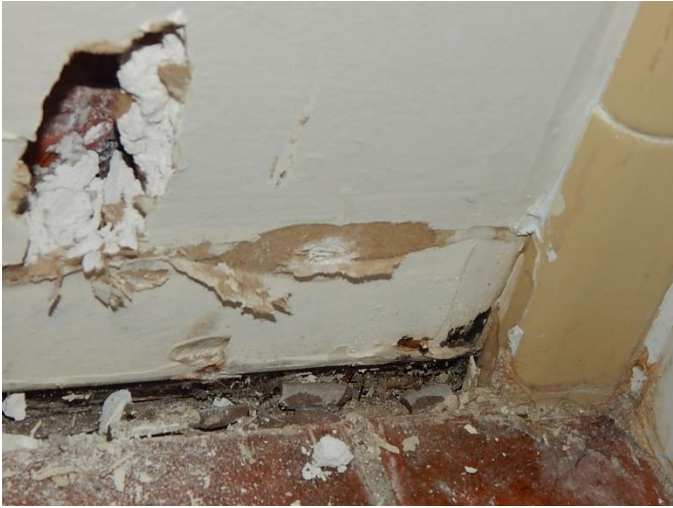
Mold growth was observed at the base of the wall beside the shower/tub fixture wall in the master bathroom
