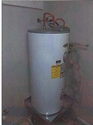
Overview of water heater(s)
