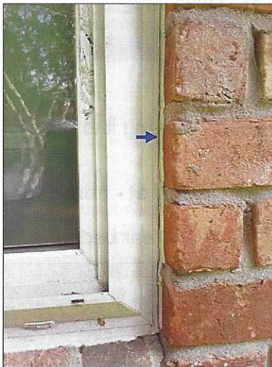
-Sealant is needed around some of the windows between the window framing and exterior brickwork to help prevent water penetration, recommend checking all windows for proper sealant. Mainly at - rear
