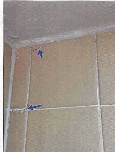
-Cracked or missing tiles were noted in the tub shower surround or shower stall, recommend repairs to help prevent water penetration to underlying materials. Unable to determine the condition of underlying materials. Mainly at - master bathroom
