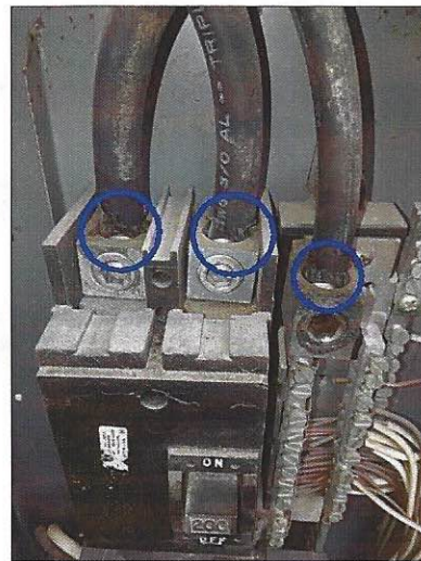
-There is no antioxidant on main aluminum feeds to the panel box. This should be used to help prevent overheating.
