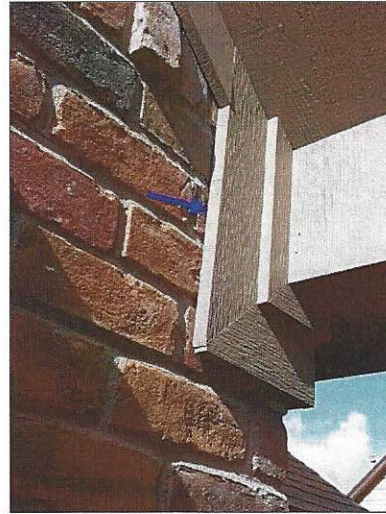
-Recommend sealing between the trim and brickwork to help prevent water penetration. Mainly at - front right
