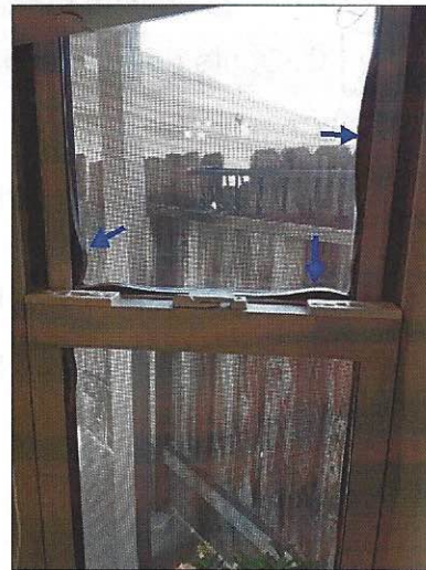
Indications are that the window seals are defective and may lead to a broken thermal seal in the future. Mainly at- breakfast nook
