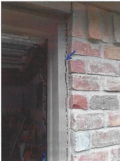
-Recommend sealing between the trim and brickwork to help prevent water penetration. Mainly at - garage
