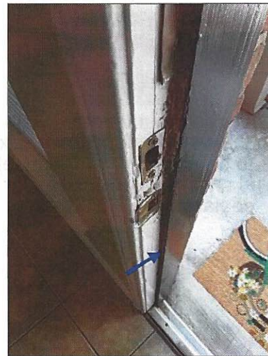
-The weather strip is missing around the door, causing it to not seal properly. Mainly at - back door
