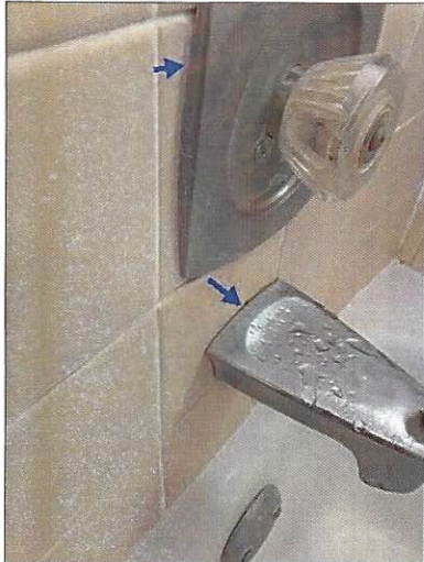
-All tub shower faucets and spouts should be sealed to help prevent water penetration behind the fixture.
