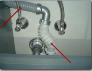
The accordion type drain is not approved for the master sink drain.
