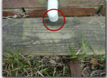
The temperature pressure relief valve leaks to the exterior of the house.
