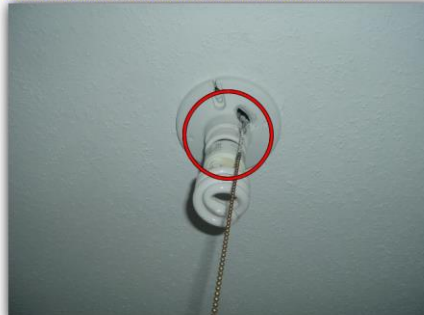
The rear right bedroom closet light fixture is defective and a fire hazard
