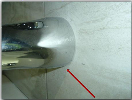
The master tub spout leaks water past the gasket.
