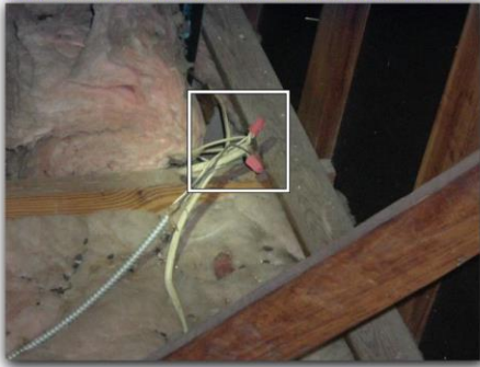
The open electrical junctions in the attic require junction boxes and are a fire hazard.
