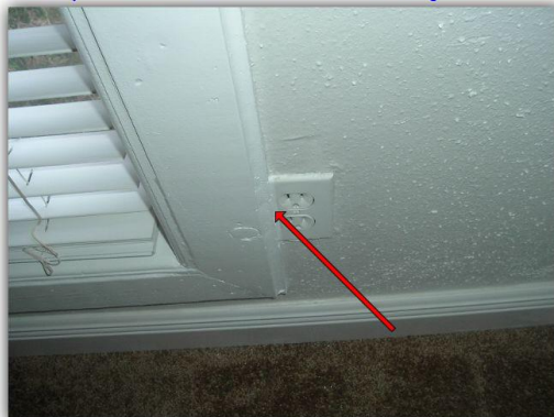
The wall receptacle was located behind the window trim at the rear right den wall.
