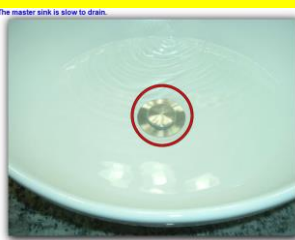
The master sink is slow to drain.
