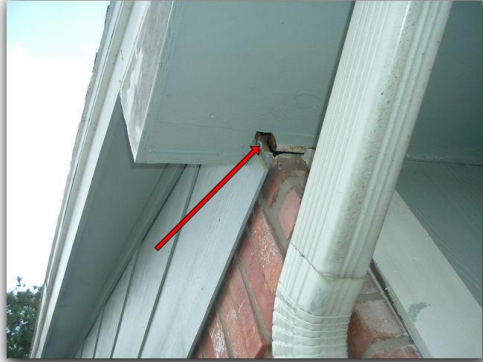
There is missing trim at the rear right of the house.
