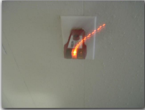
The front wall receptacle at the garage conversion bathroom tested open ground.
