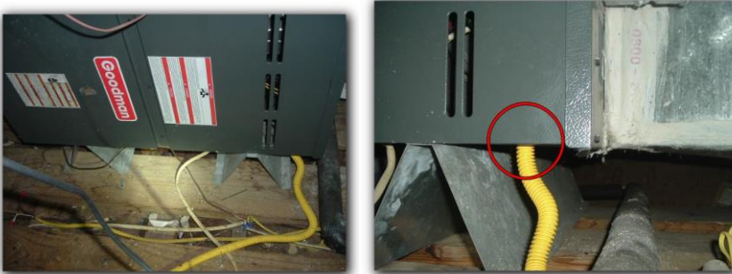
The gas flex line is not permitted in the appliance cabinet. Must be hard piped.
