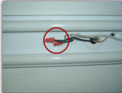
There are open electrical junctions at the utility room ceiling light
