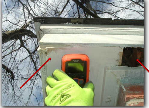
The soffit at the front of the house has active water penetration/decay.
