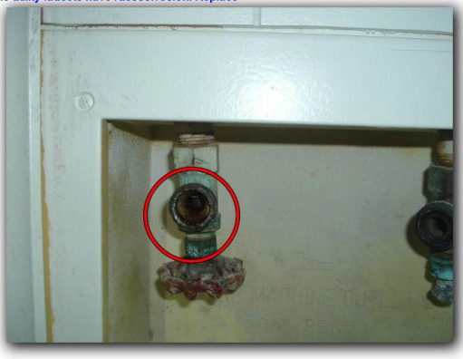
The utility faucets have rust/corrosion. Replace
