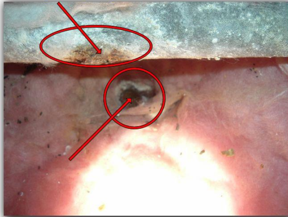
The rusted out galvanized plumbing in the attic leaks.
