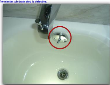
The master tub drain stop is defective.
