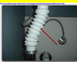
The accordion type drain line is not approved for the guest bathroom sink.
