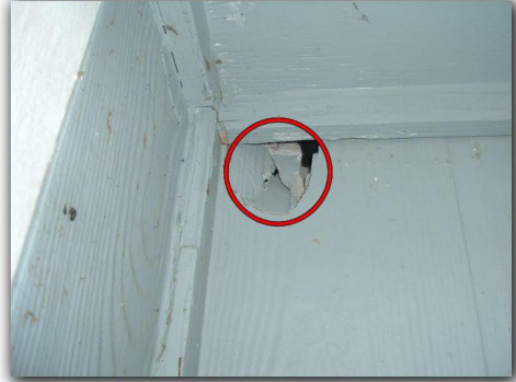
There is damaged siding at the upper rear of the house.
