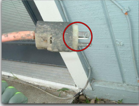
The extension cord at the rear of the house is not approved for branch wiring.
