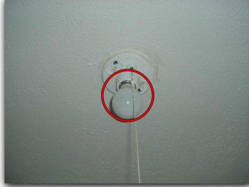
The uncovered closet light in the garage conversion was non functional and a fire hazard.
