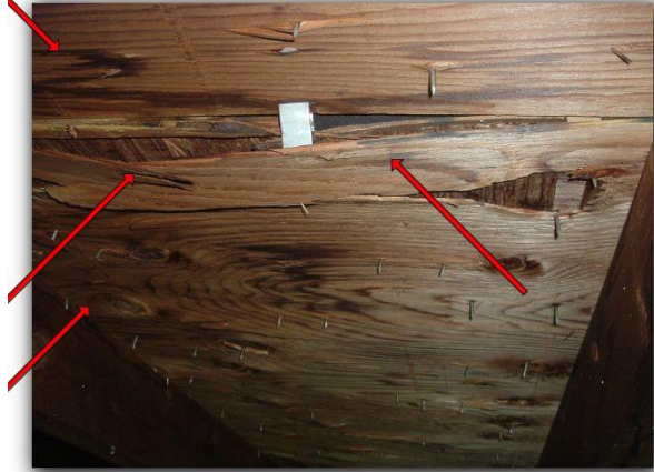
There is evidence of roof leaks/decayed decking in the attic.
