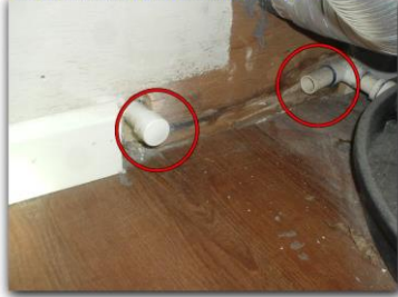
The emergency pan drain line was not connected to the exterior drain
