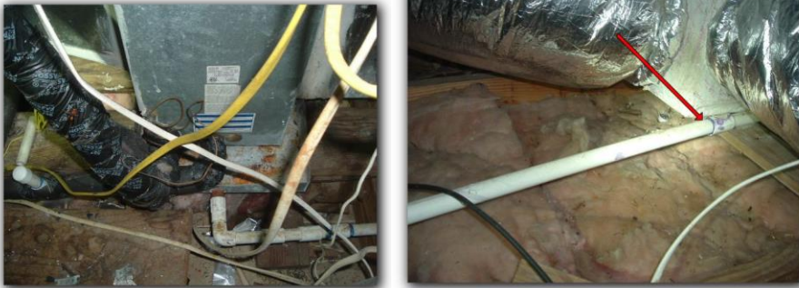
The emergency pan drain line has a negative slope to the drain
