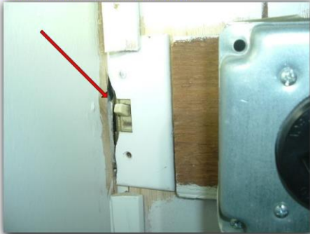
The left utility room wall switch is located too far in the wall.
