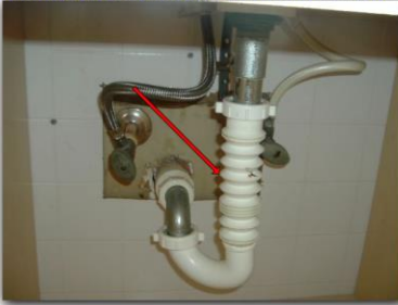
The accordion type drain is not approved for the garage conversion bathroom sink.
