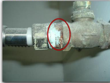
There is evidence of rust at the shut off connection
