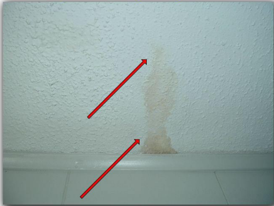
There is active water penetration on the utility room ceiling.
