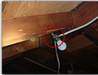
The exposed wiring at the attic lights is a fire hazard.
