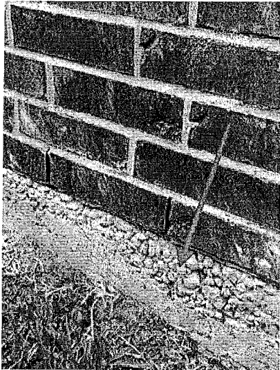
There is some honeycombing on the left-hand side of the house.
