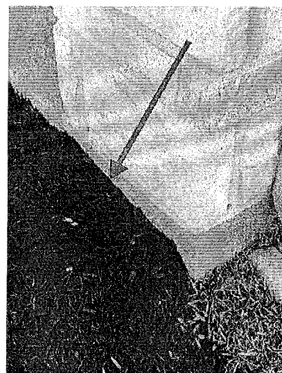
The grading at the front of the house is too high there should be 6 inches of clearance from the top of the ground to the bottom of the siding.
