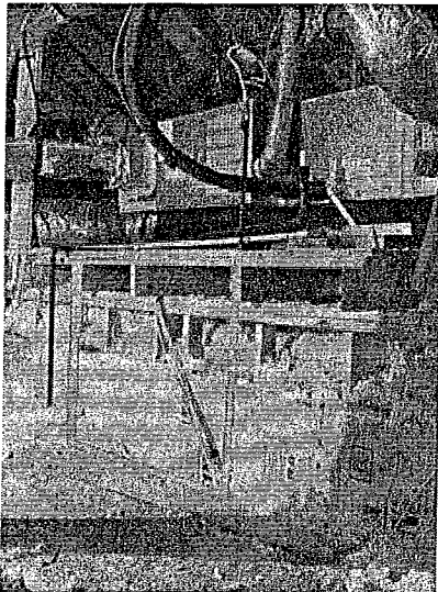
There is not a proper set of steps or ladder to access the equipment in the attic space.
