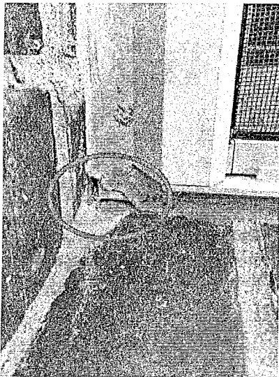
There are multiple locations where the caulk does not fully seal along the exterior side of the window frame.
