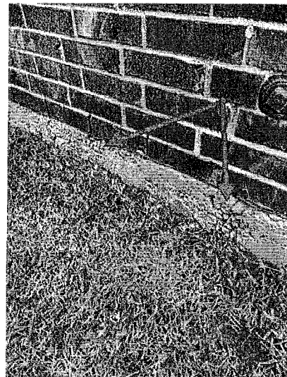
There is some honeycombing on the right-hand side of the house.
