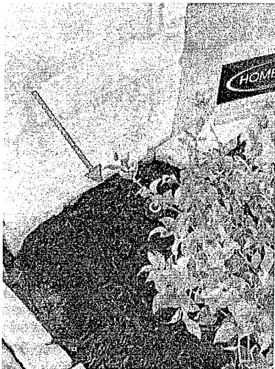
The grading at the front of the house is too high there should be 6 inches of clearance from the top of the ground to the bottom of the siding.
