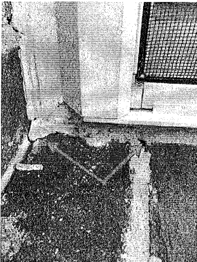
There are multiple locations where the caulking does not fully seal along the exterior side of the window frame.
