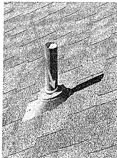
The roof jack right hand side of the house is not installed properly around the vent pipe.
