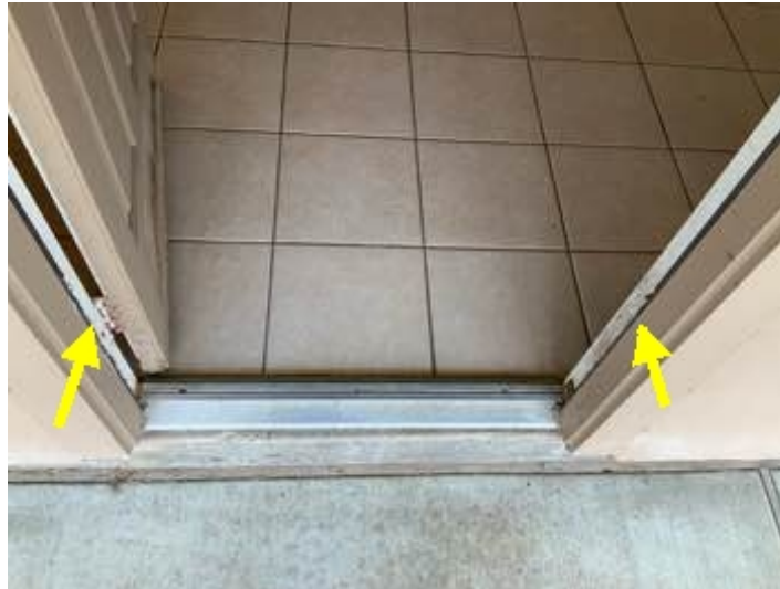
Damaged weather stripping at the rear egress door.
