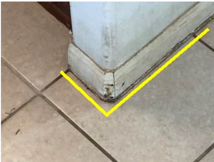
Moisture damage on the baseboards in the kitchen.
