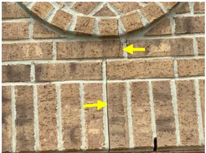
Brick and mortar step crack on the front of the garage.
