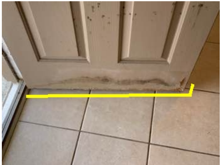
Damaged and deteriorating rear egress door.
