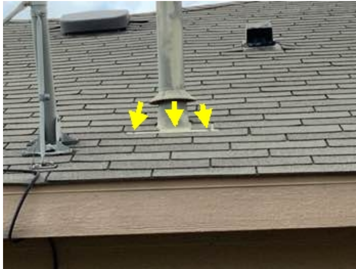
Exposed nail heads on the vent flashing.
