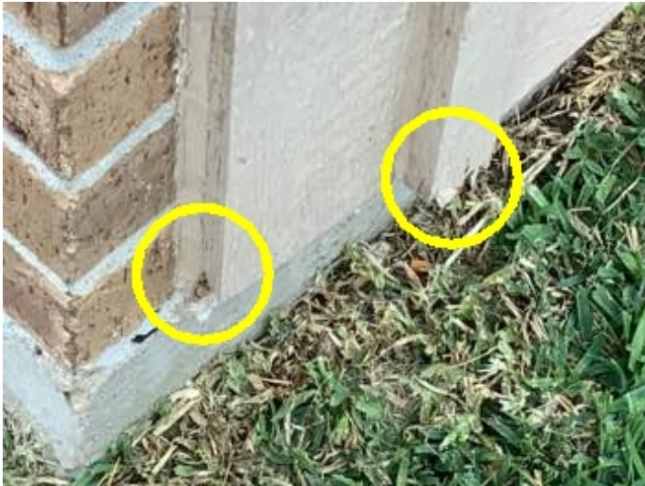
Damaged and deteriorating trim on the right front corner of this home.
