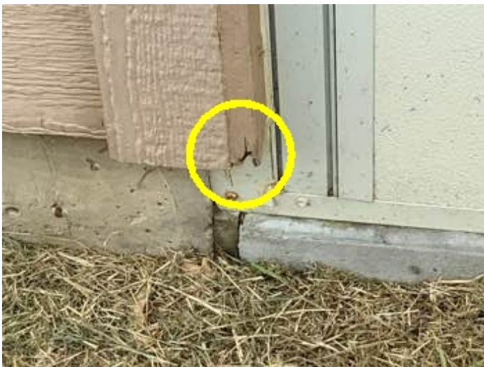
Damaged trim on the right rear corner of this home.
