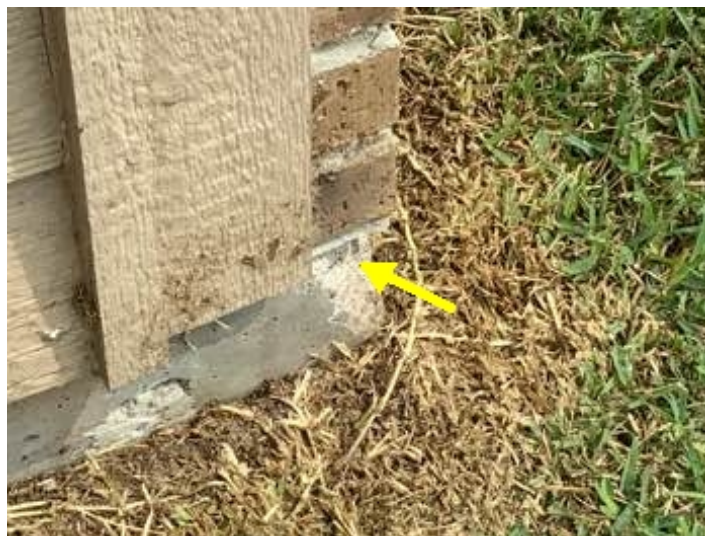
Corner pop on the left front corner of this home.
