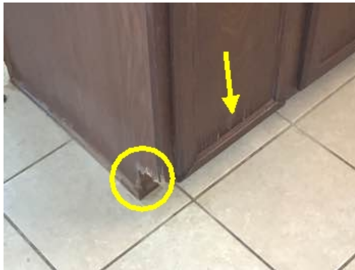
Damaged kitchen cabinets.
