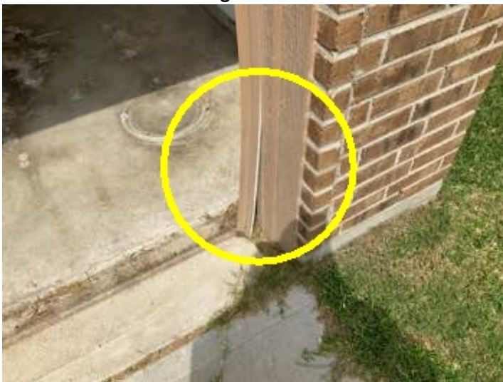
Loose trim on the right side of the garage door.
