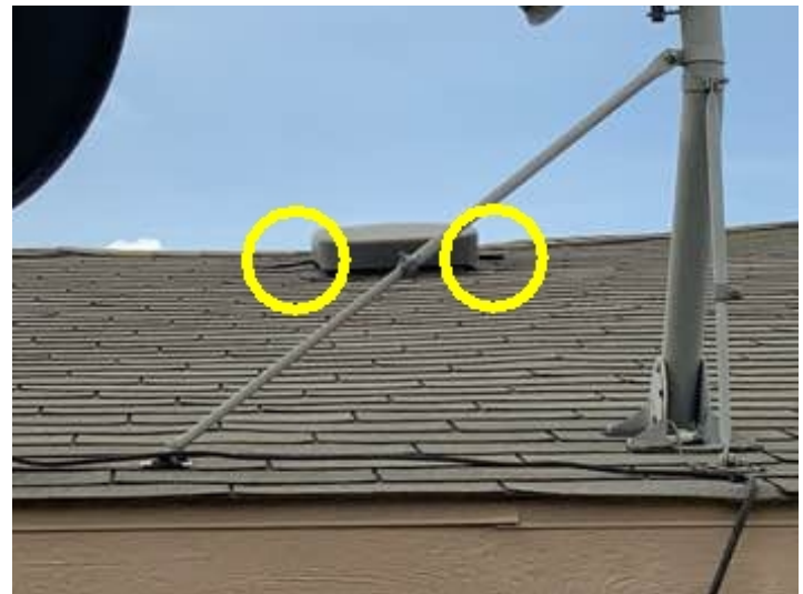
More lifting shingles on the right side of this home.
