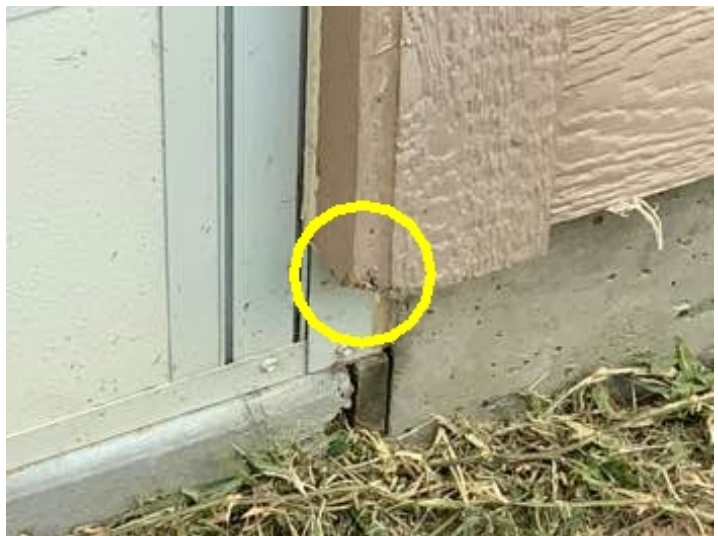
Damaged trim on the left rear corner of this home.
