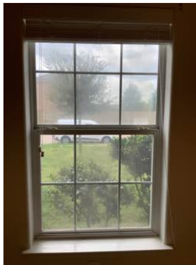
Moisture between the panes of the front guest bedroom window.
