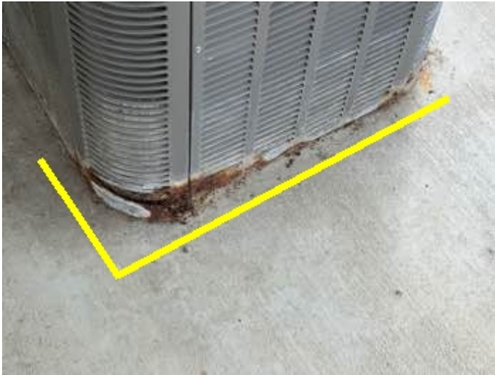
Damaged and deteriorating condensing unit cabinet.
