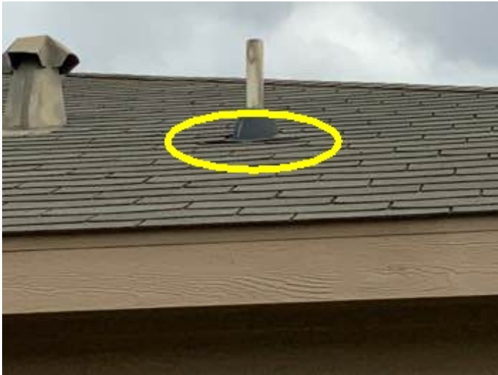
Lifting vent boot flashing on the left side of this home.
