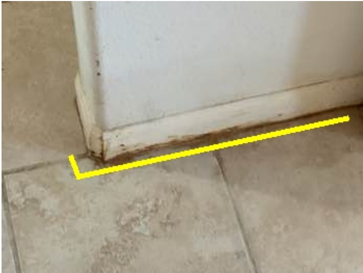
Moisture damage on the baseboards outside the left front guest bedroom.
