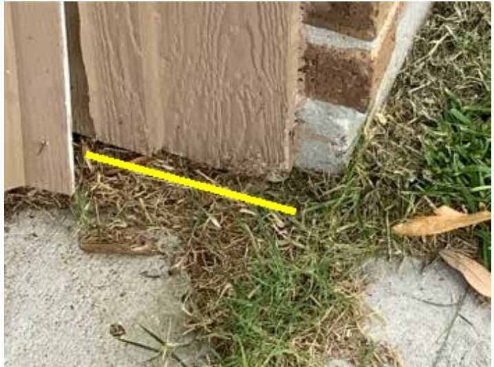
Damaged and deteriorating casing at the garage door.
