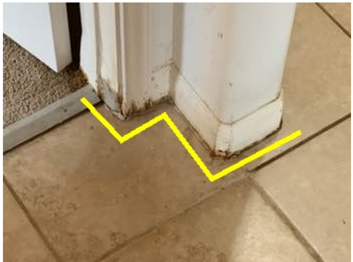
Moisture damage on the baseboards outside the left rear guest bedroom.
