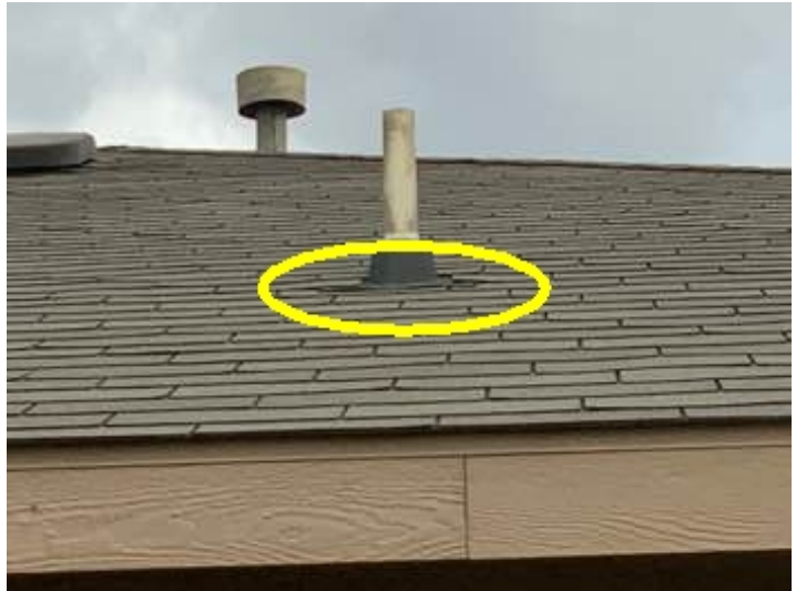
Another lifting vent boot flashing on the left side of this home.
