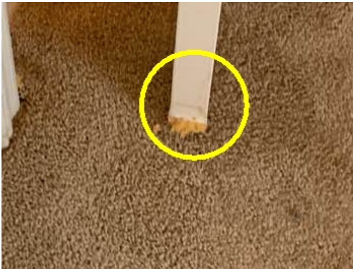
Moisture damaged front guest bedroom door.
