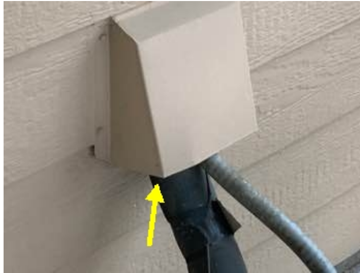
Gap around the condensing unit penetrations on the rear of this home.
