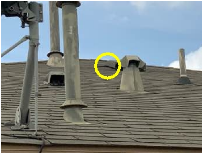
Lifting shingle on the right side of this home.
