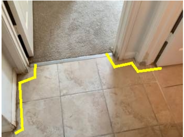
Moisture damaged trim at the front guest bedroom and bathroom doors.
