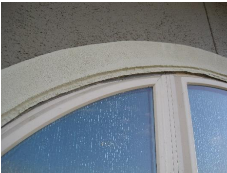
Windows not properly flashed in multiple locations.
