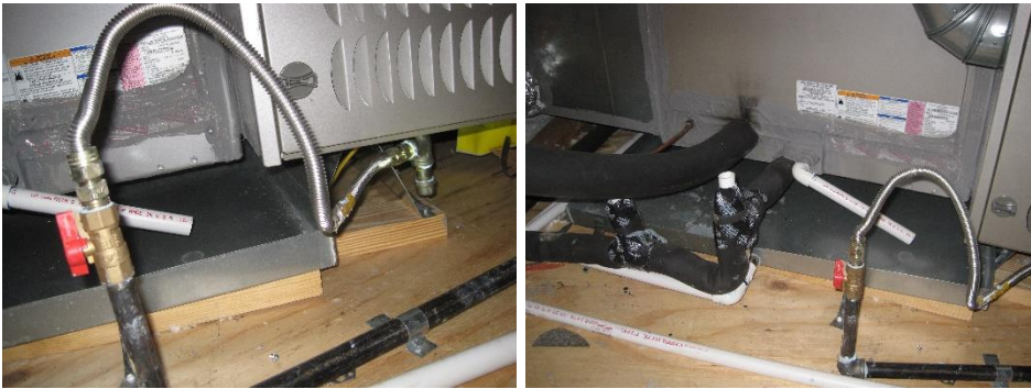
Burner nozzles are dirty.
