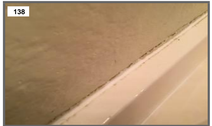
Master bathroom, splashguard to left of sink is loose.
