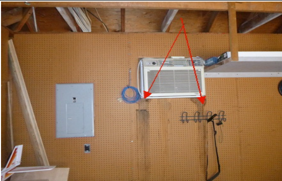
*Leaky portable AC / water damaged peg board
