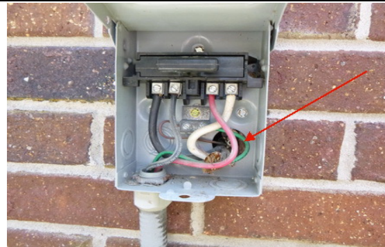
*Missing conduit and knockout insulator
