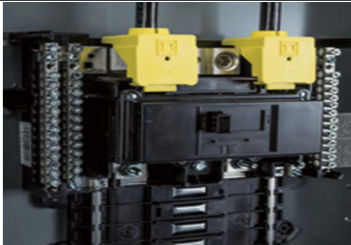
*Service entrance barriers
