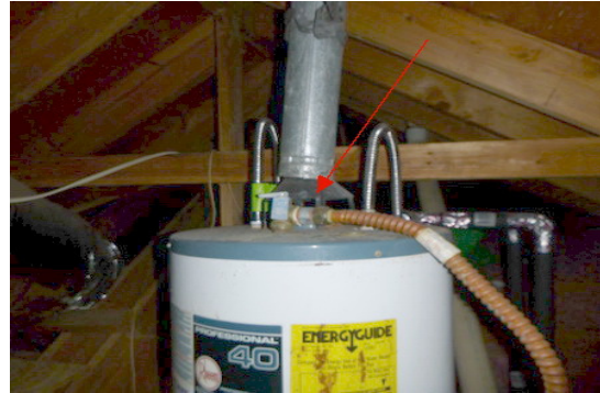
*Corrosion at water line fitting(s)
