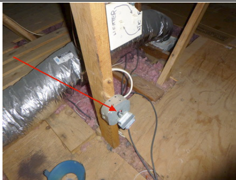
*Secure loose transformer
