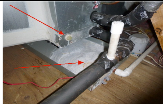
*Install drain at secondary and rust in emergency pan
