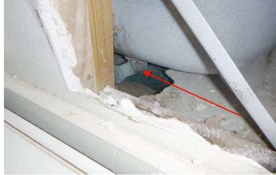
*Hall bath tub drain leak
