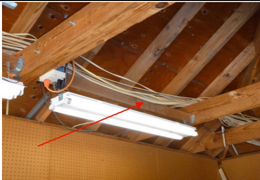
*Support wiring at the ceiling
