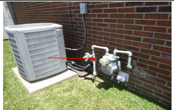
*Condenser / gas meter – too close
