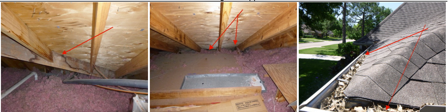
*Water stains at the underside of the roof deck
