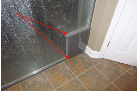
*Water leak at shower surround
