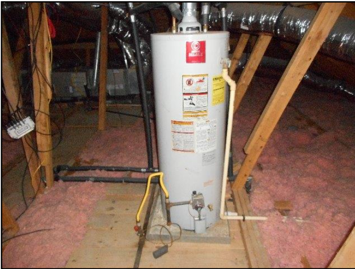
General view of water heater.
