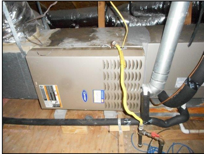
General view of heating system.
