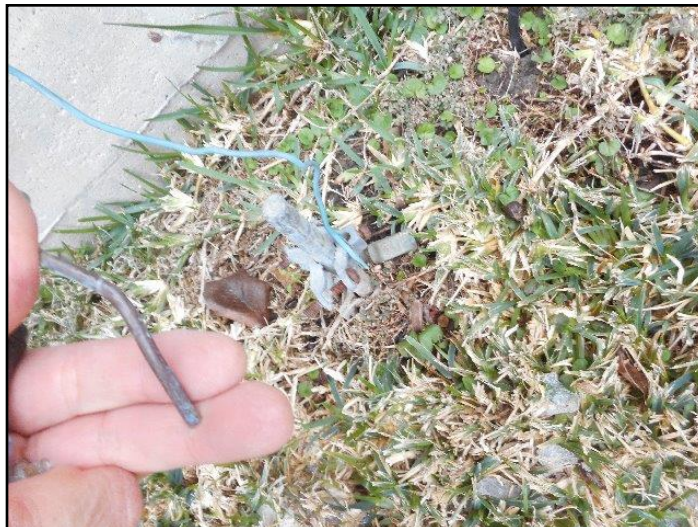
Ground wire is not properly secured to...
