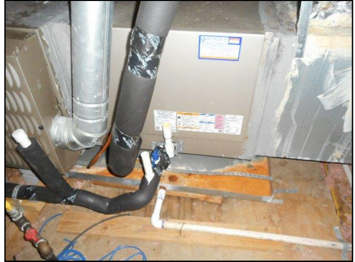
General view of air conditioning equipment
