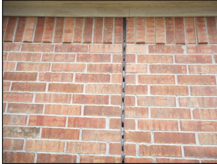
Sealant in the expansion joints has...
