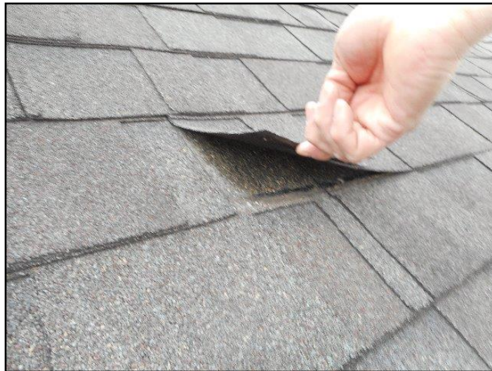
Adhesive strips not fully bonded Note:...
