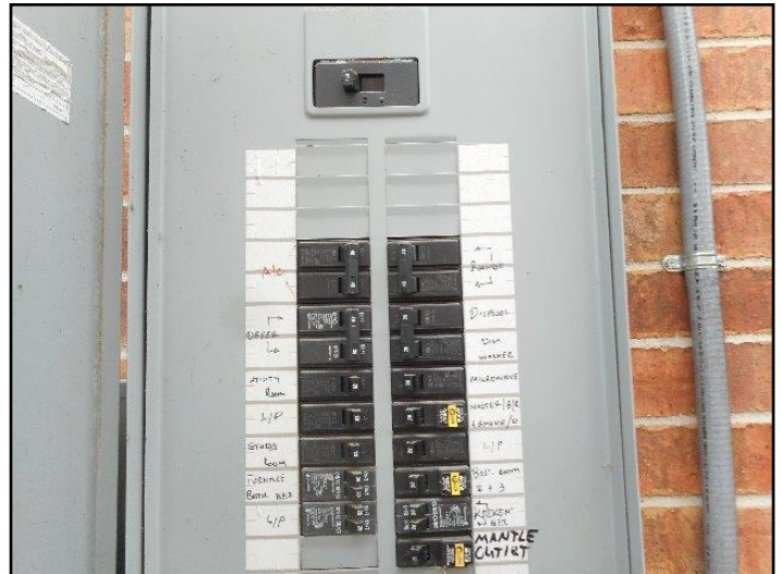
General view of electrical panel(s).
