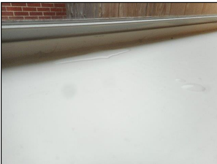
Note: Water stains observed on the window...
