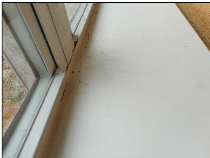
Note: Water stains observed on the window...
