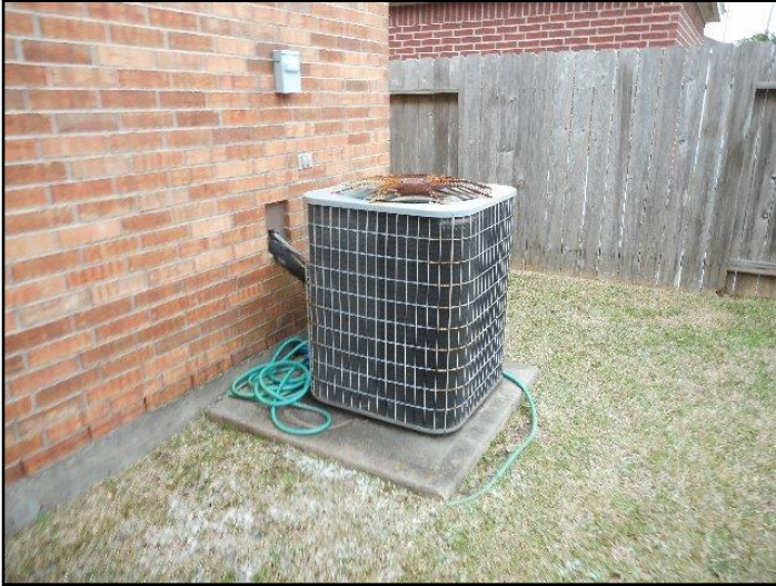
General view of air conditioning equipment
