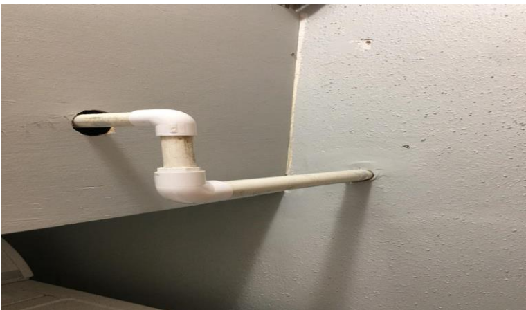
HOT WATER DRAINPIPE
