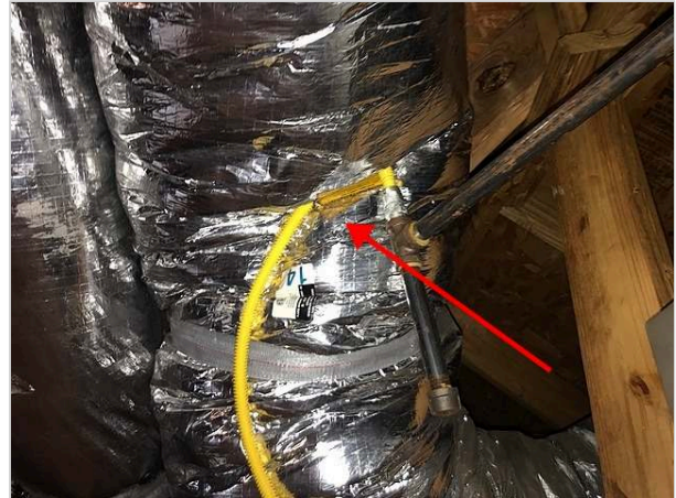
In contact with the gas line
