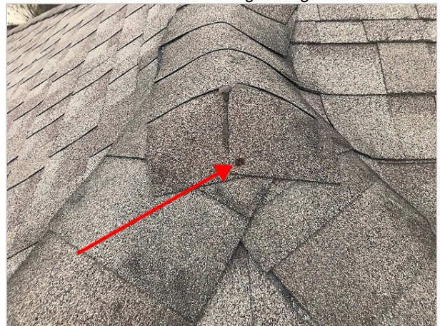
Nail not caulked/showing rust corrosion
