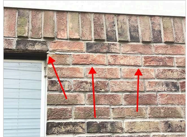
Crack in the brick/rusted header/lintel (right exterior wall)
