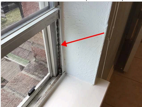
Broken/defective balance (hall bathroom)
