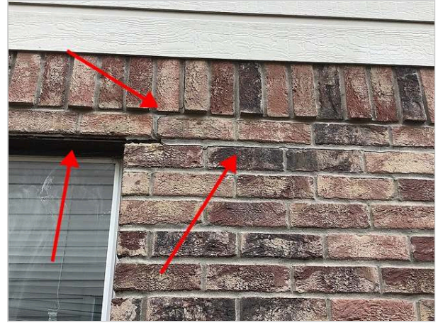
Cracks in the brick/rusted header/lintel (left exterior wall)
