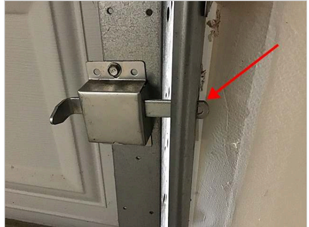
Door lock not disabled
