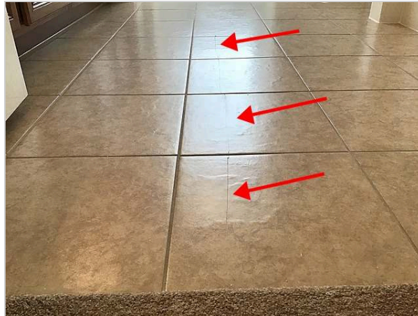
Cracked/damaged floor tiles (master bathroom)
