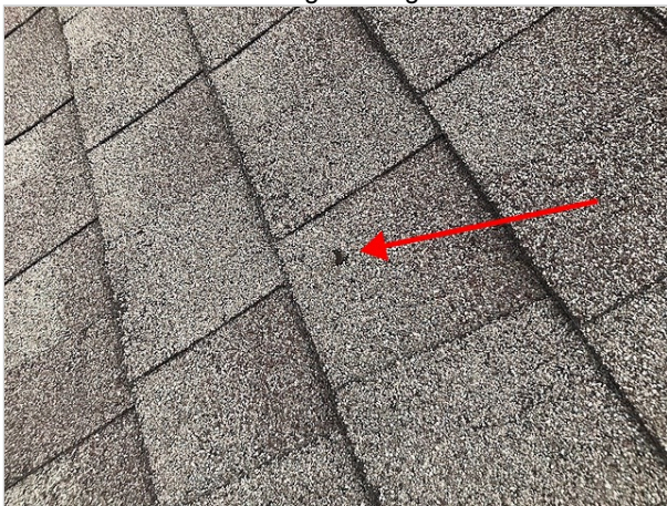
Nail backed out through shingle
