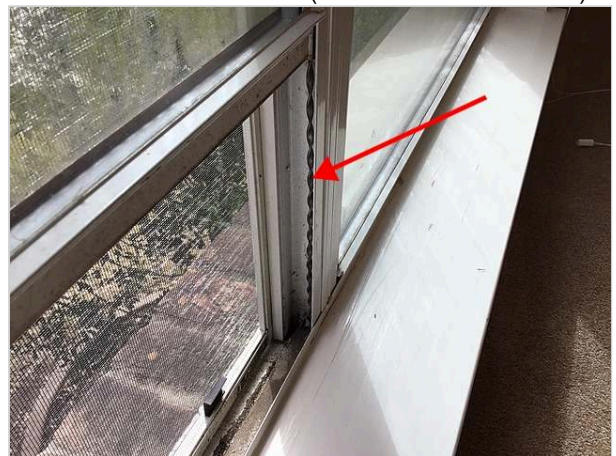
Broken/defective balance (front bedroom)
