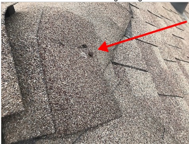
Nails not caulked/showing rust corrosion
