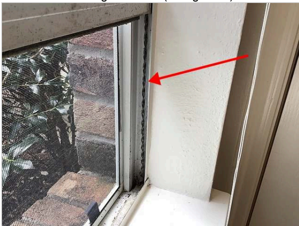
Broken/defective balance (half bathroom)
