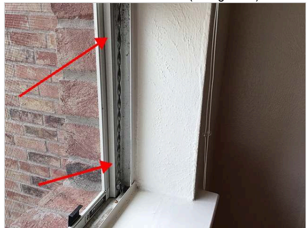
Broken/defective balance (second floor hall window)
