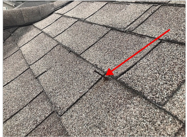
Nail driven through shingle
