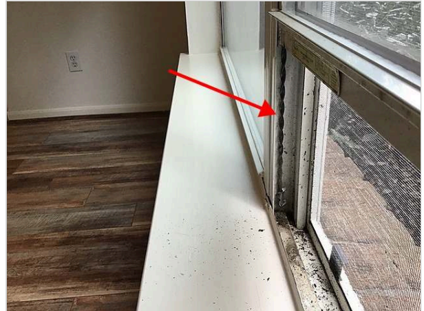
Broken/defective balance (dining room)
