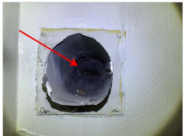
Needed to be cleaned
