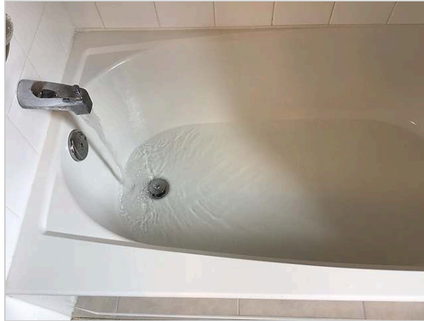
Slow to drain (hall bathtub)
