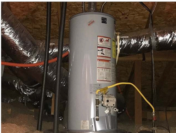
Unit in attic
