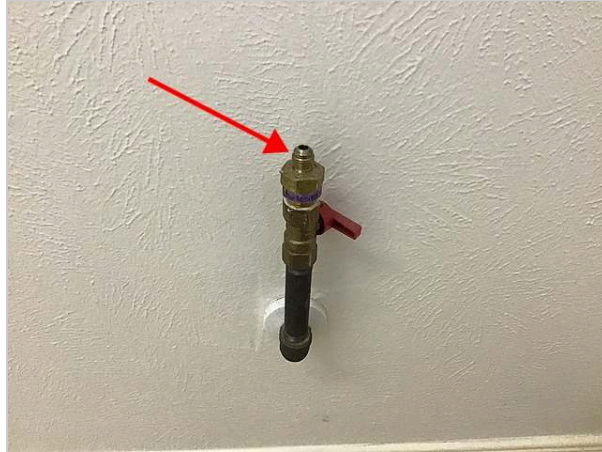
Not properly capped (utility room)
