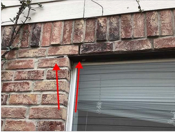
Crack in the brick/rusted header/lintel (left exterior wall)
