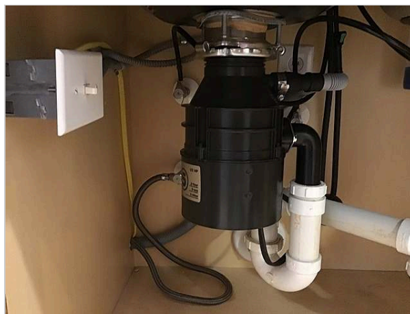
Functioning as intended
