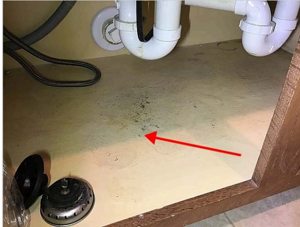
Signs of previous leaks (kitchen)
