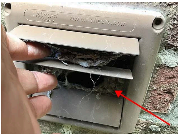
Needed to be cleaned
