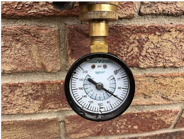
Static water pressure (60-70 psi)
