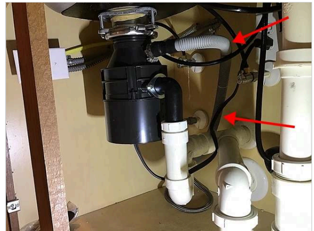
Not properly looped
