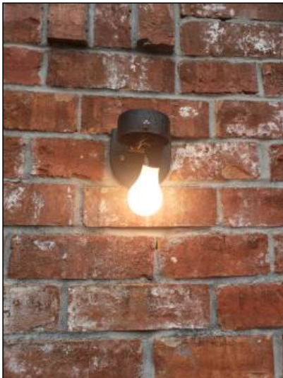
-Light fixture globe is missing or damaged. Mainly at - left exterior
