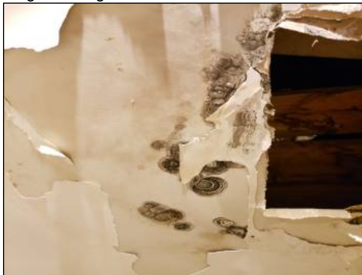
-Mold like stains are present, recommend remediation or cleanup as needed. Unable to determine condition of the underlying materials. Mainly at - garage ceiling
