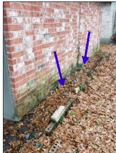
-The soil and or rock level around the home is higher than recommended or in contact with the siding materials. Recommend lowering the soil line to help prevent water penetration and/or damage to the structure. Mainly at - front
