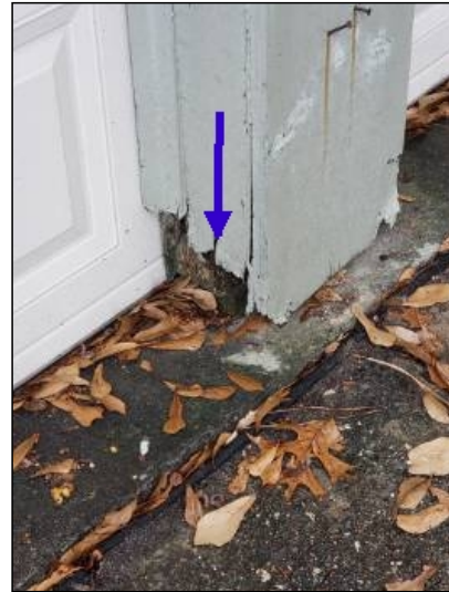
-Deterioration was noted at the trim, recommend replacing all deteriorated trim. Unable to determine the condition of the underlying materials. Mainly at - garage
