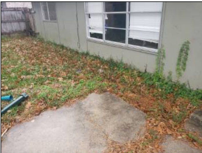
-The soil and or rock level around the home is higher than recommended or in contact with the siding materials. Recommend lowering the soil line to help prevent water penetration and/or damage to the structure. Mainly at - rear
