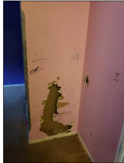
-There is damage to the drywall, recommend repairs as needed. Mainly at - throughout
