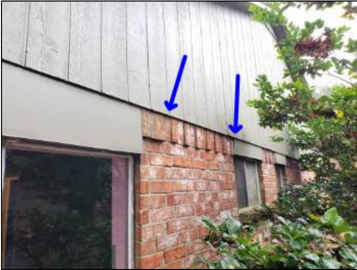
-Deterioration was noted at the siding, recommend replacing all deteriorated siding to help prevent further deterioration and water penetration. Unable to determine the condition of the underlying materials. Mainly at - right
