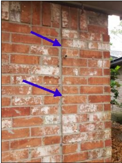
-Settlement cracks were noted in the brickwork. Mainly at - front right
