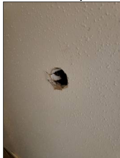
-There is damage to the drywall, recommend repairs as needed. Mainly at - throughout
