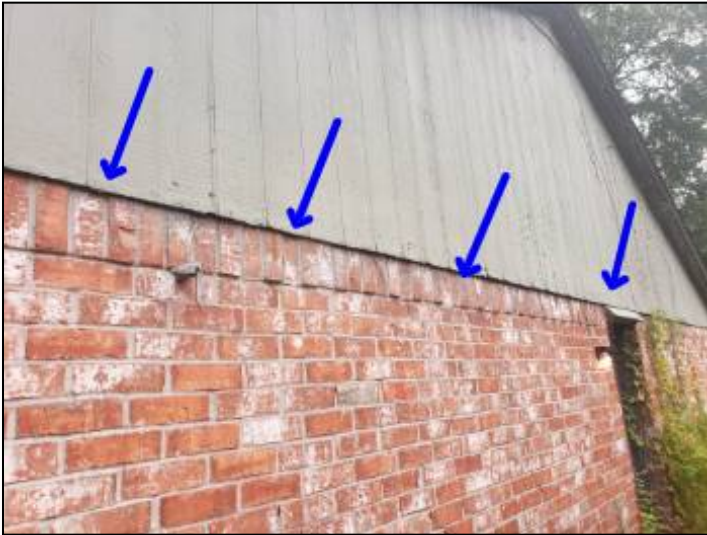
-Deterioration was noted at the siding, recommend replacing all deteriorated siding to help prevent further deterioration and water penetration. Unable to determine the condition of the underlying materials. Mainly at - left
