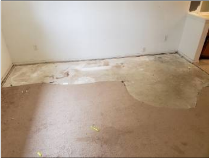
Carpet is damaged. Mainly at- master bedroom
