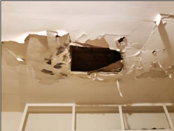
-There is at least one hole in the ceiling in the garage. All holes in the garage ceilings or wall against living areas should be patched to help keep the recommended fire barrier between the home and garage.
