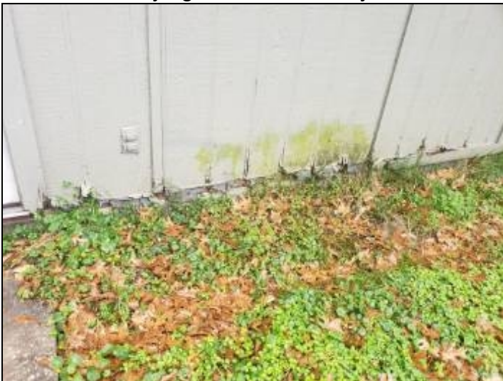
-Deterioration was noted at the siding, recommend replacing all deteriorated siding to help prevent further deterioration and water penetration. Unable to determine the condition of the underlying materials. Mainly at - rear
