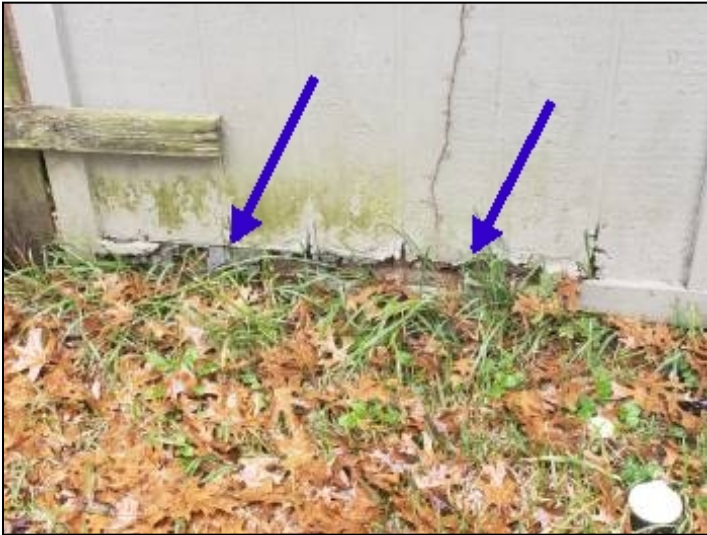
-Deterioration was noted at the siding, recommend replacing all deteriorated siding to help prevent further deterioration and water penetration. Unable to determine the condition of the underlying materials. Mainly at - rear
