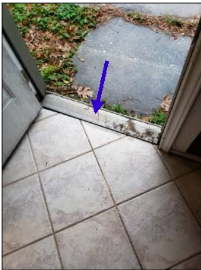
Threshold is sloped into the house. Threshold should slope toward the outside to shed water. Mainly at- back door
