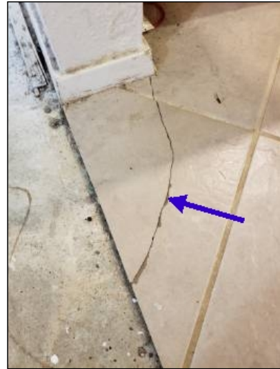
-Cracks were noted in the tile. Mainly at - master bath
