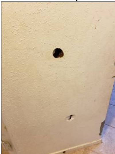
-There is damage to the drywall, recommend repairs as needed. Mainly at - throughout
