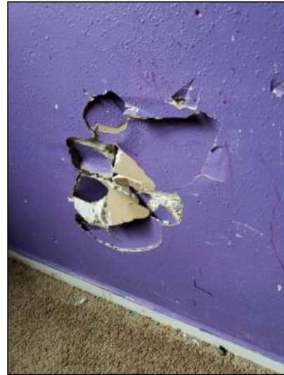
-There is damage to the drywall, recommend repairs as needed. Mainly at - throughout
