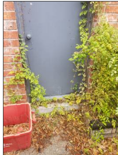
-Deterioration was noted mainly along the door jamb, recommend repair or replacement to help prevent water penetration. Unable to determine the condition of the underlying materials. Mainly at - garage exterior door
