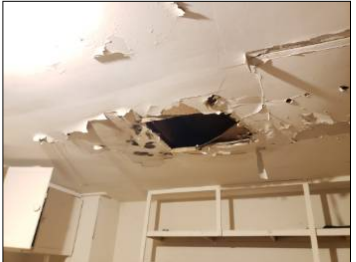
-Paint is peeling in the garage ceilings. This is a common occurrence due to high moisture of unconditioned garage space, recommend repainting to help prevent further deterioration.
