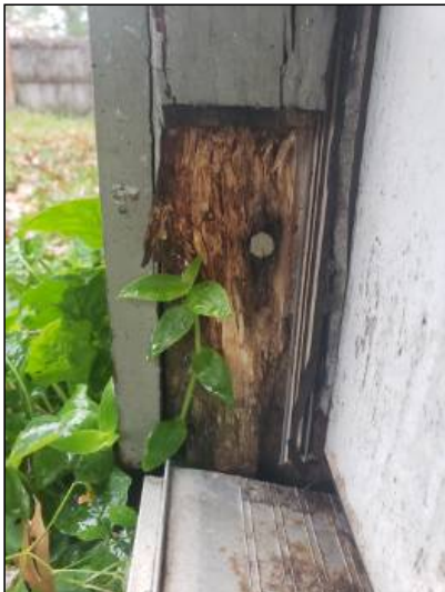
-Deterioration was noted mainly along the door jamb, recommend repair or replacement to help prevent water penetration. Unable to determine the condition of the underlying materials. Mainly at - back door
