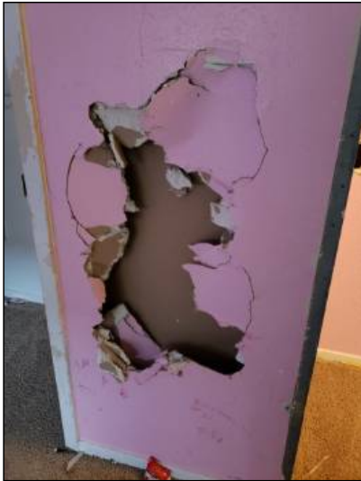
-There is damage to the drywall, recommend repairs as needed. Mainly at - throughout
