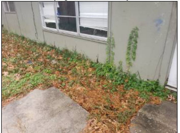
-Deterioration was noted at the siding, recommend replacing all deteriorated siding to help prevent further deterioration and water penetration. Unable to determine the condition of the underlying materials. Mainly at - rear
