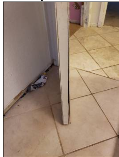
-The skin on the door is loose, recommend re-securing. Mainly at - hall bath
