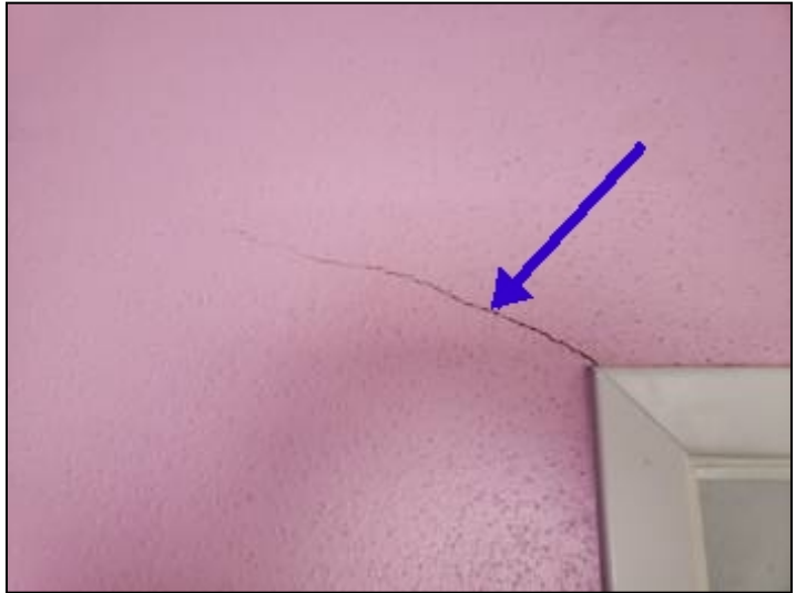
-Settlement cracks were noted in the drywall. Mainly at - front right bedroom
