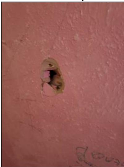
-There is damage to the drywall, recommend repairs as needed. Mainly at - throughout
