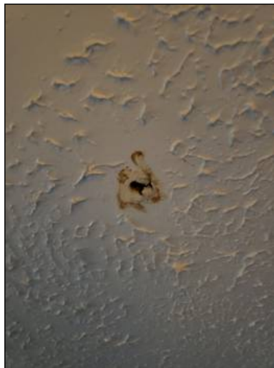
Hole in ceiling. Mainly at- front left bedroom
