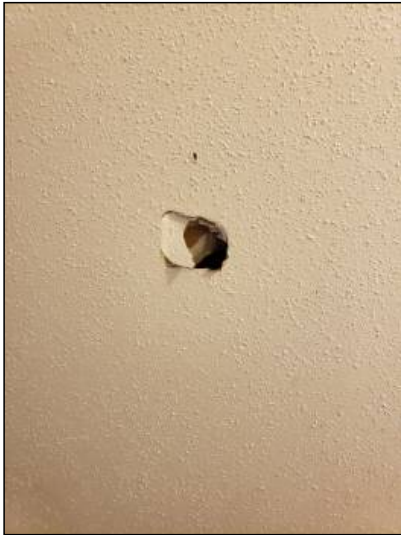
-There is damage to the drywall, recommend repairs as needed. Mainly at - throughout
