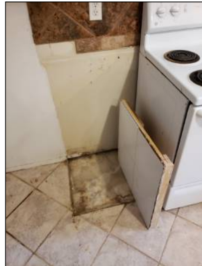
-Although cabinets are not inspected it was noted that cabinets are damaged throughout.
