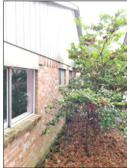
-Recommend trimming vegetation so that it is not in contact with the house. Vegetation in contact with the structure can hold moisture against the structure and promote damage to building materials and conducive conditions for wood destroying insects.
