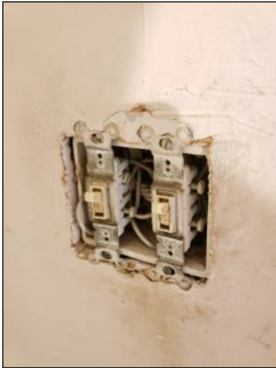
-Switch plate is broken or missing, recommend replacing covers to help prevent electrical shock. Mainly at - garage
