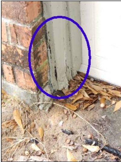
-Deterioration was noted at the trim, recommend replacing all deteriorated trim. Unable to determine the condition of the underlying materials. Mainly at - garage
