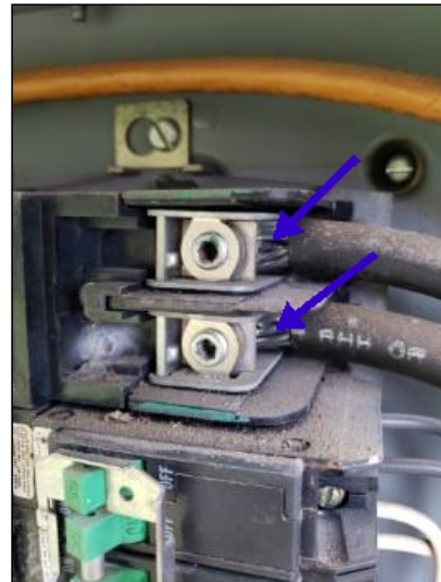
-There is no antioxidant on main aluminum feeds to the panel box. This should be used to help prevent overheating.
