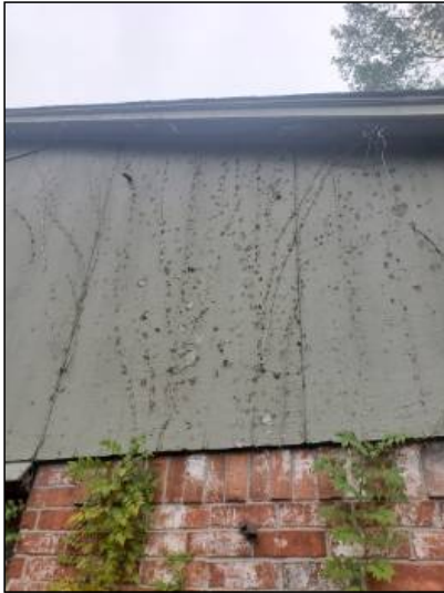
-There is some damage to the exterior siding, recommend repair or replacement to help prevent water penetration. Unable to determine the condition of the underlying materials. Mainly at - left
