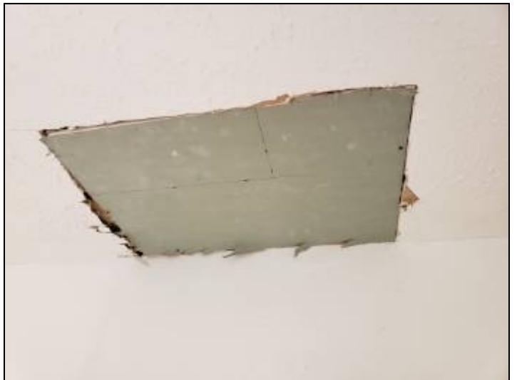
-Previous repairs were noted in the ceiling. Mainly at - breakfast nook
