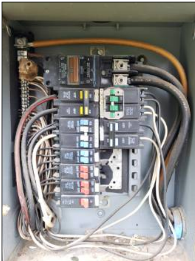
Overview of main electrical panel
