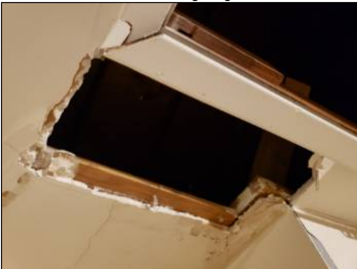
-There is at least one hole in the ceiling in the garage. All holes in the garage ceilings or wall against living areas should be patched to help keep the recommended fire barrier between the home and garage.
