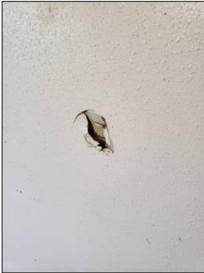
-There is damage to the drywall, recommend repairs as needed. Mainly at - throughout
