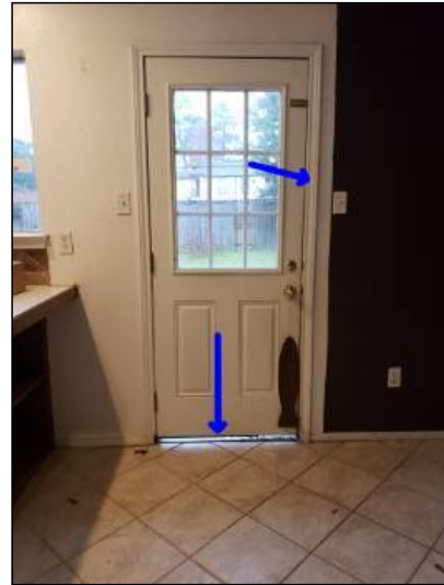
-There is visible light noted around the door. Mainly at - back door
