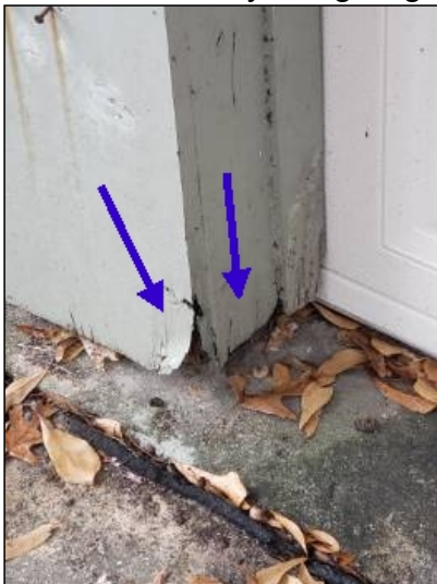
-Deterioration was noted at the trim, recommend replacing all deteriorated trim. Unable to determine the condition of the underlying materials. Mainly at - garage
