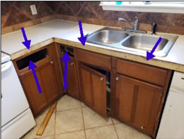
-Although cabinets are not inspected it was noted that cabinets are damaged throughout.
