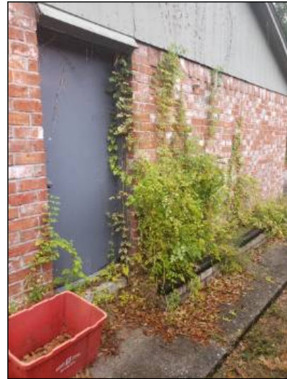
-Recommend trimming vegetation so that it is not in contact with the house. Vegetation in contact with the structure can hold moisture against the structure and promote damage to building materials and conducive conditions for wood destroying insects.
