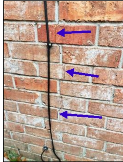
-Settlement cracks were noted in the brickwork. Mainly at - right
