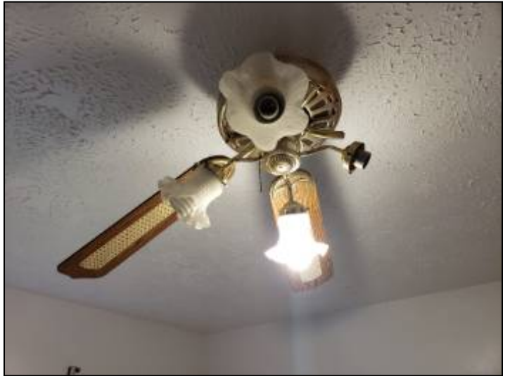
Light fixture is damaged. Mainly at- master bedroom
