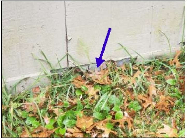
-Deterioration was noted at the siding, recommend replacing all deteriorated siding to help prevent further deterioration and water penetration. Unable to determine the condition of the underlying materials. Mainly at - rear
