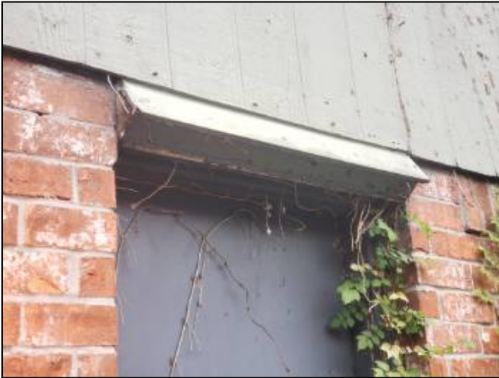
Door header is loose. Mainly at- garage exterior door
