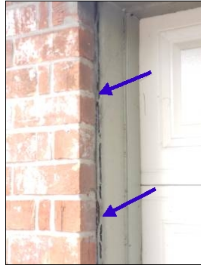
-Recommend sealing between the trim and brickwork to help prevent water penetration. Mainly at - garage
