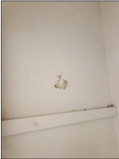
-There is damage to the drywall, recommend repairs as needed. Mainly at - throughout
