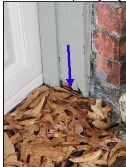
-Deterioration was noted at the trim, recommend replacing all deteriorated trim. Unable to determine the condition of the underlying materials. Mainly at - garage
