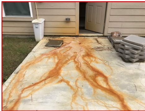
Rust stains from the AC secondary drain
