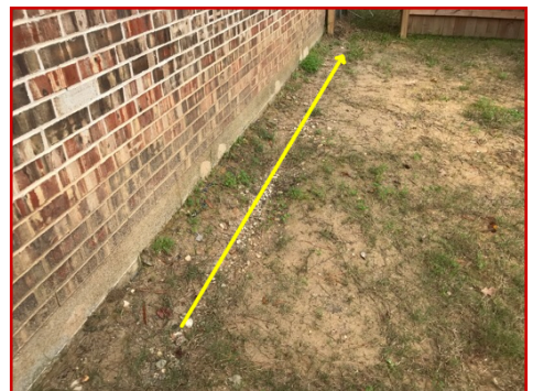
Rain draining from the roof is cutting a trench
