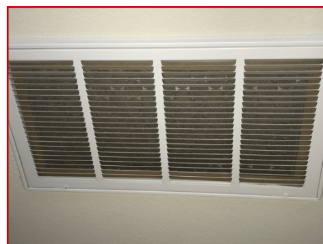
Down stairs return, dirty filter
