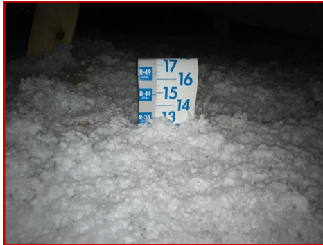
Fiberglass blown insulation
