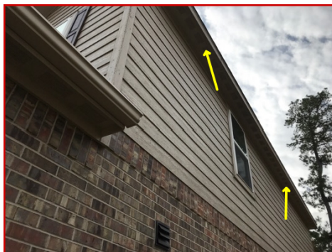
Only partial gutters
