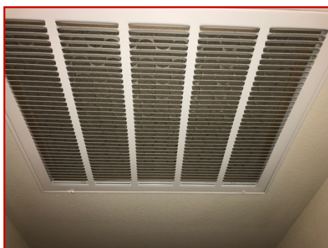
Upstairs return, dirty filter
