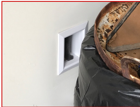
Main water shut off in garage
