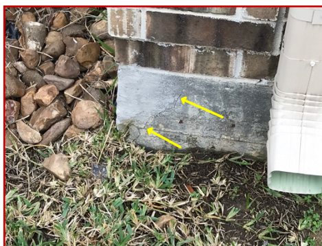
Common corner crack
