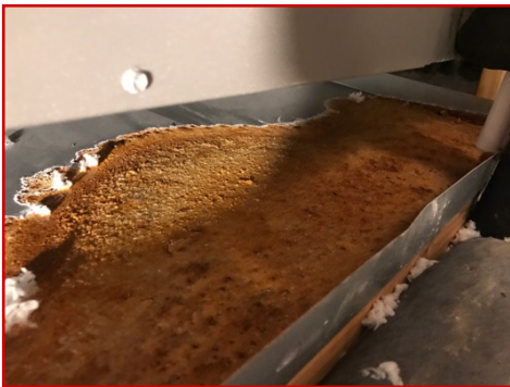
Minor rust in catch pan, no moisture
