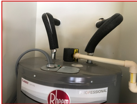
Water and electrical connections ok
