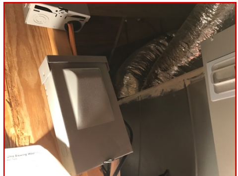
Electric shut off
