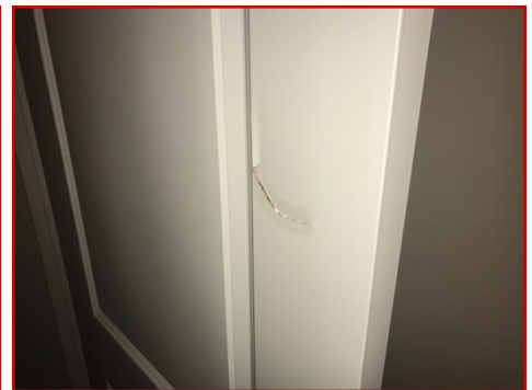
Minor damage to door in upstairs bathroom
