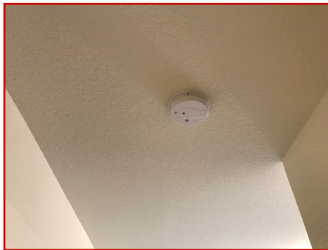
Smoke detector in upstairs bedroom is chirping
