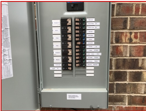
Dead front is clean, all breakers marked, AFCI and GFCI breakers present
