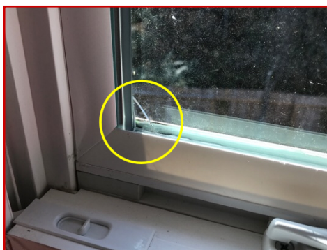
Cracked window pane in upstairs living room
