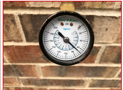
Static pressure approximately 70 psi
