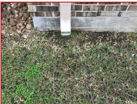
Gutter discharges to foundation
