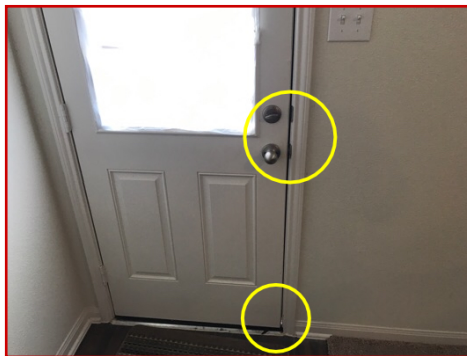
Light visible at rear door and door rattles when closed
