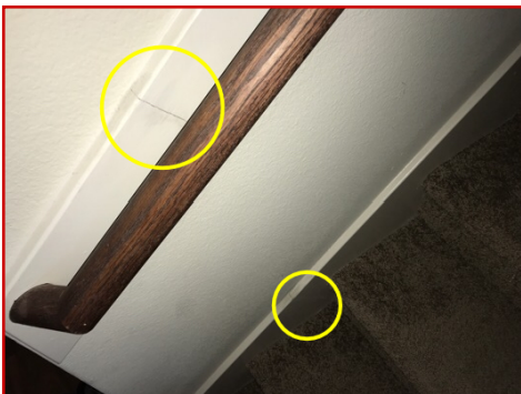
Separation in trim at stairs
