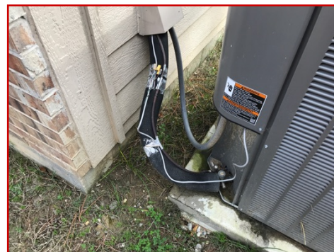
Line insulation is ok
