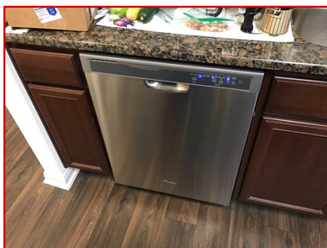
Dishwasher appeared to operate normally at inspection
