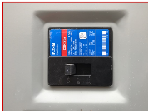
150 amp main breaker
