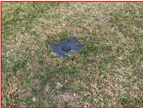
Water meter in front yard
