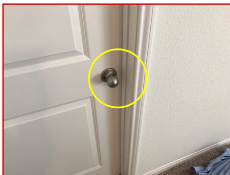
Master bedroom door does not latch
