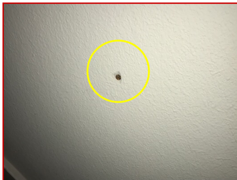
Nail pop in stairway wall
