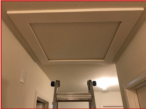
Sealed insulated attic hatch in upstairs hallway
