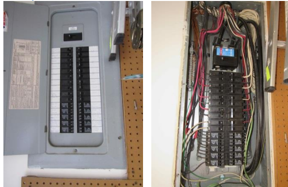
Main panel box.
