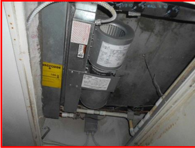
Inoperable A/C Unit
