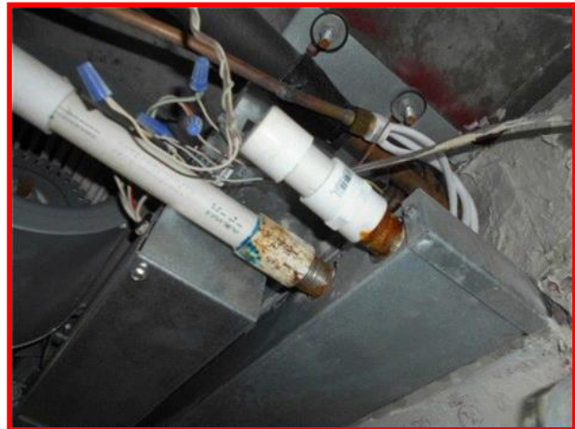
Inoperable A/C Unit
