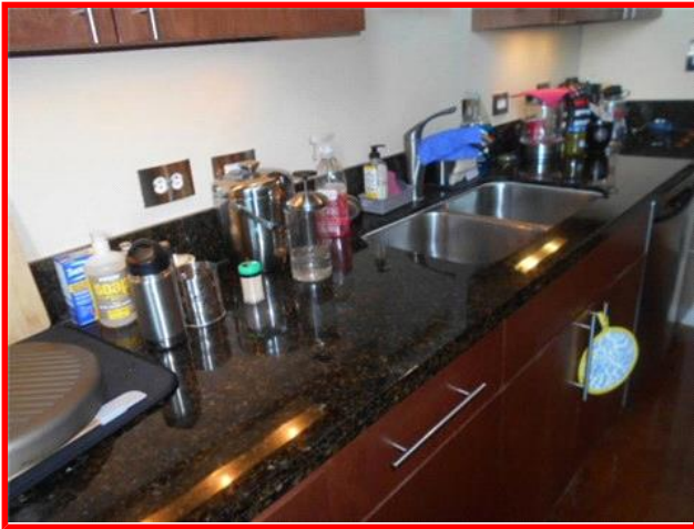
Missing GFI Protection at Kitchen Counter Outlets
