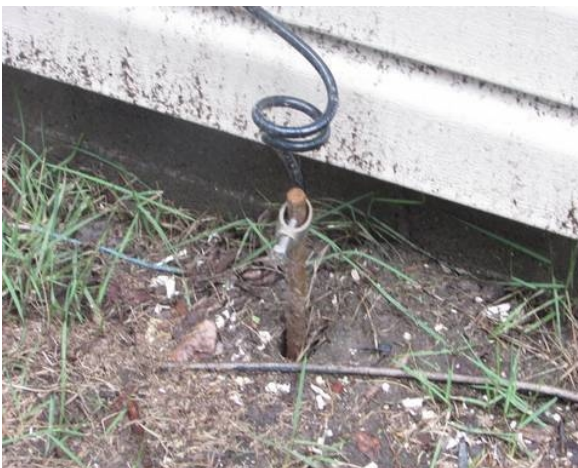
Grounding Rod connection
