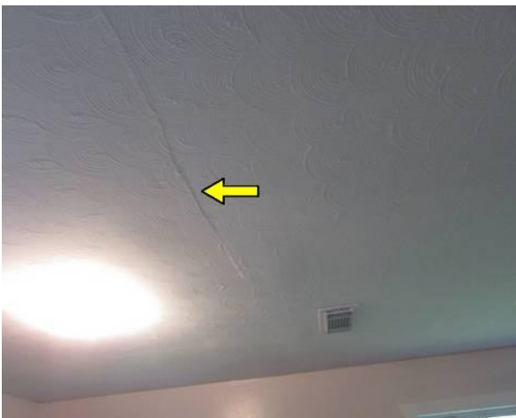
Crack - living room
