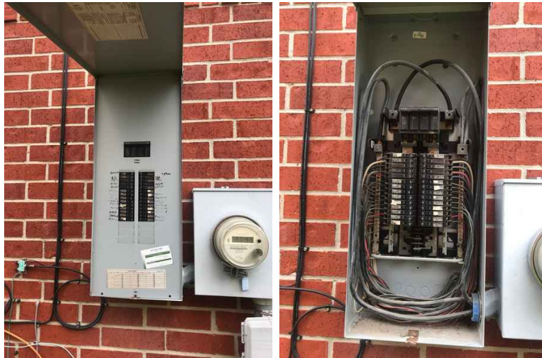
General Infrared Photos of Distribution Panel(s):
