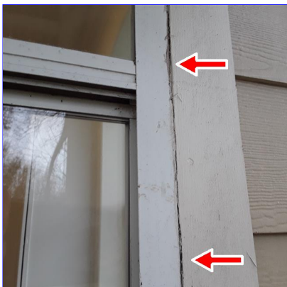
H. Item 3(Picture) Window at back upper balcony by kitchen
