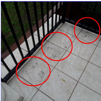
F. Item 1(Picture) Chipped tile at upper first level balcony
