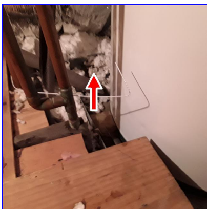
C. Item 1(Picture) Water heater pan needs to be cleaned out.
