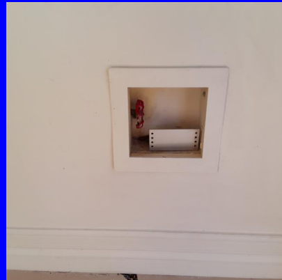
Main water shut-off valve located at garage
