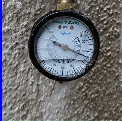
Water pressure to home is 50 PSI
