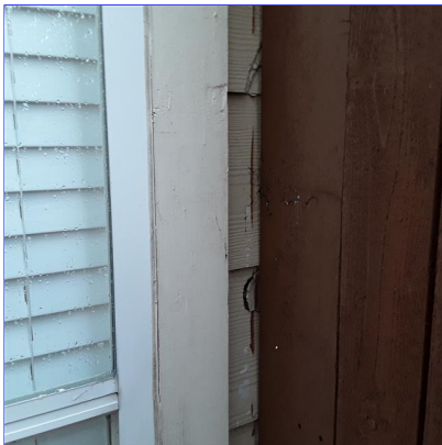
E. Item 9(Picture) Damaged siding at left side, lower level
