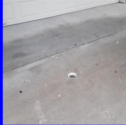
Main sewer clean out located at front drive
