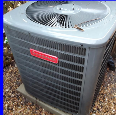
Goodman HVAC unit 2 - manufactured in 2011
