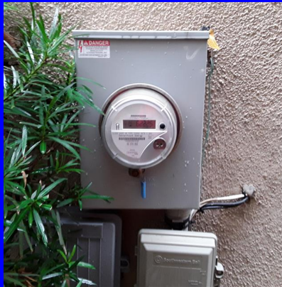
Electrical meter with underground service at right entry
