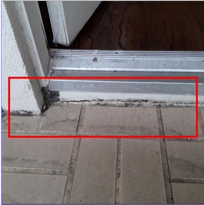
K. Item 2(Picture) First level deck, front living area needs fresh caulk at the exterior to wall, to keep moisture out of the wall system
