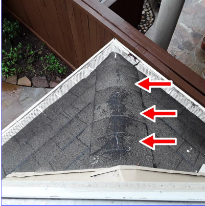
C. Item 2(Picture) Heavily damaged hip ridge shingles at rear lower level.
