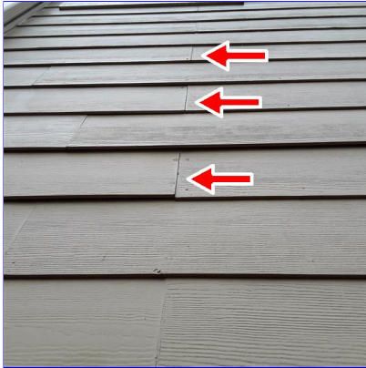
E. Item 7(Picture) Left side siding and areas around home need the caulk at joints. to prevent moisture from penetrating wall system.
