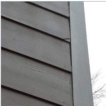
E. Item 11(Picture) Damaged siding at left side
