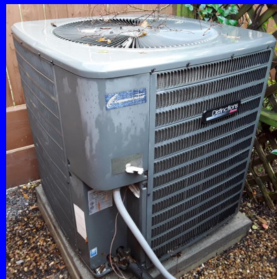
Armana HVAC unit 1 - manufactured in 2008
