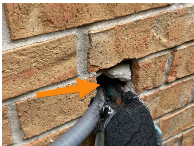
AC unit area
