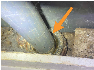
Master bathroom plumbing access
