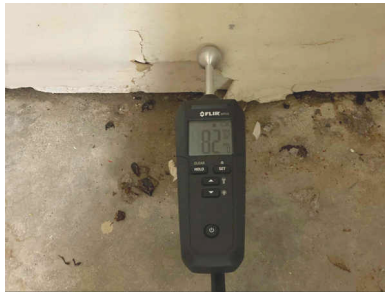
Utilities area in garage
