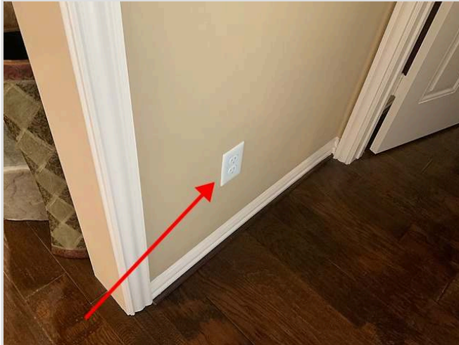
Loose (master bedroom hallway)
