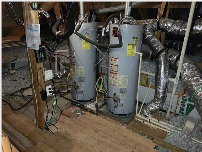
Units in the attic
