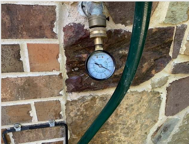
Static water pressure (50-60 psi)
