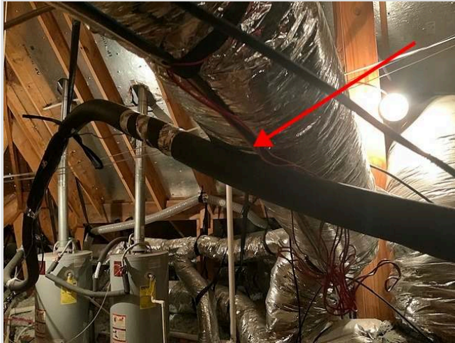
Ducts in contact with refrigerant lines
