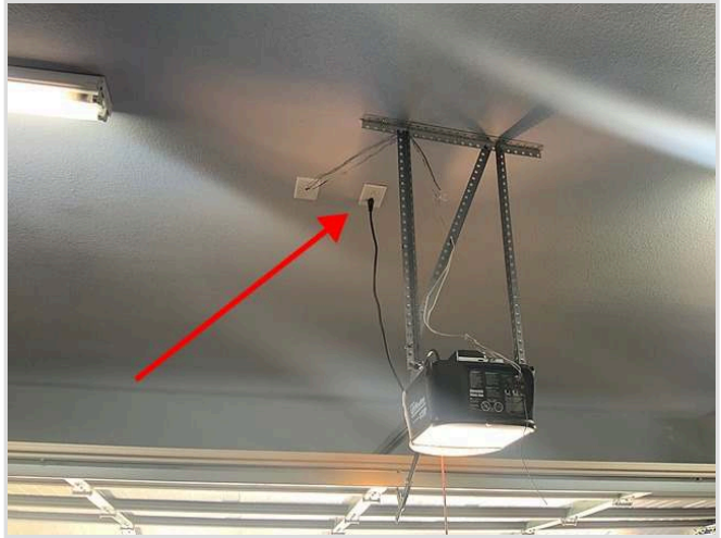
Not on GFCI
