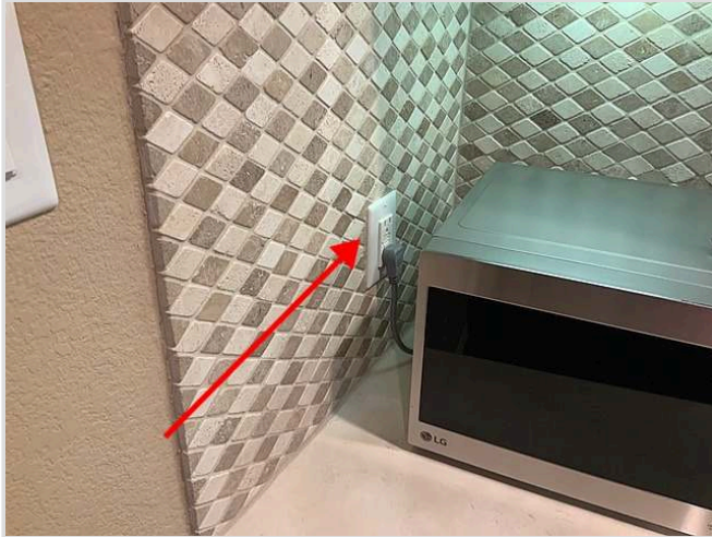
Loose (wet bar on second floor)
