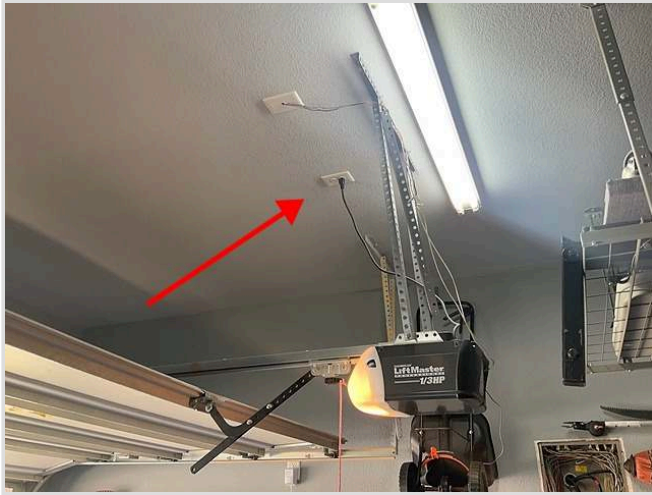
Not on GFCI
