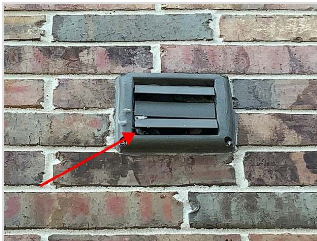
Needed to be cleaned
