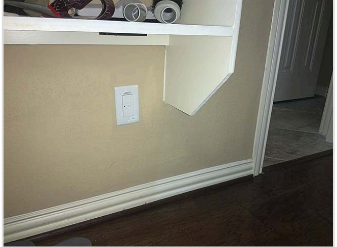
GFCI location (master bath closet)
