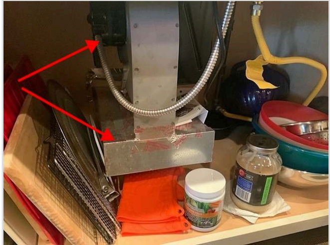
Motor and vent of range exhaust
