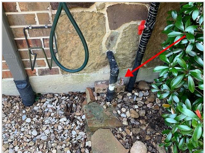
Water meter supply valve
