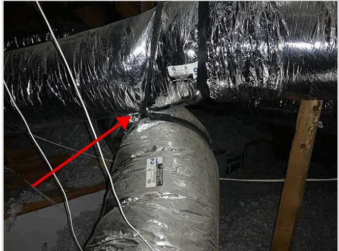
Ducts in contact with other ducts
