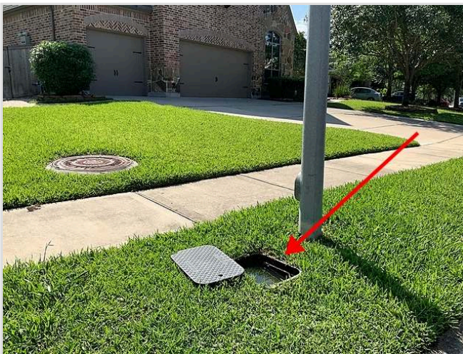
Water meter location
