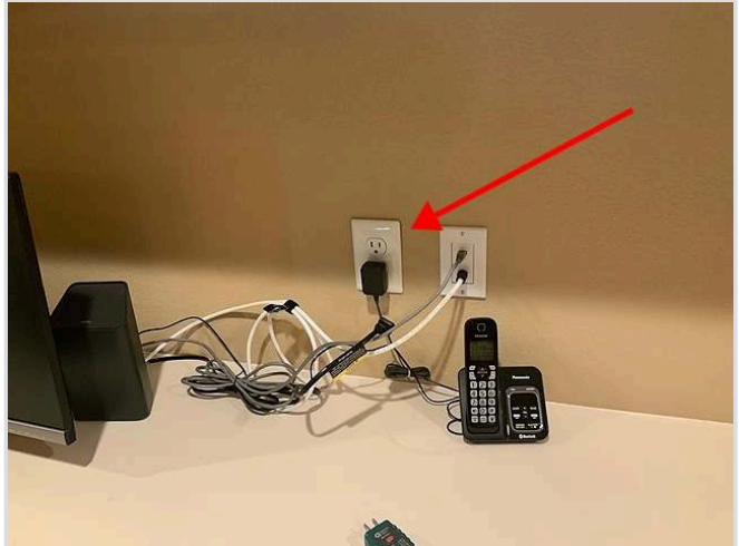
Loose (second floor hall-office area)
