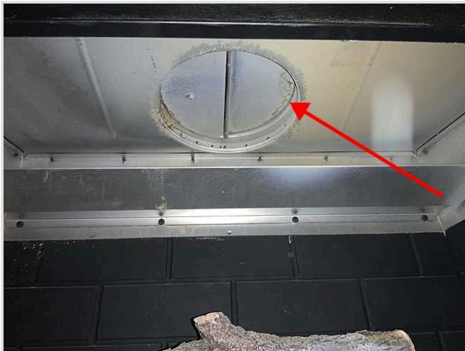
No damper clamp present
