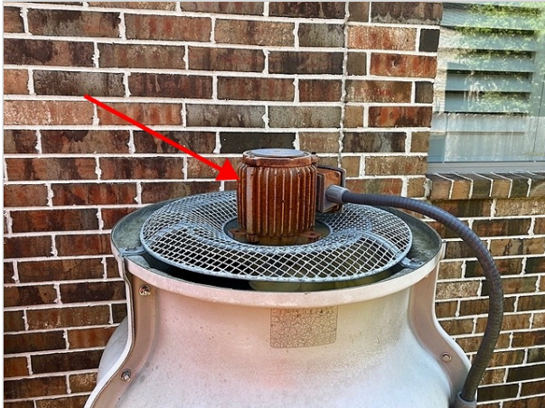
Motor housing rusted
