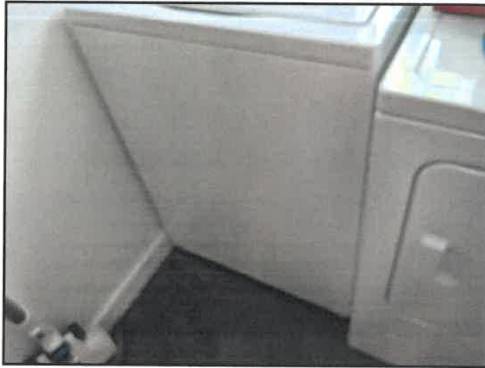
98. Drip pan missing
