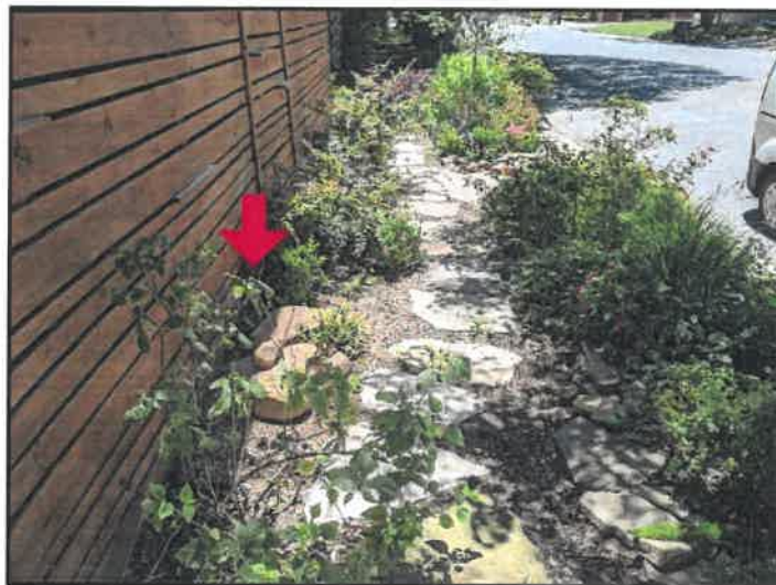
17. Too close to grade
