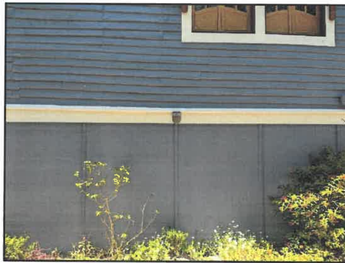
44. Bowed, bulging or leaning
