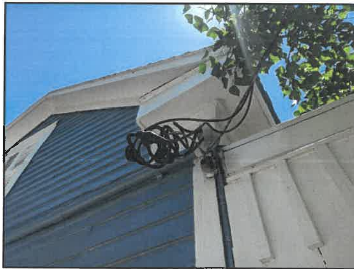
54. Wires too close to roof
