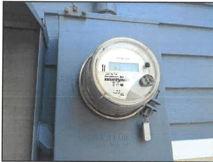
50. Breakers - exterior wall
