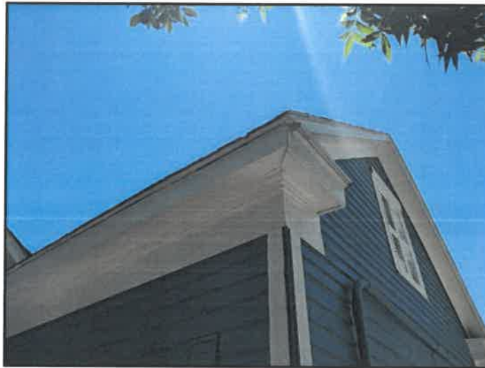
15. Vents - ineffective / missing
