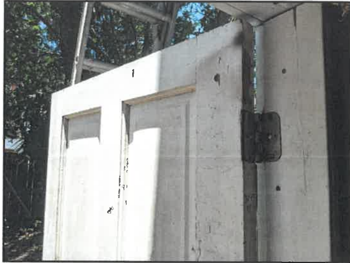
24. Loose or poor fit
