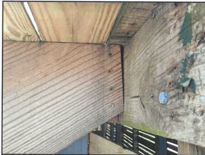
43. Inadequately secured to header
