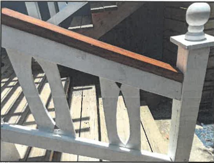
38. Openings between spindles (balusters) too...
