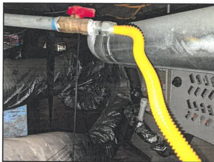
69. No drip leg (sediment trap, dirt pocket)
