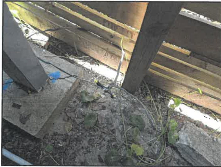
59. Wires too close to grade
