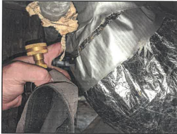
76. Disconnected or leaking
