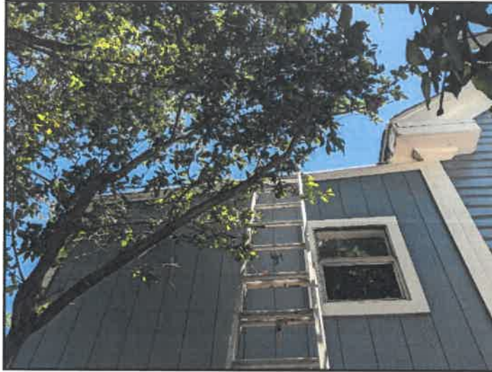
11. Tree branches touching roof
