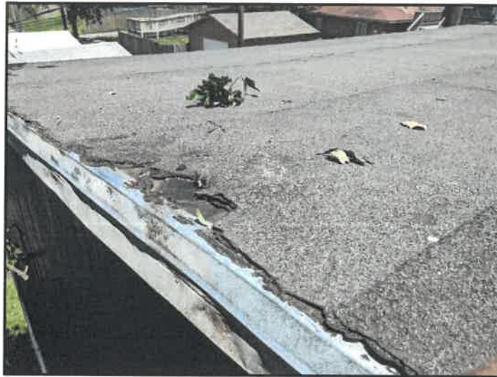
9. Damage, punctures, tears
