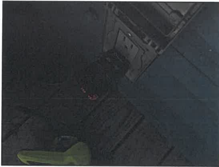
63. No GFCI/GFI (Ground Fault Circuit...
