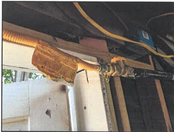
86. No drip leg (sediment trap/dirt pocket)
