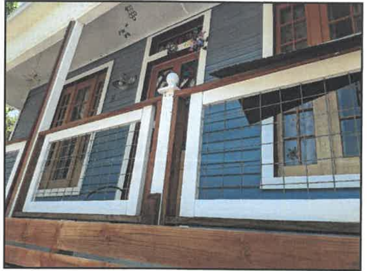
39. Openings between spindles (balusters) too...
