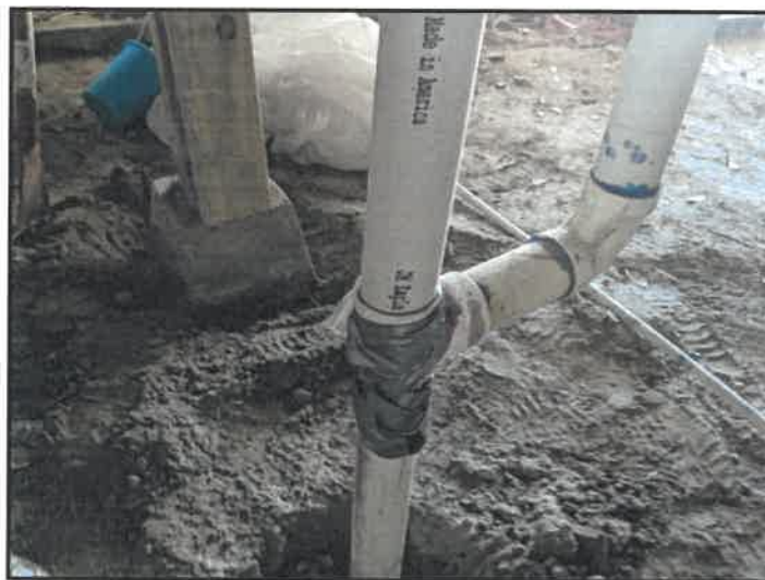
87. Poor manifolding of drain pipe
