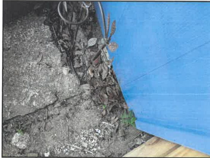
16. Too close to grade
