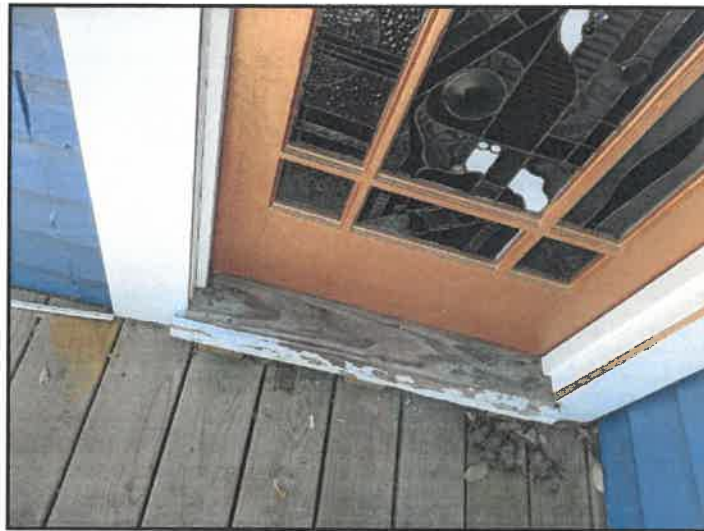
25. Paint or stain needed
