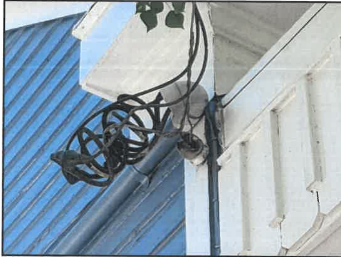
48. Overhead - cable type not determined
