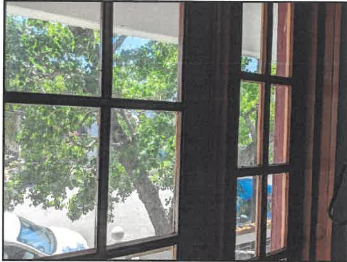
95. Safety glass not installed
