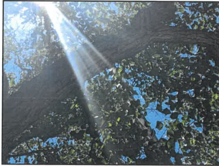
53. Branches / vines interfering with wires
