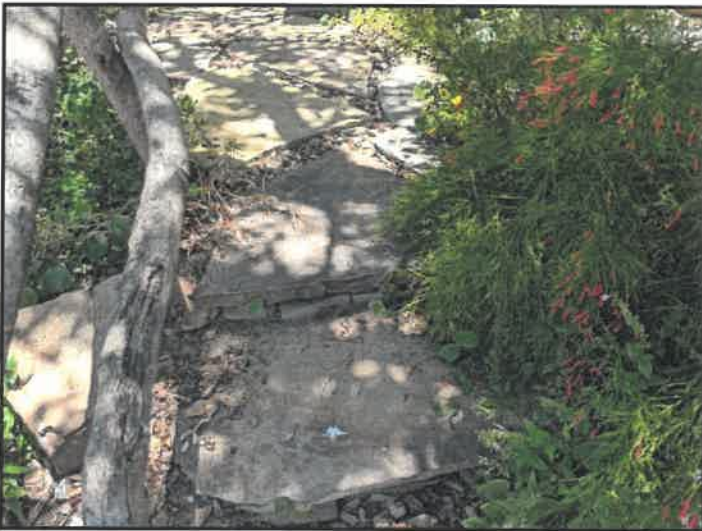
34. Stair rise too big or not uniform
