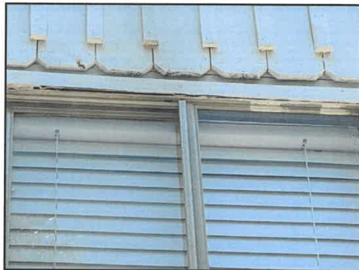
20. Paint and Caulking - deteriorated / missing
