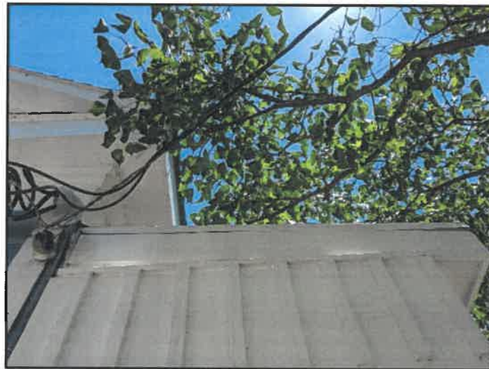
3. Tree branches touching roof
