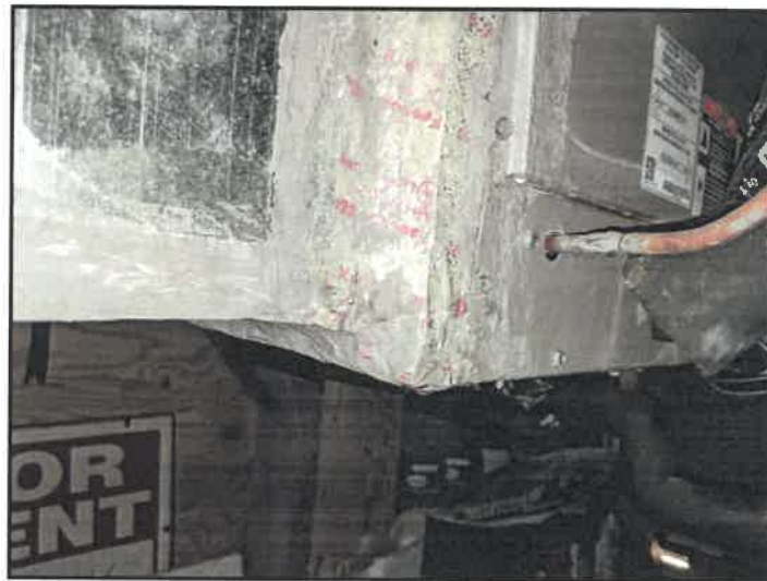
74. Blocked or crimped
