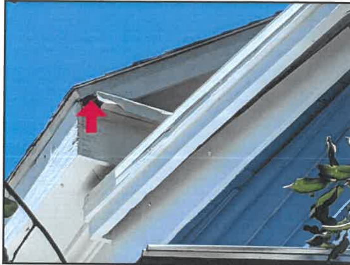
4. Loose, damaged, patched, open seams
