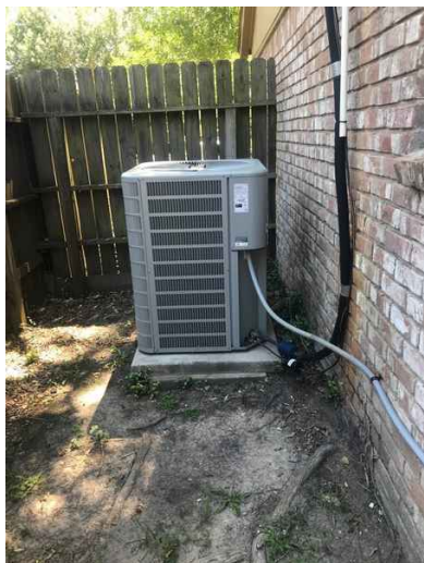
General Photos of HVAC Equipment:
