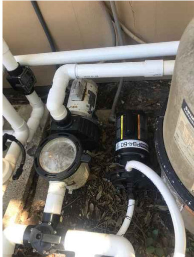
Water Treatment:: Auto-Chlorination
