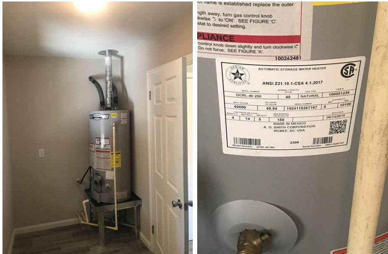
General Infrared Photos of Water Heating Equipment:
