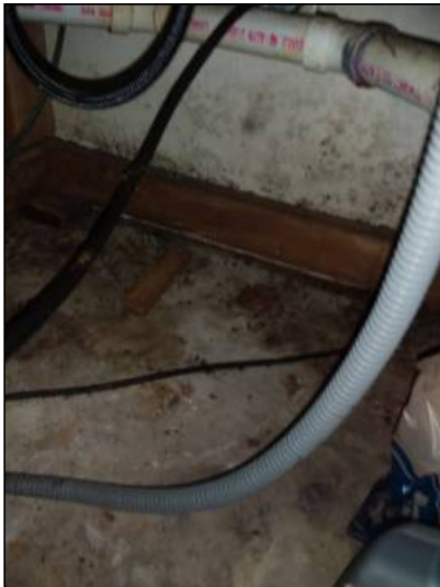
-Mold like stains are present, recommend remediation or cleanup as needed. Unable to determine condition of the underlying materials. Mainly at -underneath kitchen sink.
