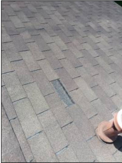
-The roof is missing shingles, recommend replacement of missing shingles. Mainly at - front left
