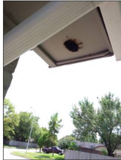
-Seal gaps and holes in soffit to help prevent water penetration or rodent intrusion. Mainly at - front
