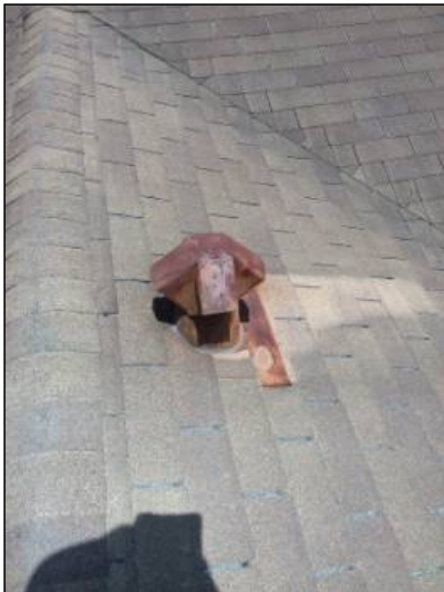
-Recommend painting all unpainted vents and flashings to help prevent damage due to UV rays or rust.
