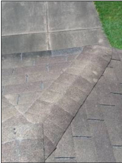
-The roof is missing shingles, recommend replacement of missing shingles. Mainly at - front left
