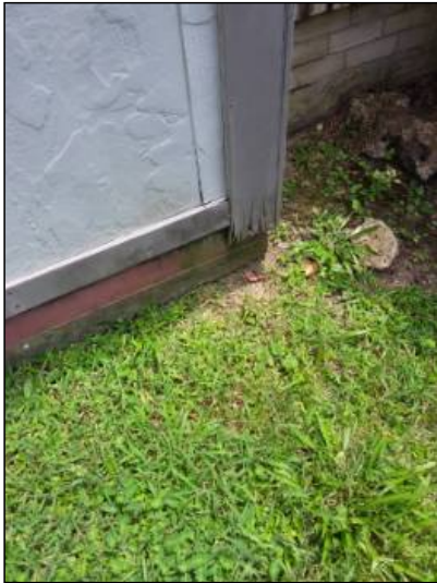
-Deterioration was noted at the trim, recommend replacing all deteriorated trim. Unable to determine the condition of the underlying materials. Mainly at - left side
