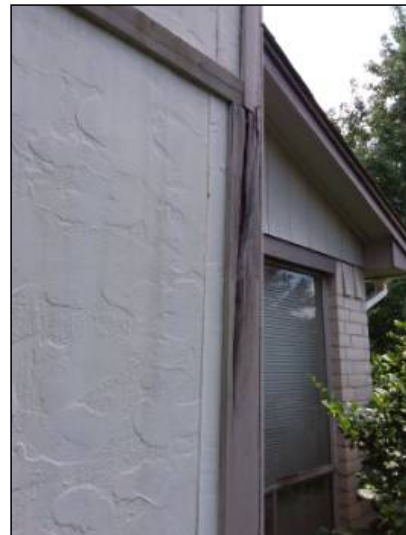
-Deterioration was noted at the trim, recommend replacing all deteriorated trim. Unable to determine the condition of the underlying materials. Mainly at - left side
