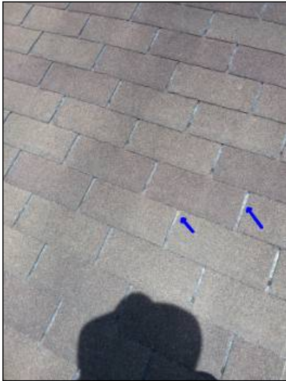
-Due to the excessive granular loss on the roof covering the roof may age prematurely. We recommend further review of the roof system for a better understanding of the present condition.
