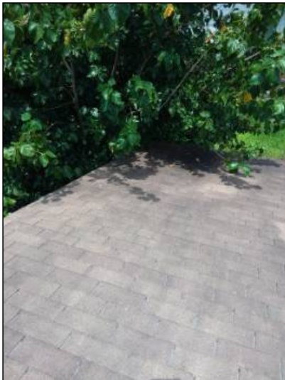
-Tree limbs should be kept trimmed at least 5' from roof to help prevent damage to the roof during windy conditions.
