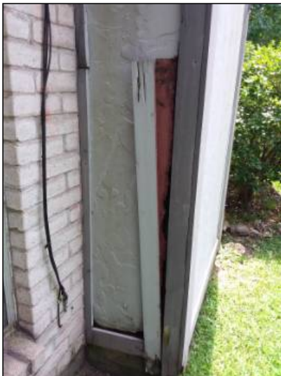
-Deterioration was noted at the trim, recommend replacing all deteriorated trim. Unable to determine the condition of the underlying materials. Mainly at - left side
