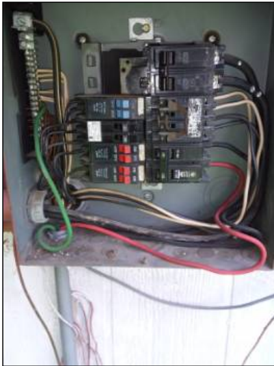
Overview of main electrical panel
