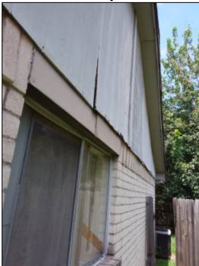
-Deterioration was noted at the siding, recommend replacing all deteriorated siding to help prevent further deterioration and water penetration. Unable to determine the condition of the underlying materials. Mainly at - right side
