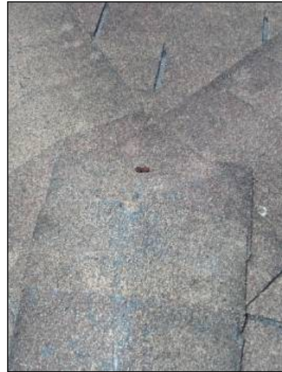
-All exposed nails and fasteners on roof should be sealed at all penetrations, ridges and roof to wall connections.
