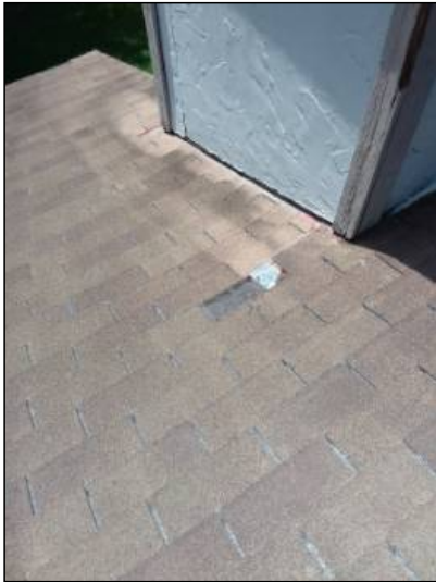
-The roof is missing shingles, recommend replacement of missing shingles. Mainly at front left
