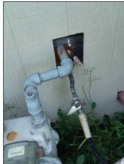
-Seal gaps and holes in siding to help prevent water penetration. Mainly at - rear
