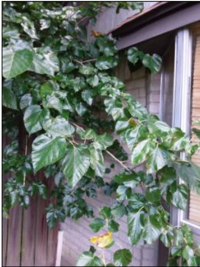
-Recommend trimming vegetation so that it is not in contact with the house. Vegetation in contact with the structure can hold moisture against the structure and promote damage of building materials.
