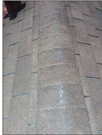
-Due to granular loss on portions of the ridge shingles these portions of the roof covering materials may age prematurely. May want to replace worn ridge shingles to help prolong the life of the roof. This is often due to normal wear due to the age of the roof.
