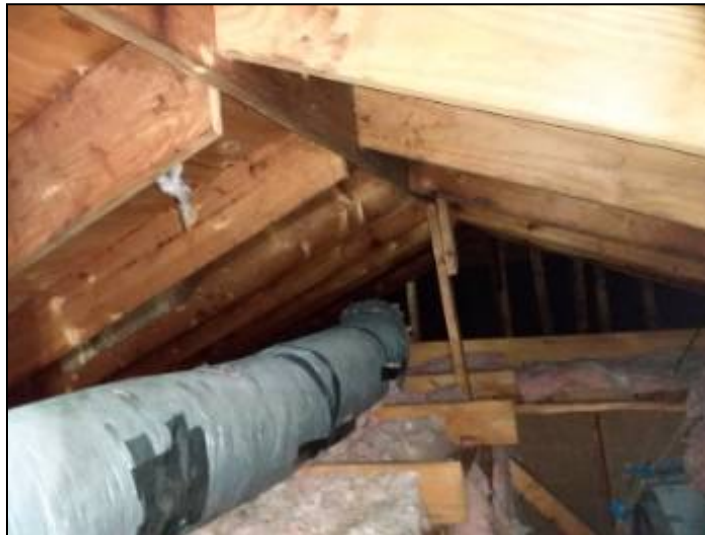
-Missing collar ties to hold ridge together.
