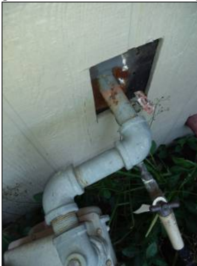
-Paint pipe at gas meter to help prevent premature deterioration.
