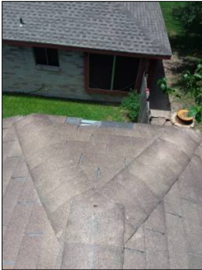
-The roof is missing shingles, recommend replacement of missing shingles. Mainly at - front left
