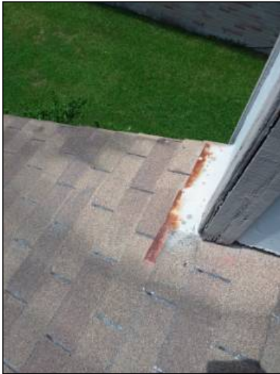
-There are signs of rusted flashings on the rooftop. We recommend painting or replacing all rusted or deteriorated flashings as needed.
