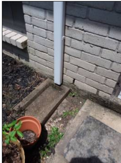
-The downspout is missing the 90 degree elbow to direct water away from foundation. Mainly at - front
