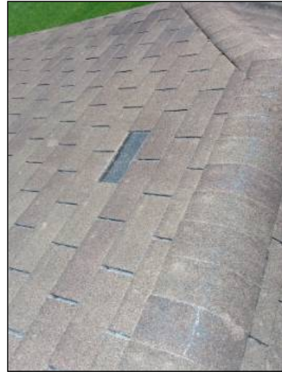
-The roof is missing shingles, recommend replacement of missing shingles. Mainly at - front right
