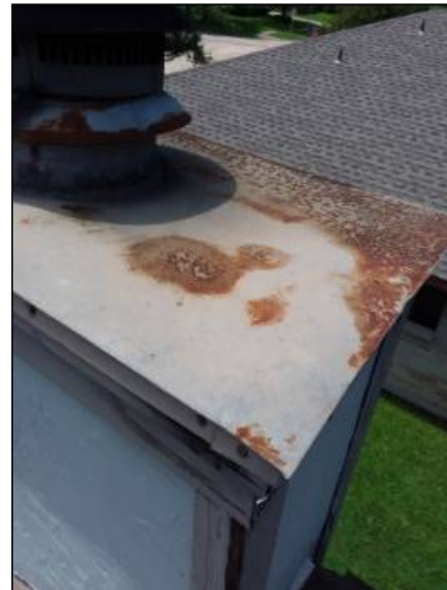
-There are signs of rusted flashings on the rooftop. We recommend painting or replacing all rusted or deteriorated flashings as needed.
