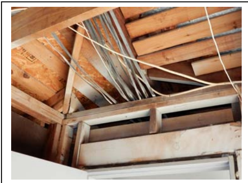
←Garage lacks adequate firestopping to the breezeway attic. Opening must be sealed properly, such as with drywall or 2x wood. This is to help stop a fire that starts in the garage from spreading to the main house structure.
