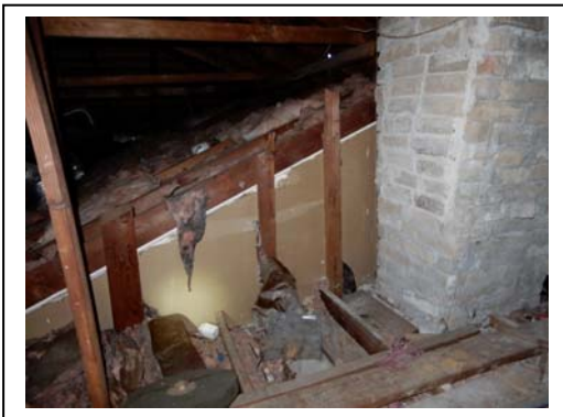
←Missing attic insulation at a few places, such as at the den raised ceiling vertical walls.
