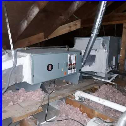
gas furnace attic
