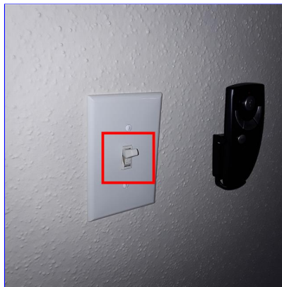
B. Item 23(Picture) damaged primary bedroom
