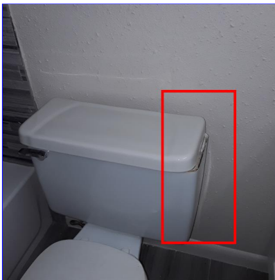
A. Item 6(Picture) toilet lid does not fit properly primary bath
