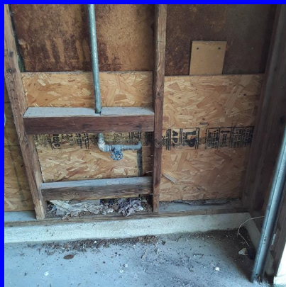
water shut off garage
