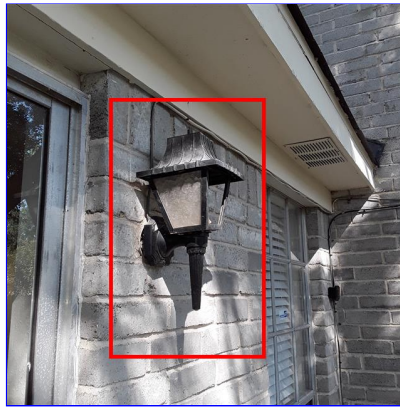
B. Item 19(Picture) fixture damaged rear
