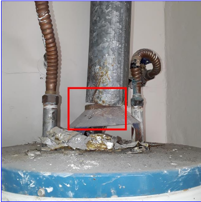
C. Item 5(Picture) pipe not connected
