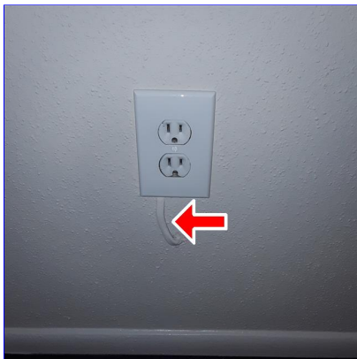
B. Item 12(Picture) multiple areas
