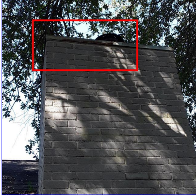
J. Item 1(Picture) rear
