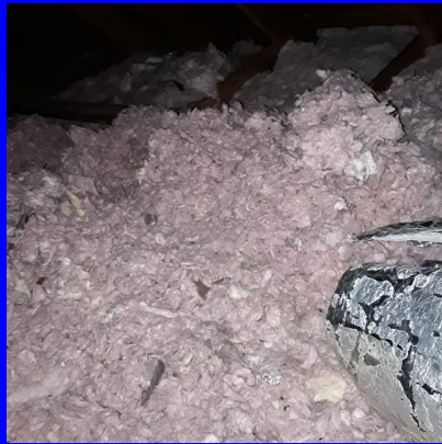
blown insulation less than 6 inches
