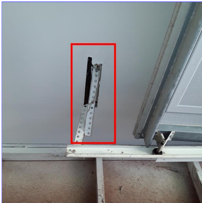
D. Item 3(Picture) garage
