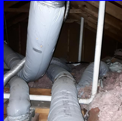
insulated ducts attic
