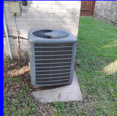
ac unit exterior rear
