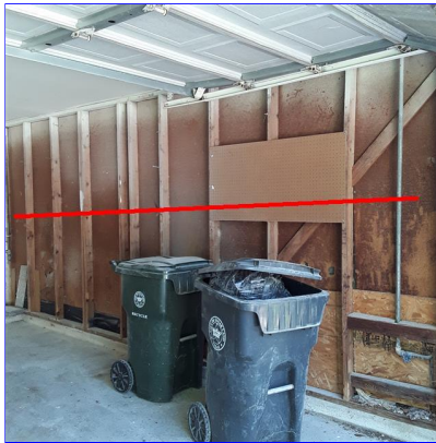
D. Item 2(Picture) garage
