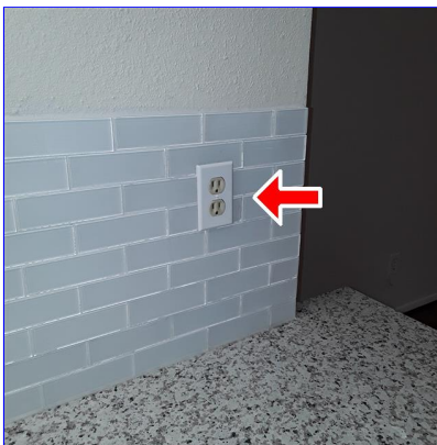
B. Item 4(Picture) kitchen outlets
