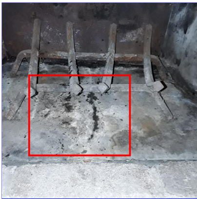
J. Item 3(Picture) water present in fireplace
