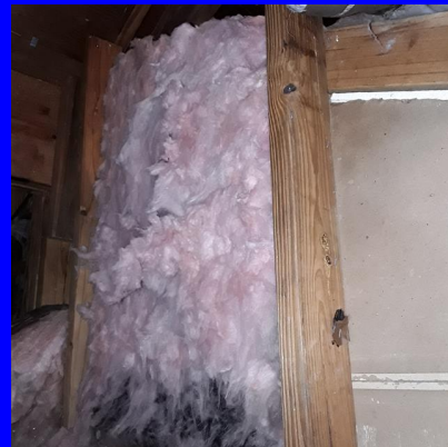
vertical insulation less than 6 inches
