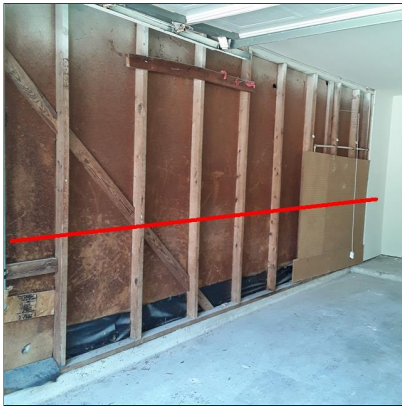
D. Item 1(Picture) garage
