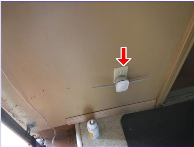
B. Item 3(Picture) No GFCI protection (garage)
