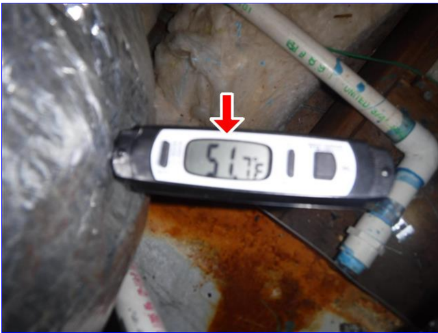
B. Item 2(Picture) View of the cooling system measured exit air temperature at the evaporator.
