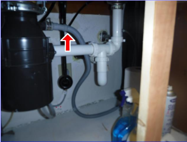
B. Item 1(Picture) Any drain line entering a food waste disposer should enter the disposer in a downward direction to prevent clogging.
