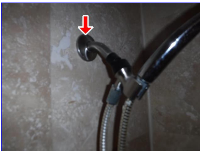
A. Item 6(Picture) Loose stem here
