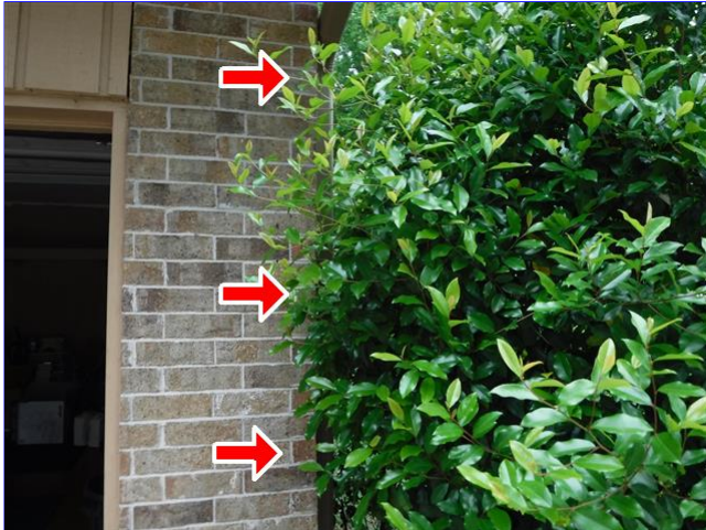
E. Item 1(Picture) Excess vegetation needs to be trimmed back
