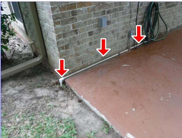
A. Item 4(Picture) This area needs to be insulated.
