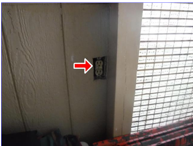
B. Item 7(Picture) Missing outlet cover here
