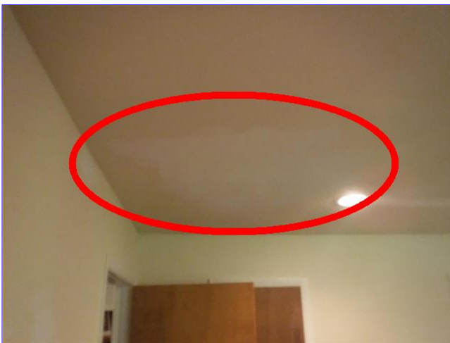
F. Item 3(Picture) Previous repair here
