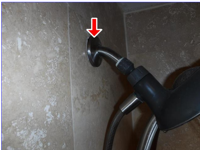
A. Item 5(Picture) Loose stem here
