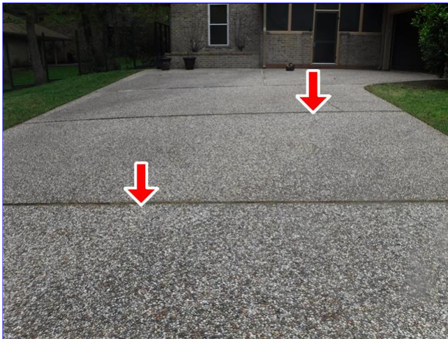
L. Item 1(Picture) Open expansion joints here
