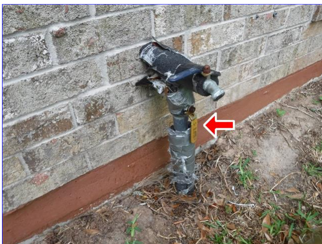
A. Item 2(Picture) View of main water shut off valve
