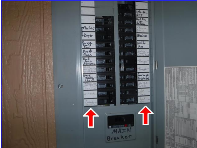
A. Item 1(Picture) View of labeled breaker panel
