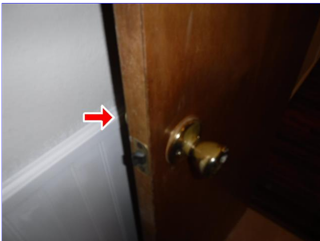
G. Item 1(Picture) Missing door stop here
