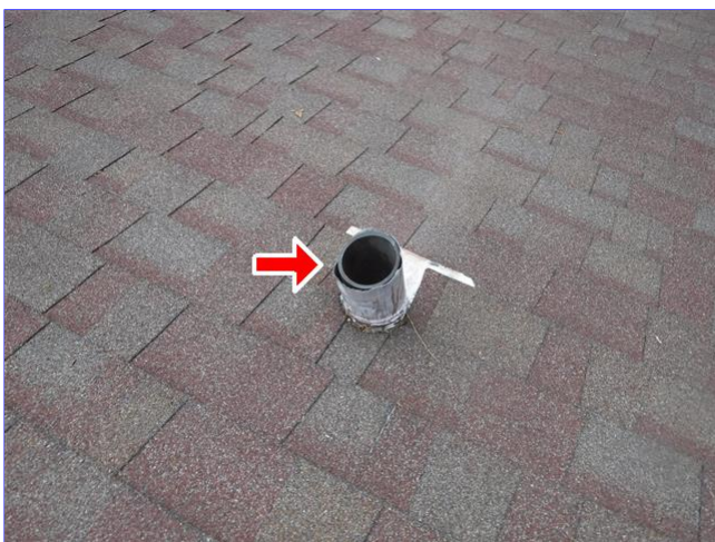
C. Item 7(Picture) Damaged vent seal here
