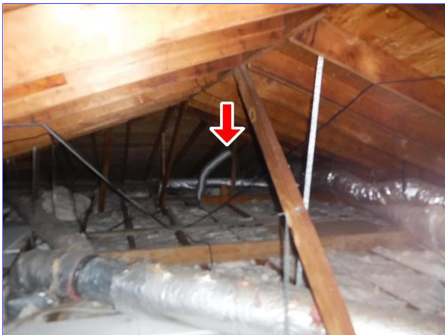
C. Item 1(Picture) Vent does not exit attic space here
