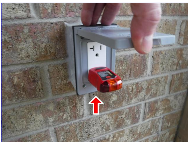
B. Item 5(Picture) No GFCI protection (exterior)
