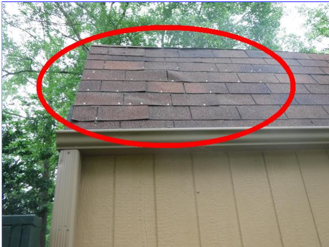
C. Item 9(Picture) Exposed nail heads here
