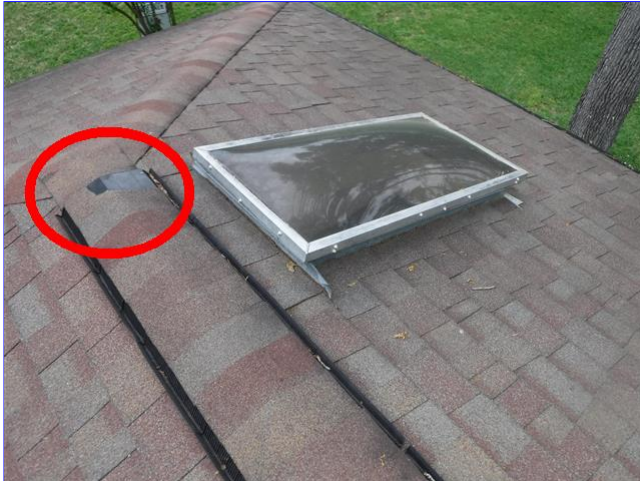
C. Item 8(Picture) Damaged shingle here
