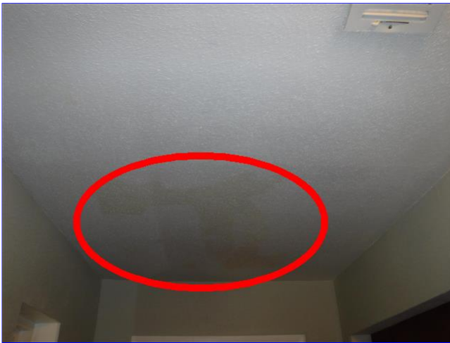
F. Item 2(Picture) Previous repair here
