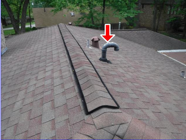
A. Item 1(Picture) Wrong type of exhaust vent here
