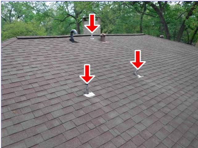
C. Item 5(Picture) Damaged vent seals here
