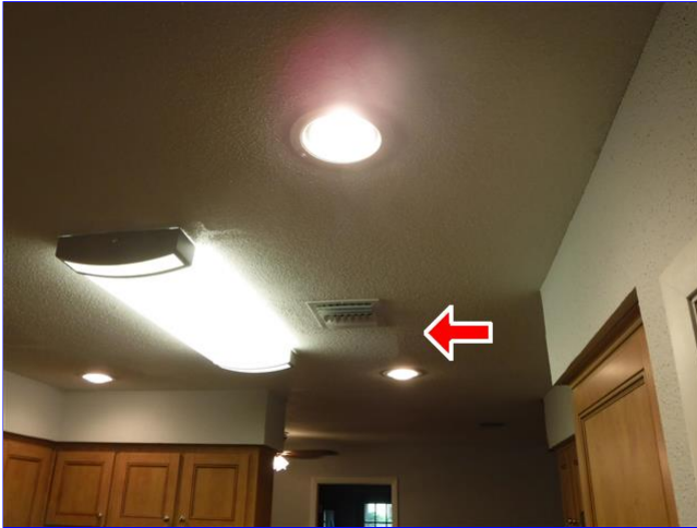
F. Item 1(Picture) Previous repair here
