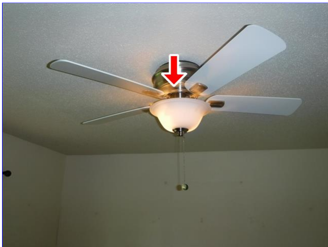
B. Item 9(Picture) Fan blades rubbing here
