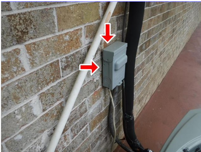
E. Item 2(Picture) This area needs to be sealed to the wall to prevent moisture and pest intrusion into the wall.
