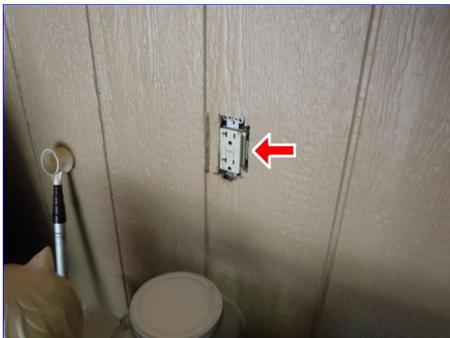
B. Item 6(Picture) Missing outlet cover here
