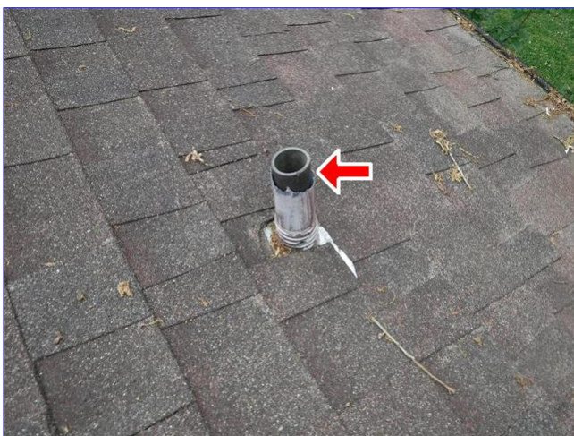
C. Item 6(Picture) Damaged vent seal here
