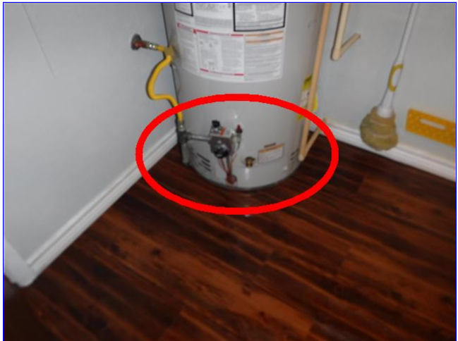
C. Item 2(Picture) Missing drain pan here
