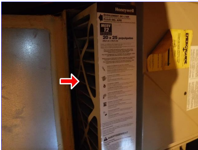
C. Item 1(Picture) Dirty filter here
