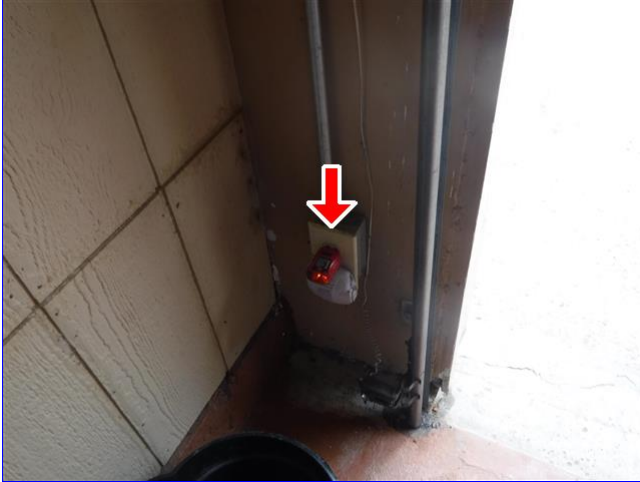
B. Item 2(Picture) No GFCI protection (garage)
