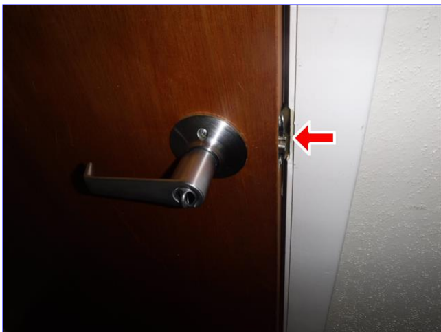
G. Item 3(Picture) Damaged striker plate here
