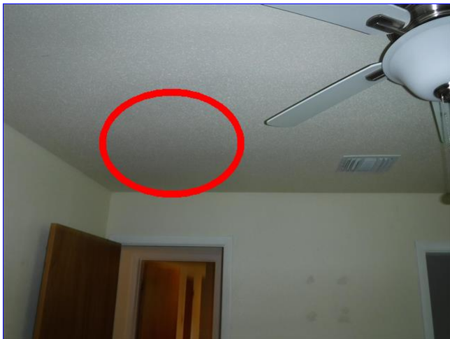
B. Item 1(Picture) No smoke alarms (bedrooms)
