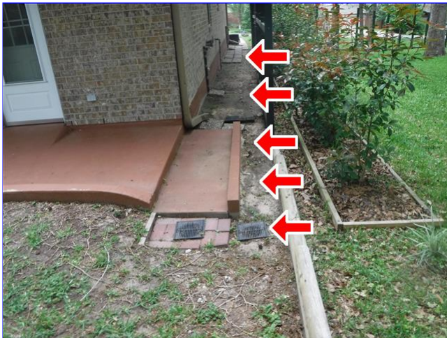
B. Item 1(Picture) Washed out area here
