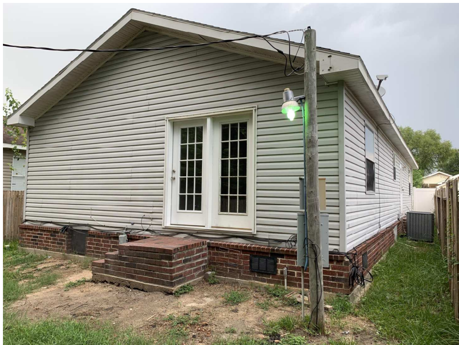
Photo Four Caption LEFT SIDE VIEW TAKEN FROM REAR YAD (PHOTO TAKEN 9-11-2020)
