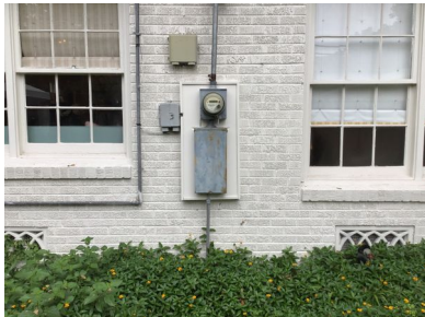
Service entrance cable location: Overhead
