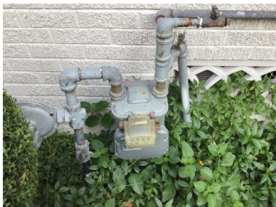
Unable to Verify Gas Line Bonding:
