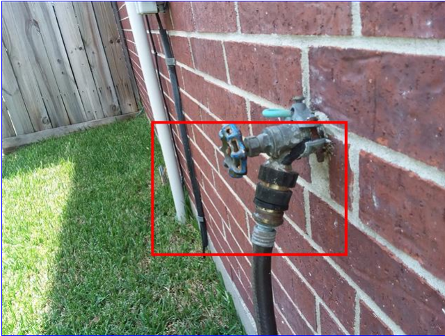
A. Item 1(Picture) Anti backflow device is missing from left exterior hose bib.
