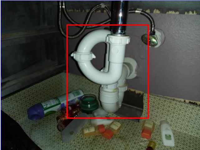
B. Item 7(Picture) Plumbing drain for vanity in the first floor powder room is incorrect.
