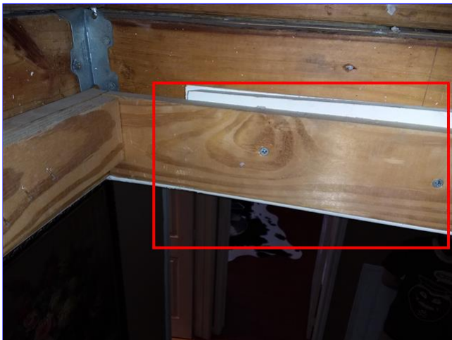
D. Item 2(Picture) The incorrect fasteners were used at the attic ladder assembly.
