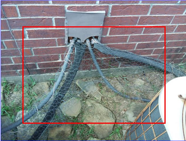
B. Item 3(Picture) Refrigerant line insulation is inadequate.
