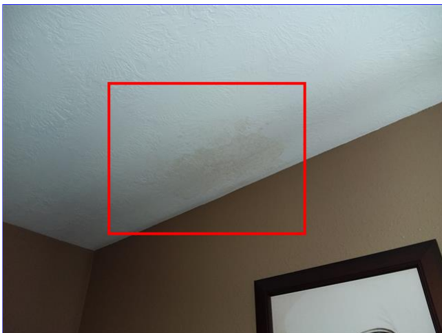
G. Item 1(Picture) Moisture staining was discovered at the ceiling in the second floor living room.
