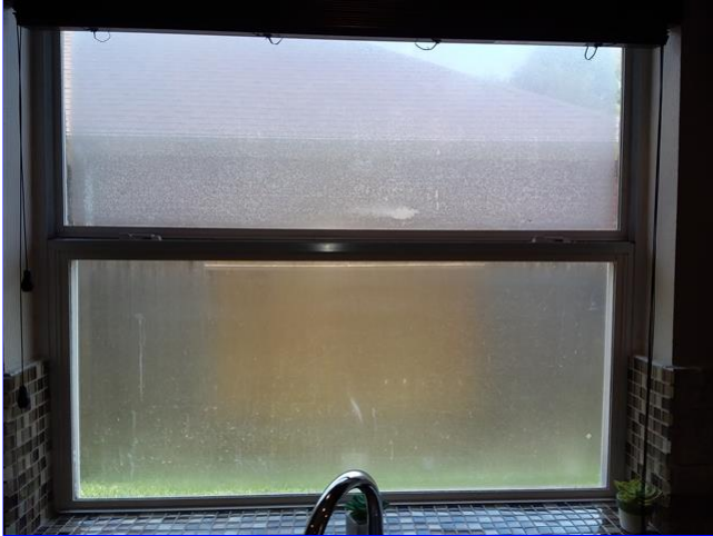
H. Item 2(Picture) Thermal seal is damaged at kitchen window.
