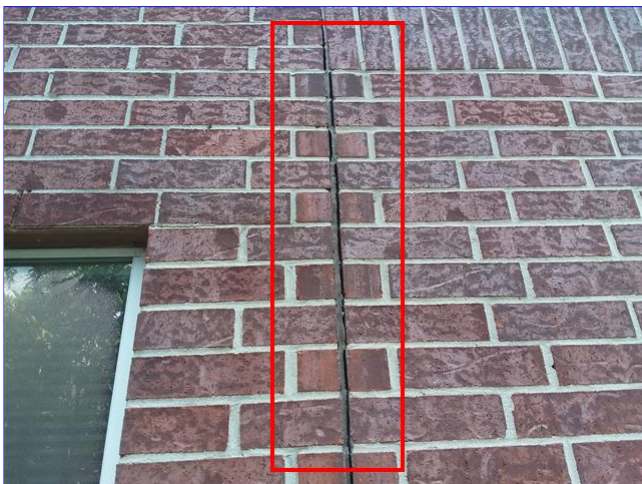
E. Item 3(Picture) Re caulk the expansion joint at the right exterior.
