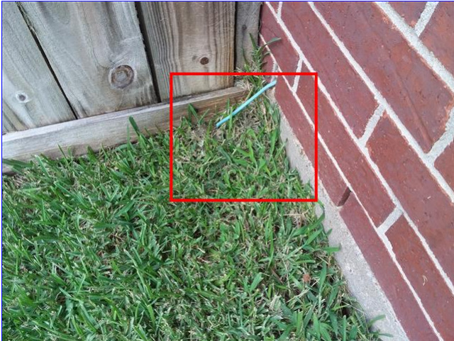
A. Item 5(Picture) Secondary ground wire is not attached to grounding rod.
