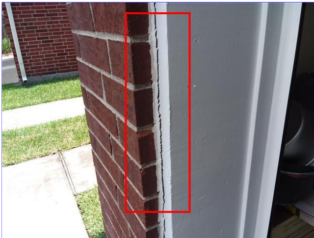
F. Item 7(Picture) Caulking is separating at the garage door frames.
