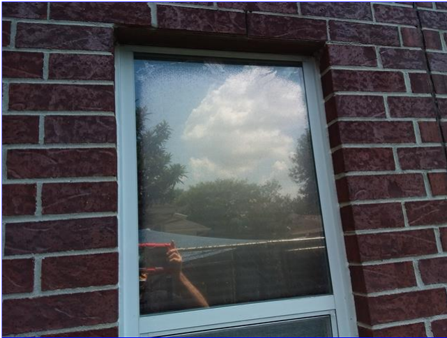
H. Item 3(Picture) Thermal seal is damaged at kitchen window.
