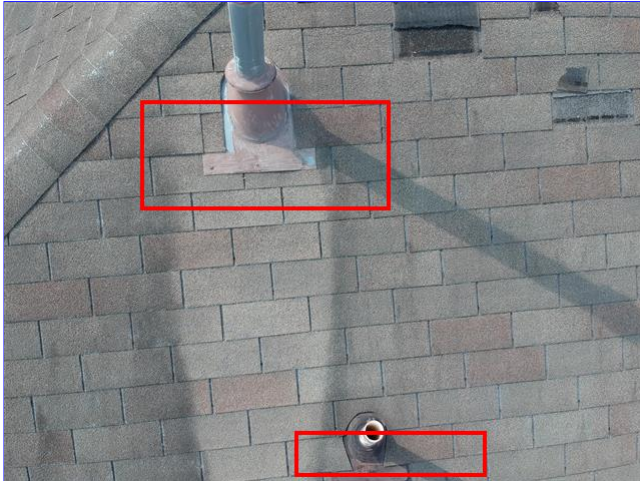
C. Item 5(Picture) Exposed nail heads at multiple areas around the home.
