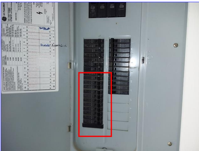
A. Item 6(Picture) Arc fault breakers missing from the electrical service panel.
