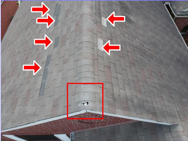
C. Item 1(Picture) Shingles are missing and or damaged at the multiple areas of the roof.
