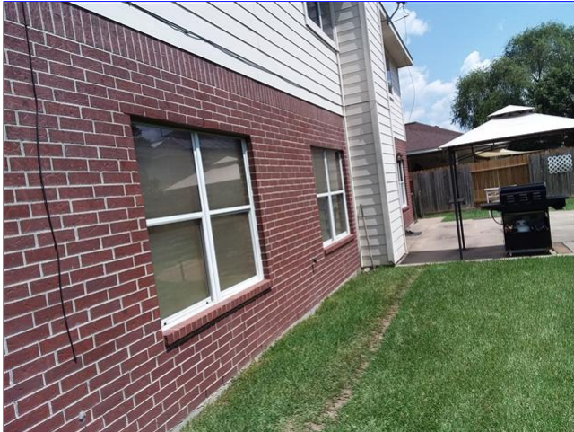
H. Item 6(Picture) Screens are missing from multiple windows around the home.
