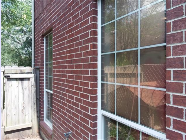
H. Item 4(Picture) Multiple windows around the home have damaged thermal seals.
