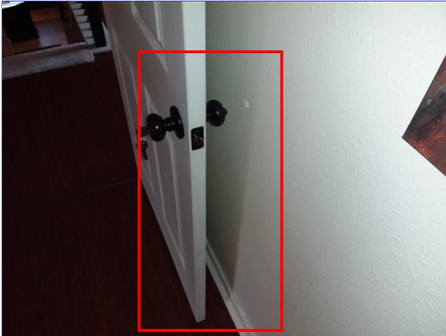
F. Item 12(Picture) Door stops missing from multiple doors around the home.
