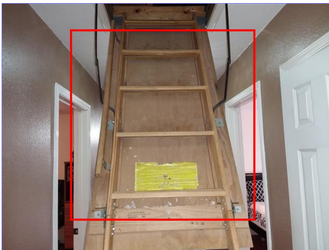
D. Item 1(Picture) Insulation missing from attic ladder assembly.
