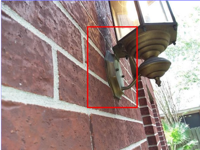
E. Item 1(Picture) Wall mounted light fixtures should be sealed to the wall.
