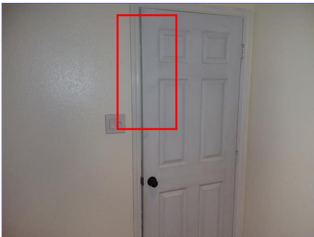
F. Item 10(Picture) Door to the second floor office is not hung correctly and will not close.
