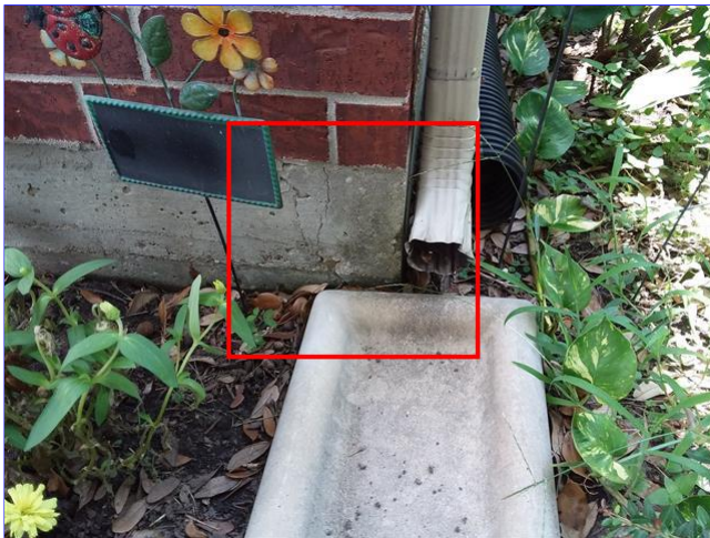
A. Item 2(Picture) A crack was discovered at the right front corner of the garage.
