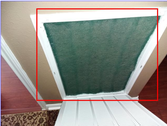
C. Item 1(Picture) Second floor return air filter needs to be replaced.
