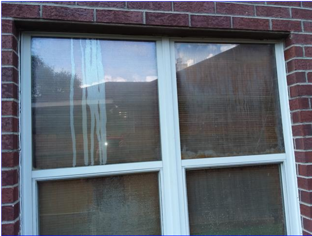
H. Item 5(Picture) Multiple windows around the home have damaged thermal seals.
