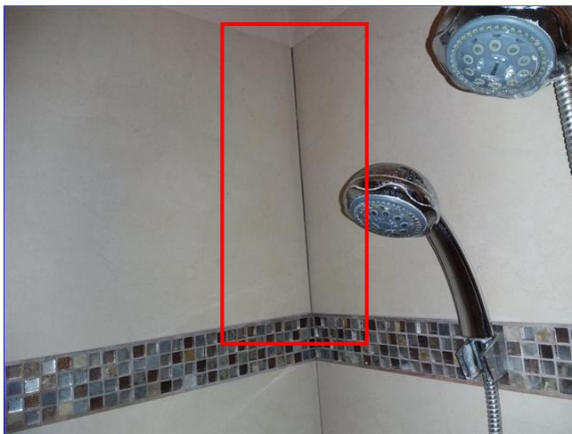
B. Item 3(Picture) Caulking and grout are missing from master shower enclosure.
