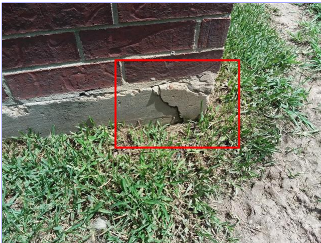
A. Item 3(Picture) Cracks at the corners of the foundation at multiple areas.
