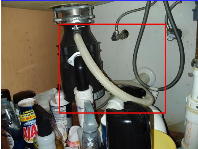
A. Item 2(Picture) High loop is missing from the dishwasher drain line in the kitchen.
