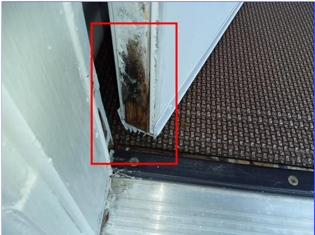
F. Item 8(Picture) Rear entry door is showing signs of wood rot on the inside.
