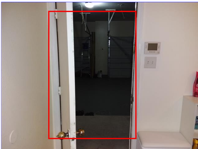
F. Item 1(Picture) Garage walk in door should self close.
