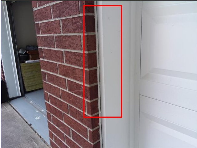
F. Item 6(Picture) Caulking is separating at the garage door frames.
