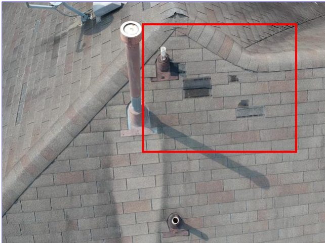
C. Item 3(Picture) Shingles are missing and or damaged at the multiple areas of the roof.
