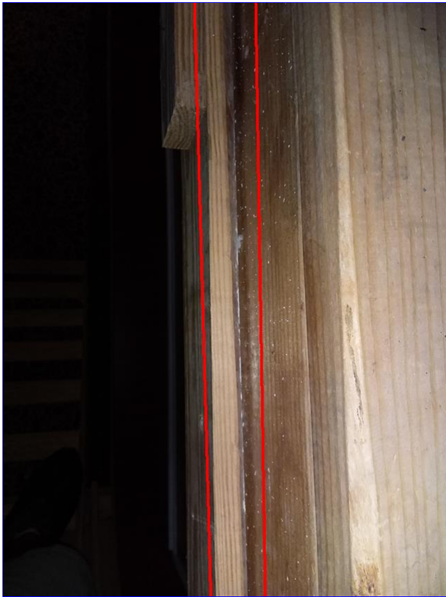
D. Item 3(Picture) foam seal is missing from the attic rough opening.
