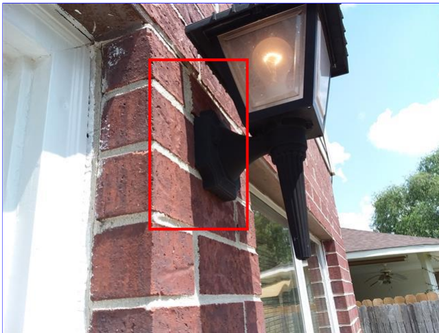
E. Item 2(Picture) Wall mounted light at the rear of the home is not sealed.
