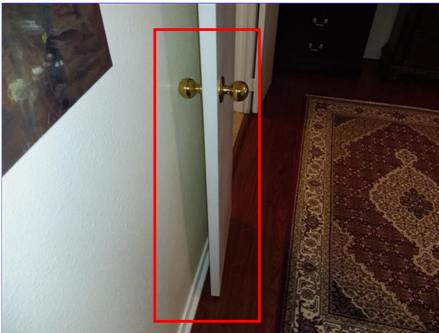
F. Item 13(Picture) Door stops missing from multiple doors around the home.
