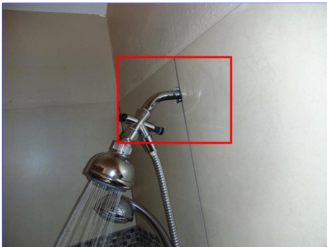
B. Item 4(Picture) Caulking and grout are missing from master shower enclosure.
