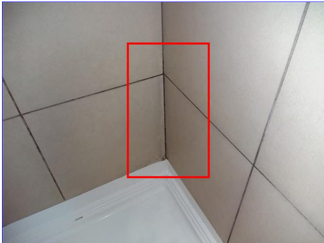
B. Item 2(Picture) Caulking and grout are missing from master shower enclosure.
