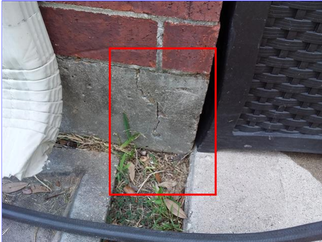
A. Item 1(Picture) A crack in the foundation was discovered at the left front corner.
