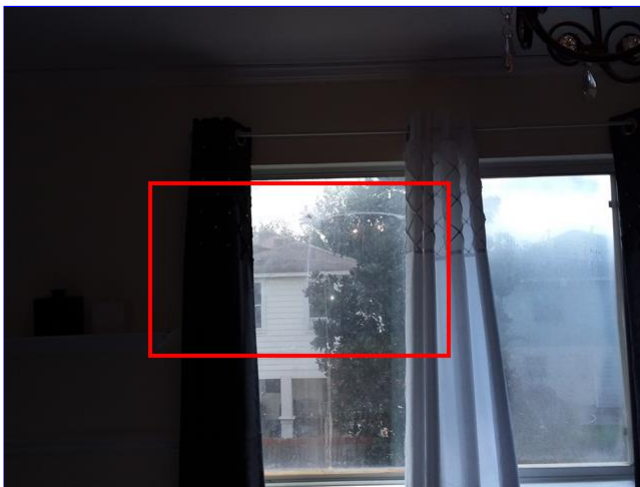
H. Item 7(Picture) Cracked window in the second floor left rear bedroom.
