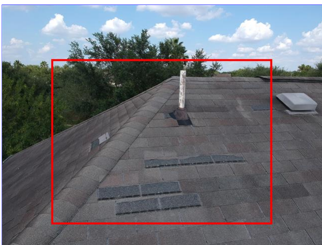
C. Item 4(Picture) Shingles are missing and or damaged at the multiple areas of the roof.
