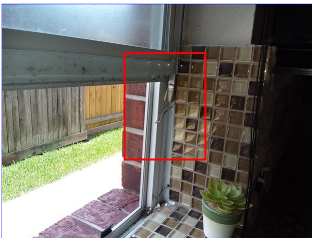
H. Item 1(Picture) Guide spring is detached at the kitchen window.
