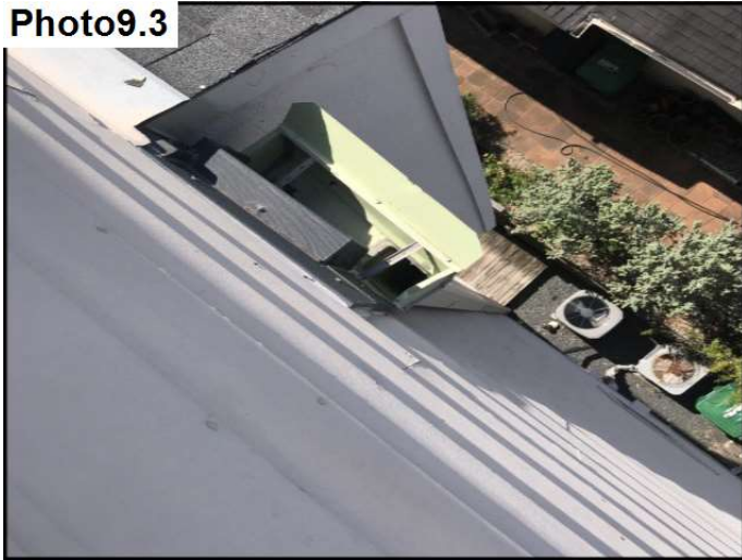
Reseal scuppers as needed.
