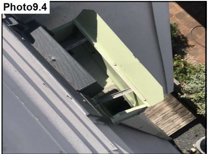
Reseal scuppers as needed.
