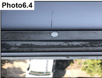
Seal alarm sensors as needed.
