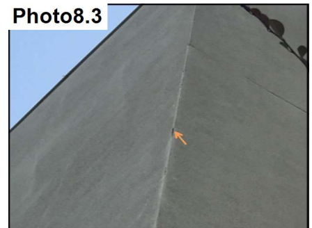
Rust noted at corner of wall.
