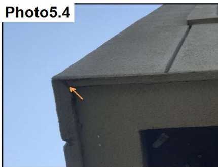
Moisture stain is present at bottom of wall.
