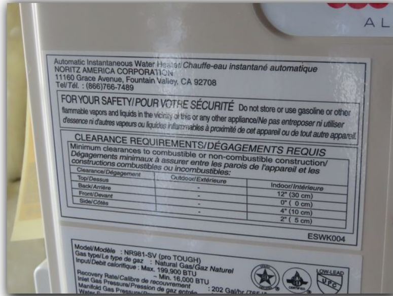
Water heater Temperature and Pressure Relief Valve
