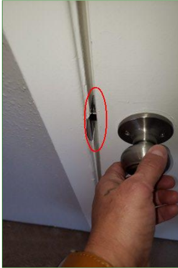
4.4 Item 1(Picture) Door will not latch
