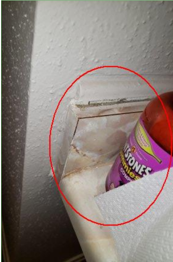
5.0.B Item 1(Picture) Damaged kitchen counter is in need of repair.
