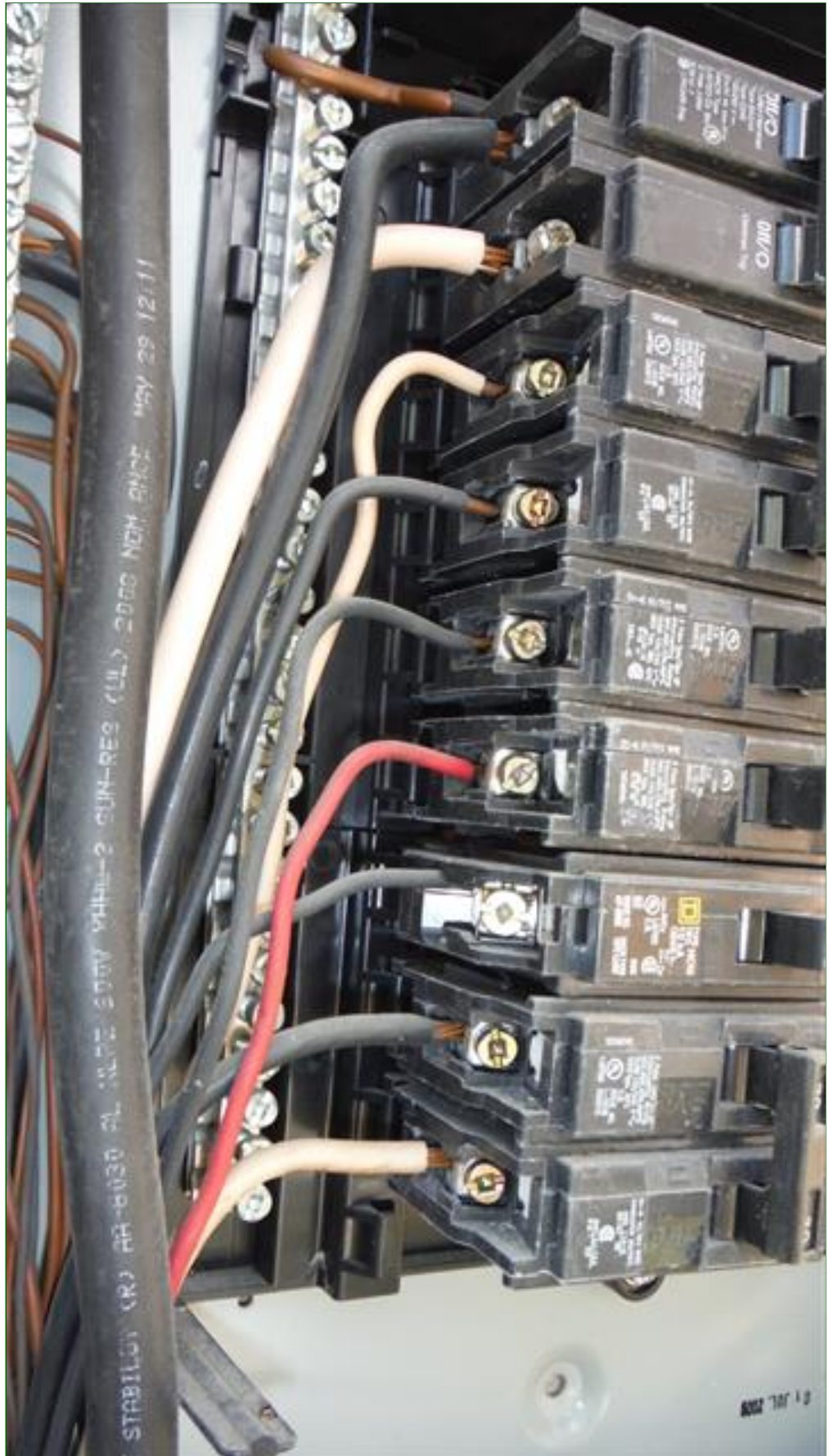
8.1 Item 6(Picture) 1908 circuit connections ok Page 82 of 126
