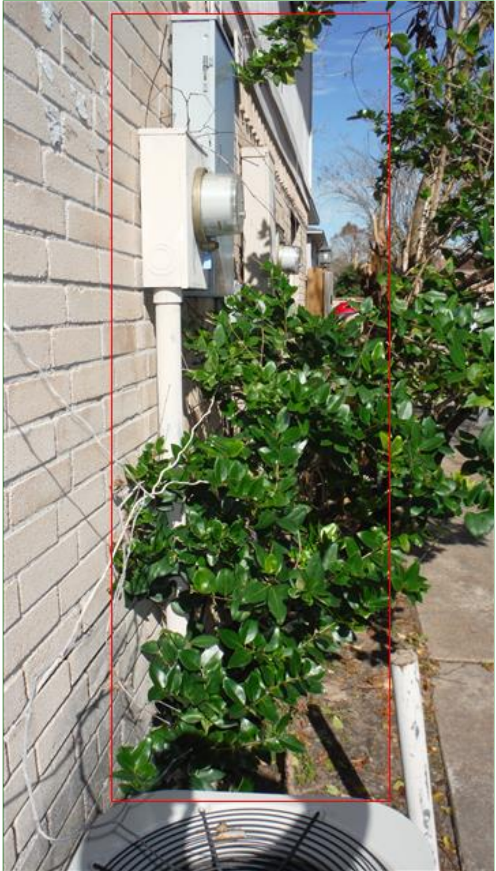
8.1 Item 1(Picture) Bushes must be trimmed back and away from panels. 3 feet of clearance is required in front of panels and 30 inches to either side.
