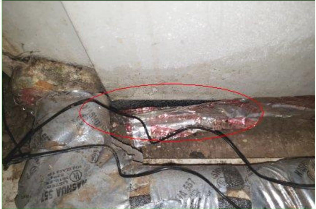
9.5 Item 6(Picture) Loose tape on air handler is in need of repair by a HVAC contractor
