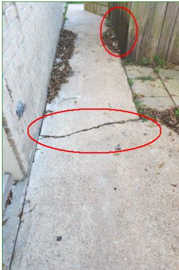
2.3 Item 6(Picture) Cracked walkway is in need of repair.
