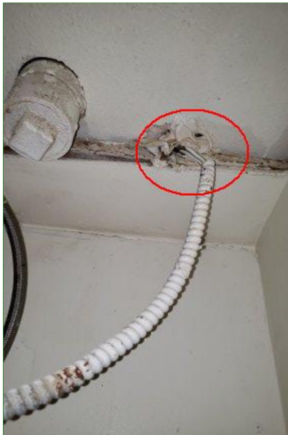
3.12 Item 4(Picture) Improper food waste disposal power supply
