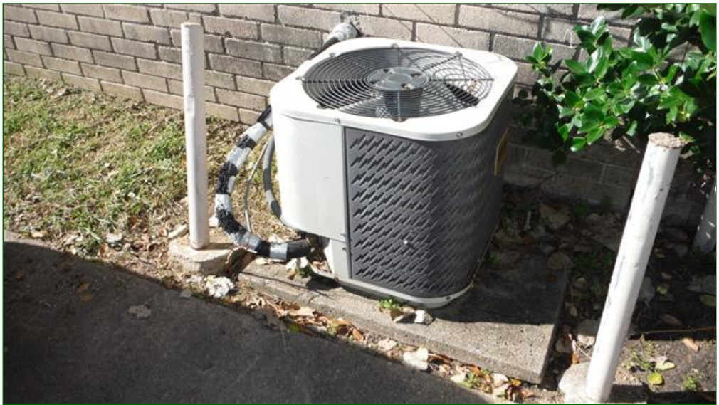
9.5 Item 11(Picture) Unit 1908 compressor
