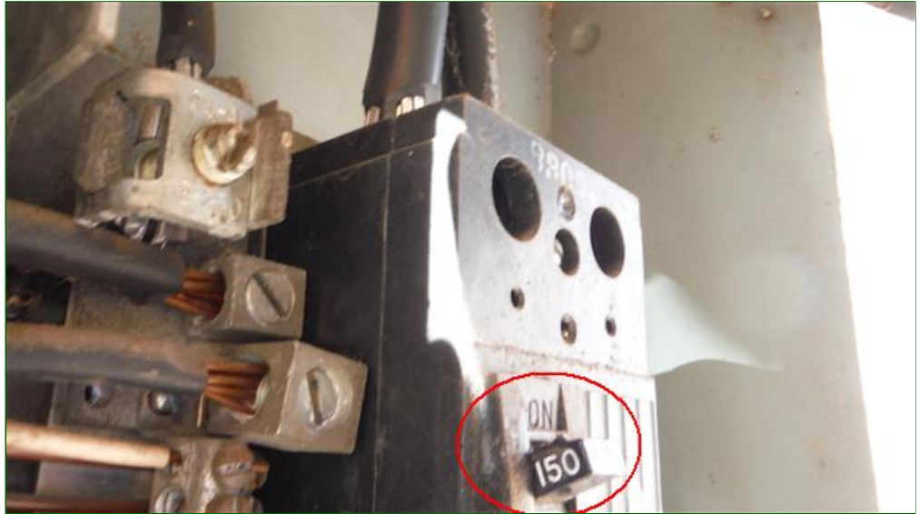
8.1 Item 20(Picture) Unit 1910 150 amp service
