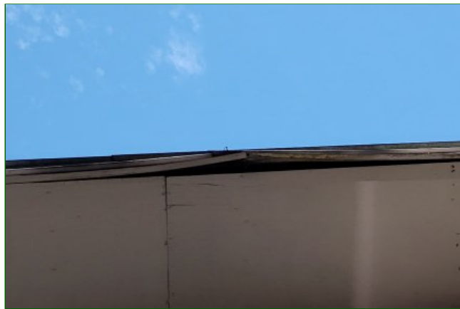
2.5 Item 5(Picture) Deteriorated soffit/fascia is in need of repair
