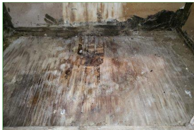
9.5 Item 9(Picture) Damaged/deteriorated materials under air handler above ceiling repairs in living room. The area was dry at the time of inspection, monitor and repair as necessary.
