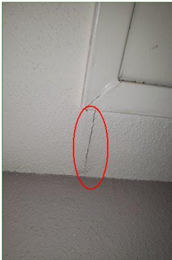
4.0 Item 2(Picture) Ceiling cracks discovered in both units are in need of repair
