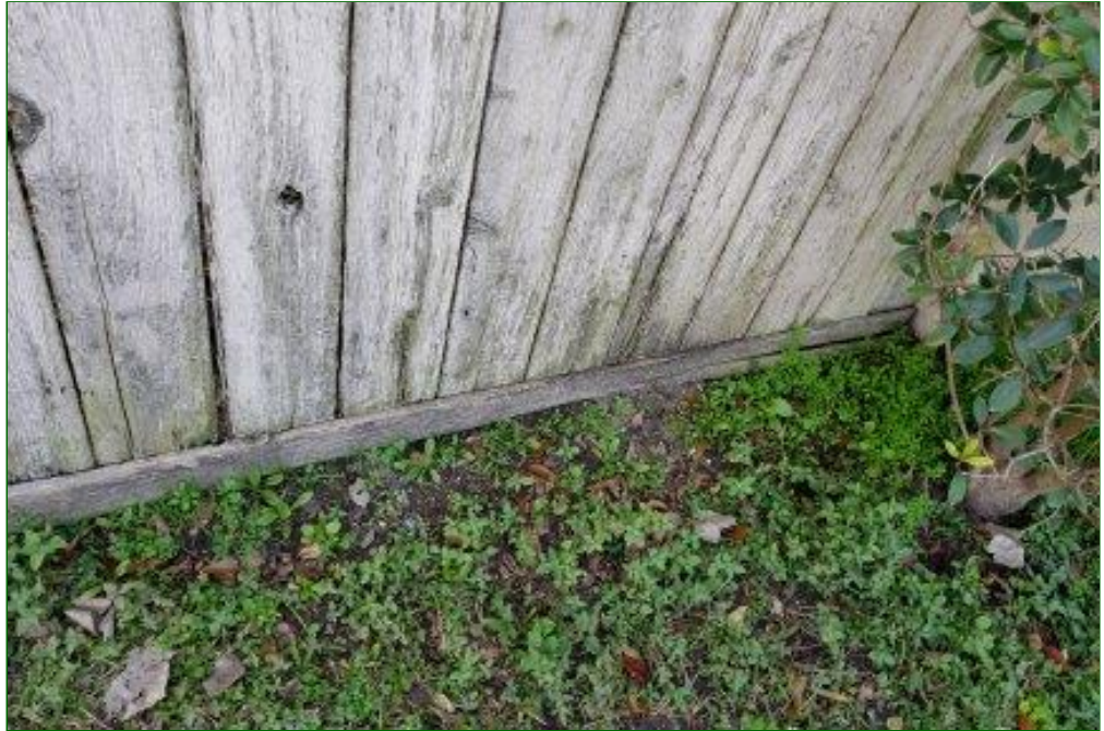
2.3 Item 5(Picture) Damaged/deteriorated fencing materials are in need of repair.
