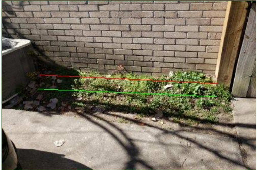
6.0 Item 3(Picture) Soil too high on brick
