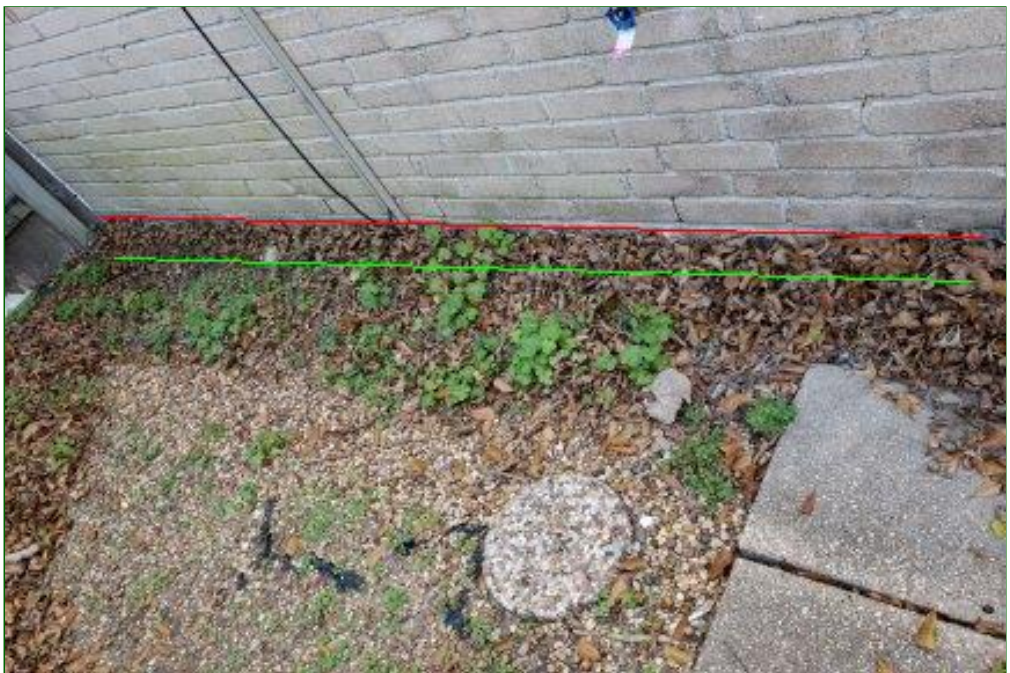
6.0 Item 6(Picture) Soil too high on brick
