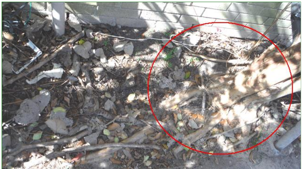
2.4 Item 2(Picture) Trees at rear of building should be removed to prevent differential settlement of the building.
