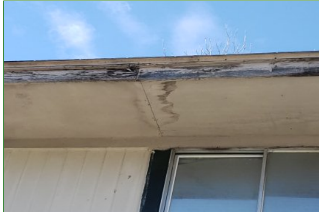
2.5 Item 4(Picture) Deteriorated soffit/fascia is in need of repair
