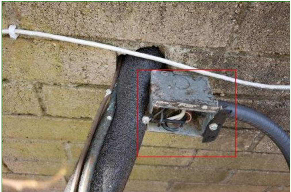
9.5 Item 20(Picture) Compressor power supply junction box is in need of repair
