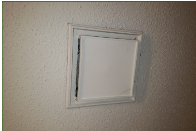
5.6.B Item 1(Picture) Exhaust fan in Unit 1910 Exhaust fan not working and in need of repair/replacement.
