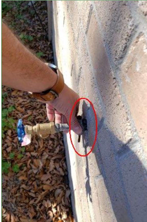
2.6 Item 1(Picture) Loose ground on exterior hose bib is in need of repair.
