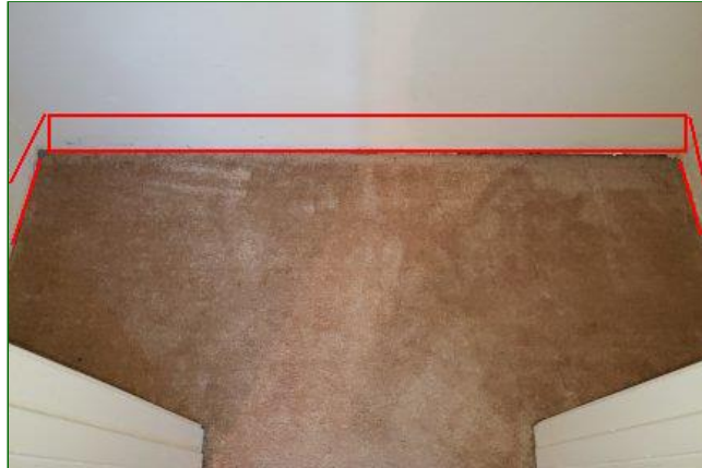
4.2 Item 10(Picture) Floor trim missing throughout unit 1908
