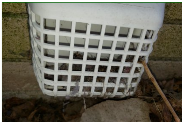
3.14 Item 1(Picture) Clogged Dryer vent termination
