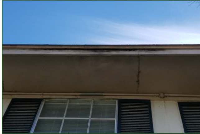
2.5 Item 1(Picture) Deteriorated soffit/fascia is in need of repair
