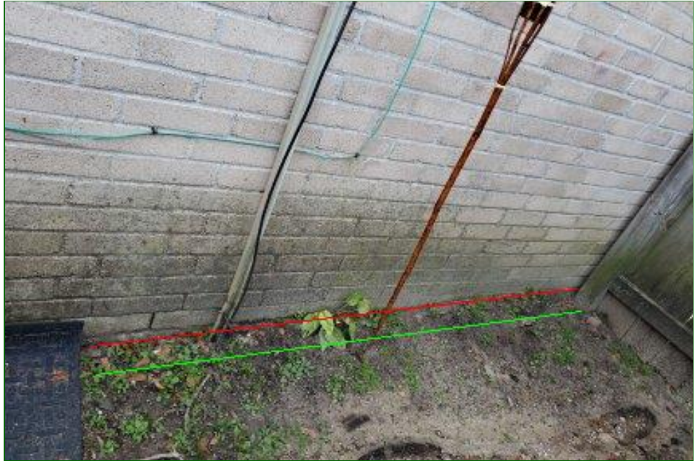
6.0 Item 7(Picture) Soil too high on brick
