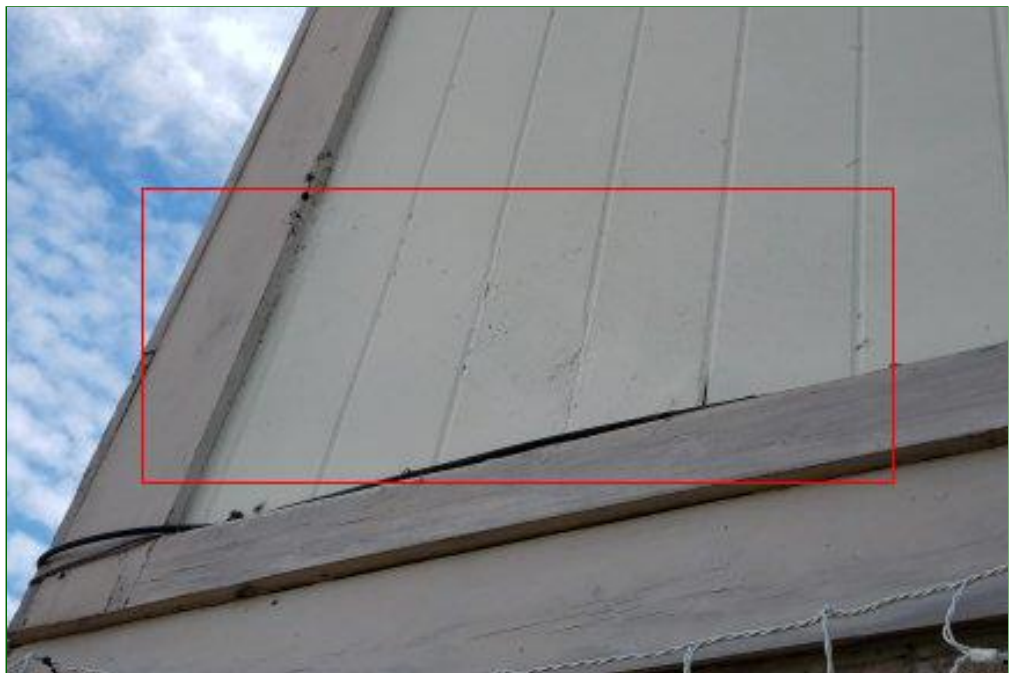
2.0 Item 4(Picture) Damaged/deteriorated siding/trim
