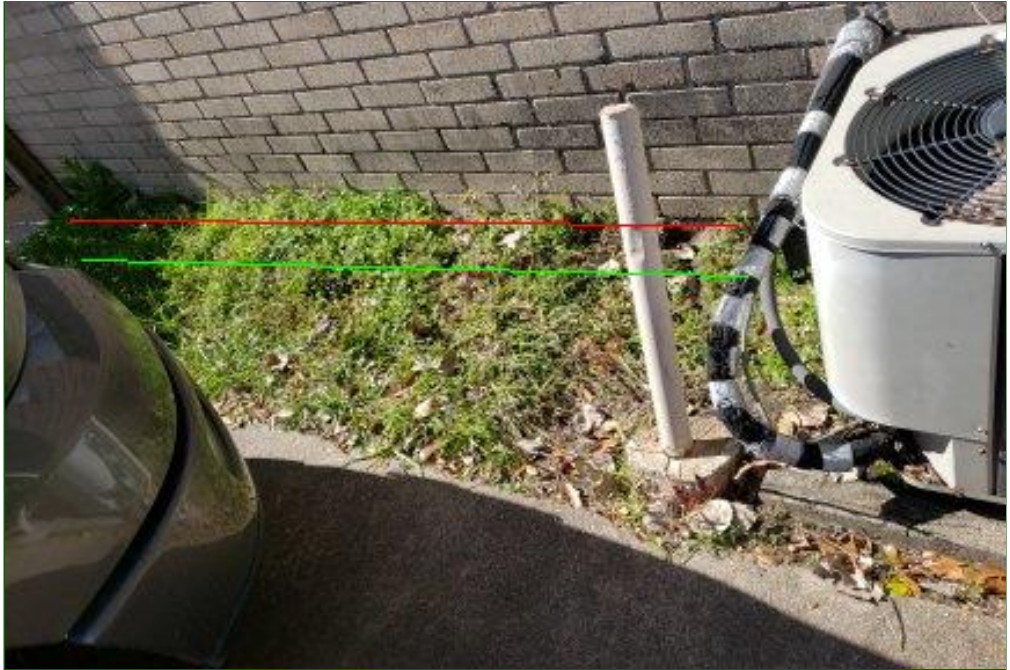
6.0 Item 5(Picture) Soil too high on brick
