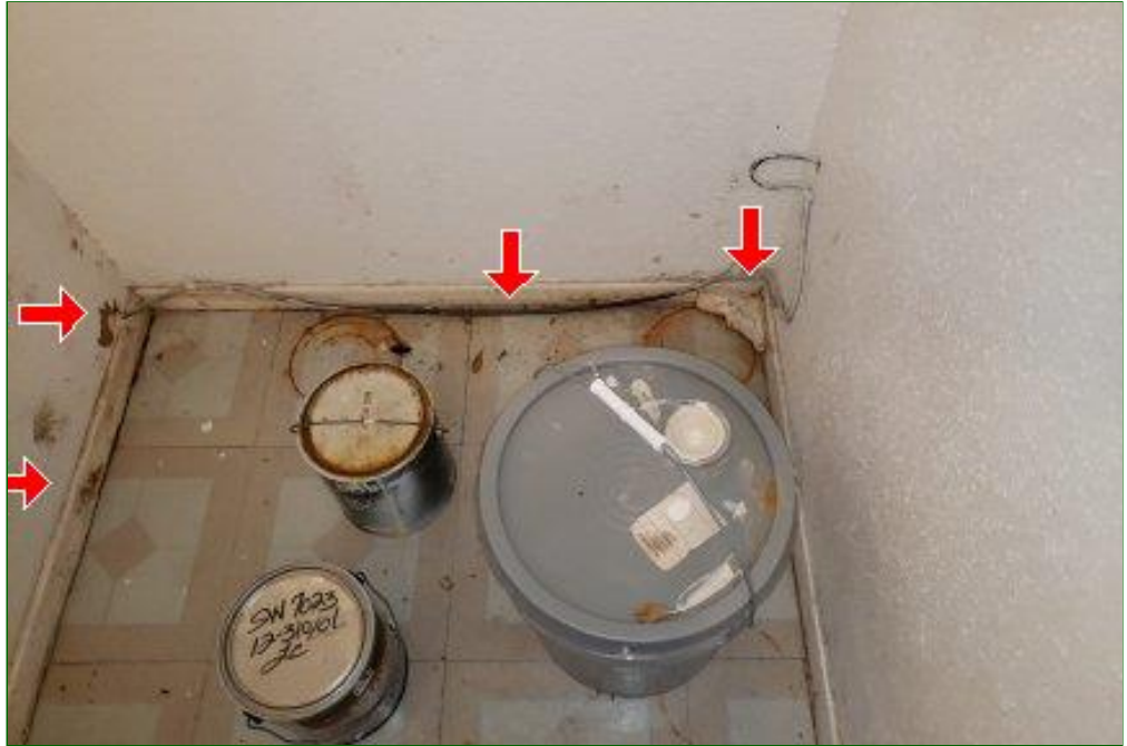
4.2 Item 4(Picture) Evidence of moisture entering front entry
