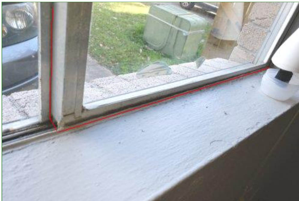
4.5 Item 3(Picture) Rear bedroom window loose in track
