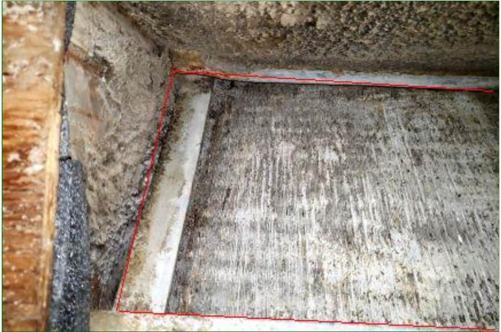
9.5 Item 10(Picture) Evaporative coils are dirty and in need of service/repair.
