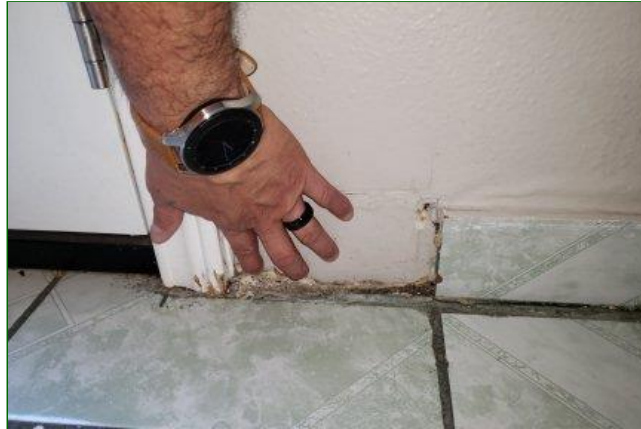
4.2 Item 7(Picture) Deteriorated drywall at side exit
