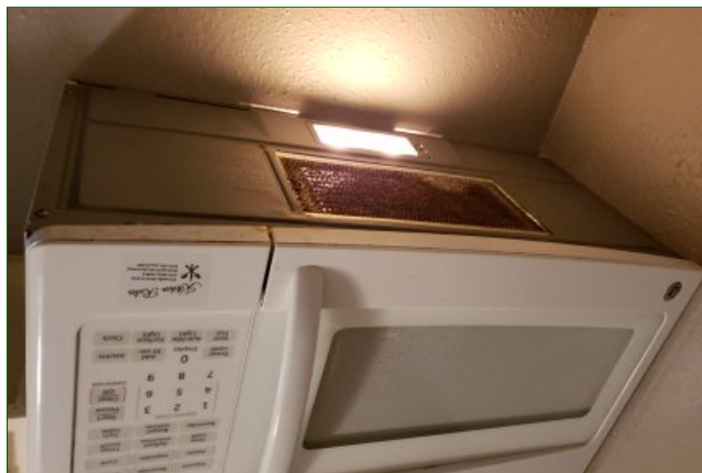
3.11 Item 1(Picture) Range hood exhaust system
