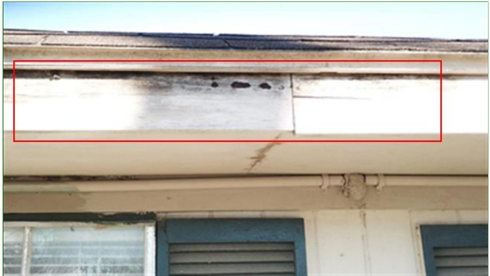
2.5 Item 7(Picture) Deteriorated soffit/fascia is in need of repair
