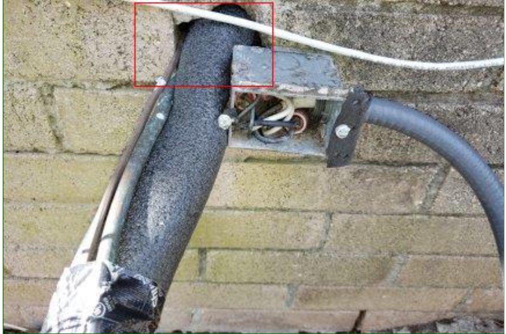
9.5 Item 19(Picture) Seal wall penetrations
