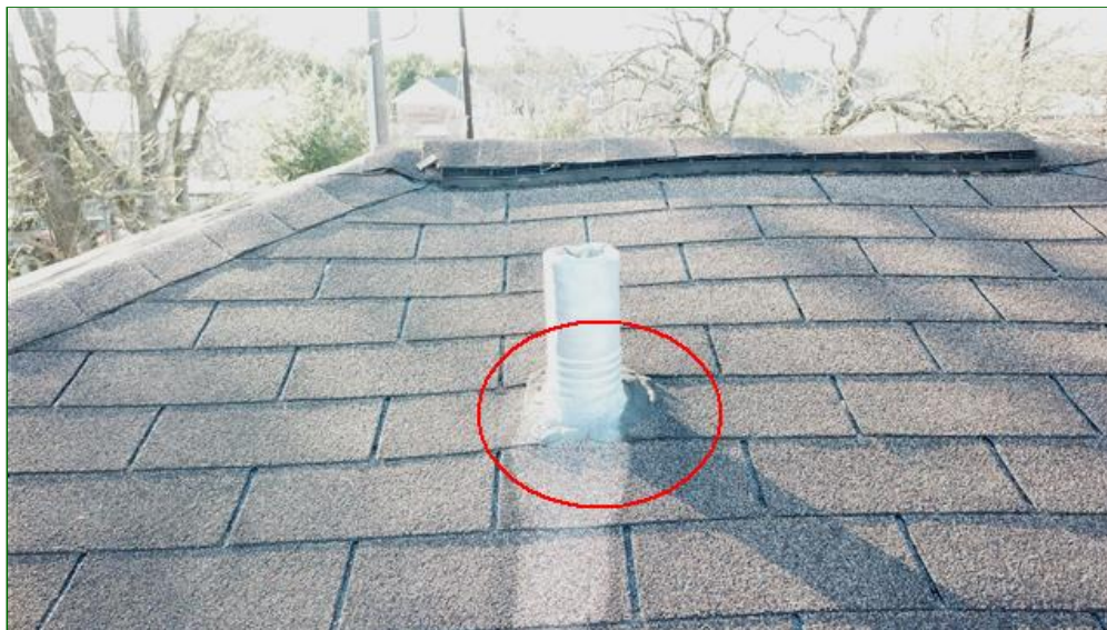
1.2 Item 1(Picture) Improperly installed vents
