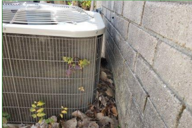
9.5 Item 1(Picture) Compressor should be installed 24 inches from wall as per manufacturers installation instructions
