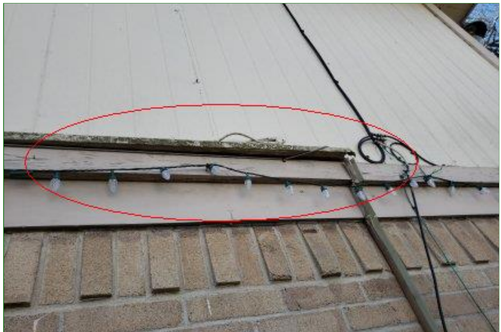
2.0 Item 2(Picture) Damaged/deteriorated siding/trim
