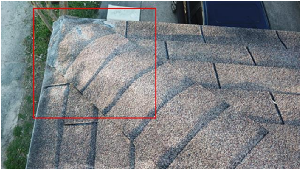
1.0 Item 6(Picture) Damaged shingles
