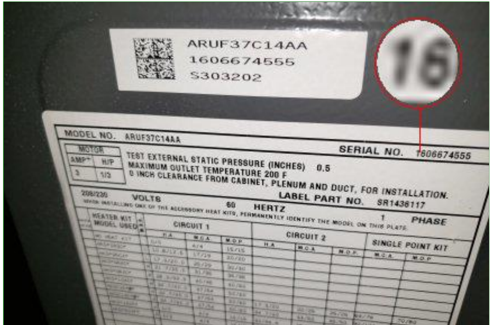
9.5 Item 16(Picture) Air handler was manufactured in 2016
