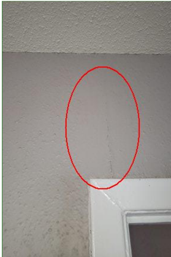
4.1 Item 1(Picture) Wall crack
