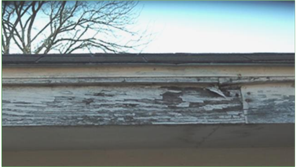
2.5 Item 9(Picture) Deteriorated soffit/fascia is in need of repair
