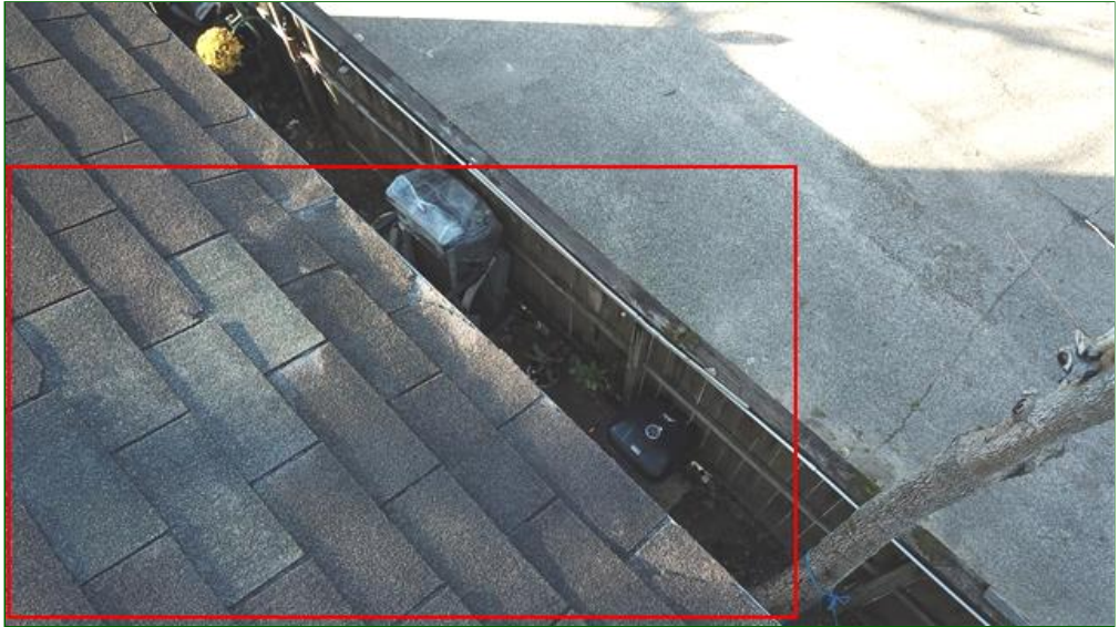
1.0 Item 5(Picture) Damaged shingles
