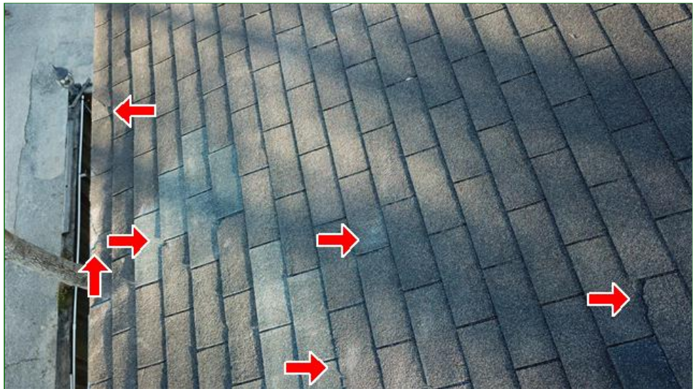
1.0 Item 4(Picture) Damaged shingles
