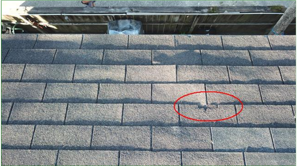
1.0 Item 7(Picture) Damaged shingles
