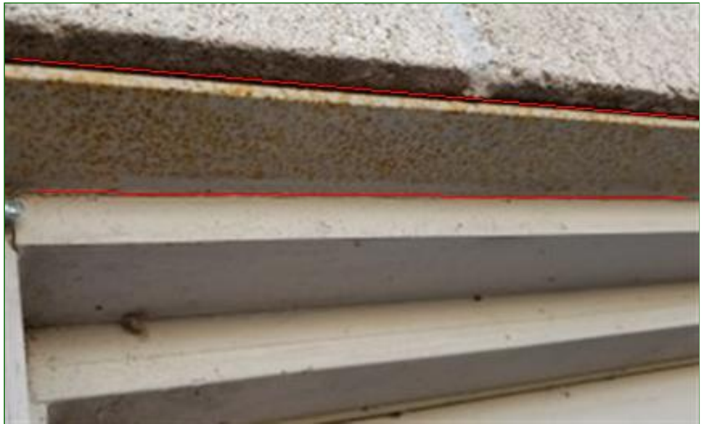
2.1 Item 3(Picture) Rusty lintels above doors and windows are in need of painting with a rust inhibitor to prevent premature deterioration of load bearing lintels.
