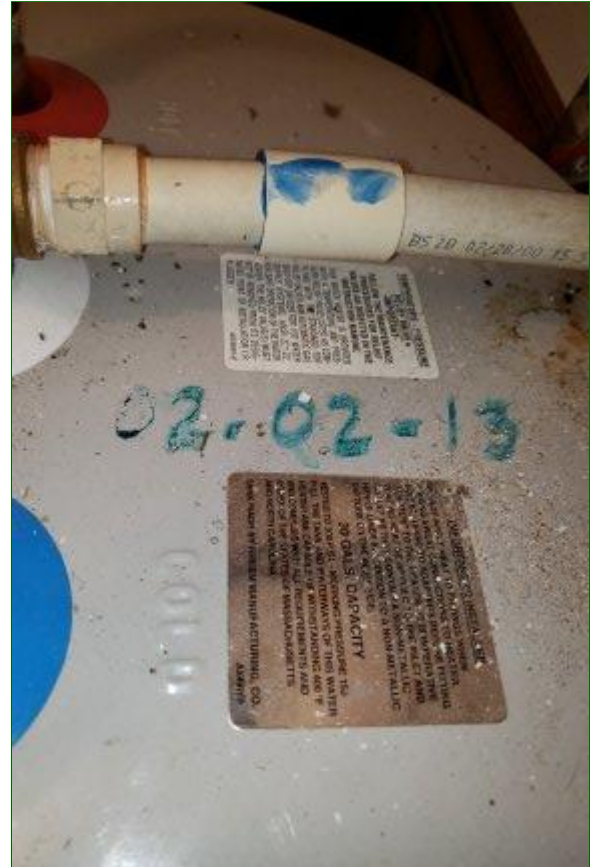
7.2 Item 2(Picture) Water heater installed in 2013
