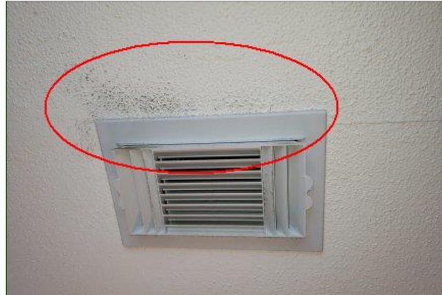
9.3 Item 1(Picture) Dirty vents
