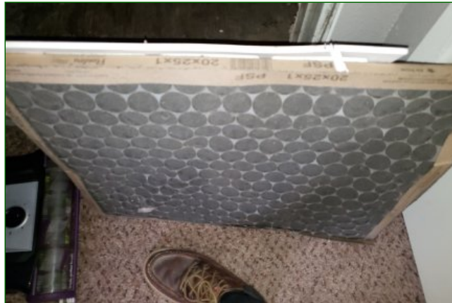
9.5 Item 21(Picture) Extremely dirty filter
