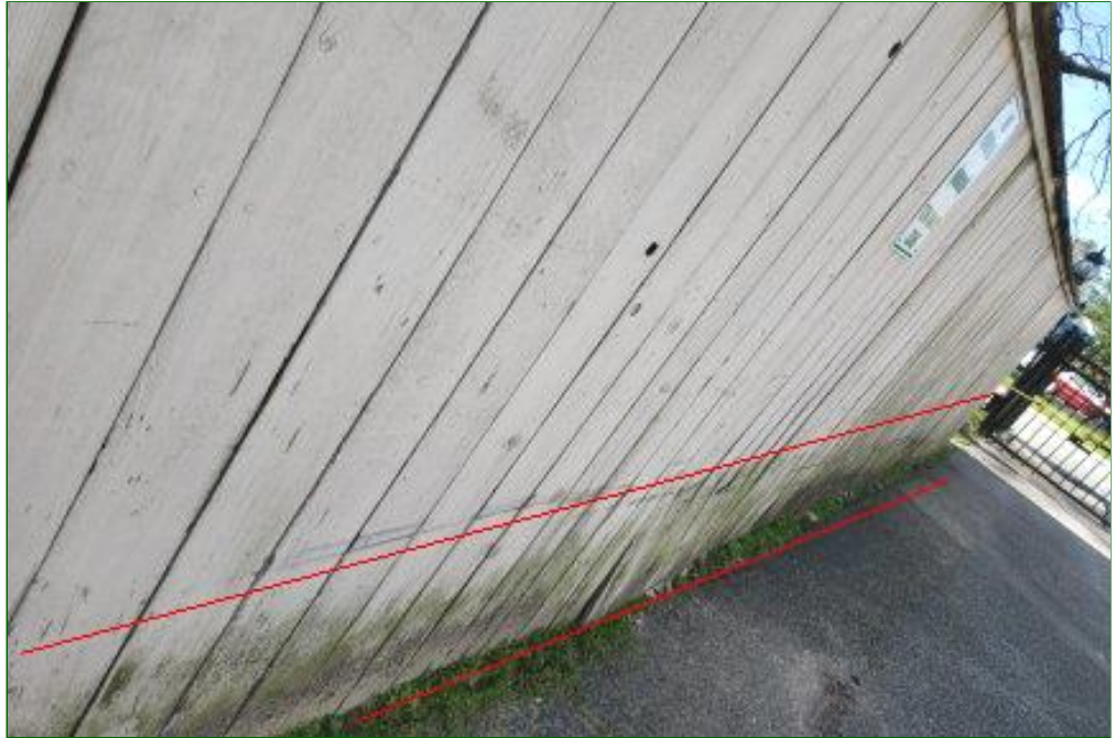
2.3 Item 1(Picture) Fencing at both units have microbic growth with a musty odor that is in need of cleaning
