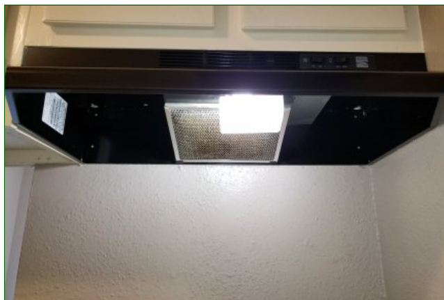
3.11 Item 2(Picture) Range hood exhaust system
