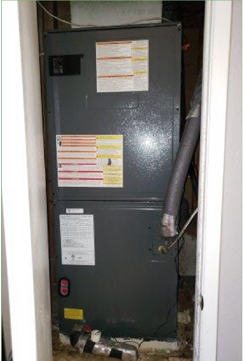
9.5 Item 15(Picture) Air handler
