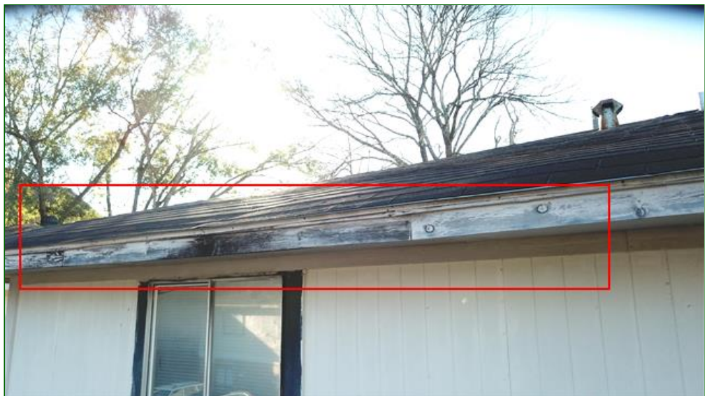
2.5 Item 8(Picture) Deteriorated soffit/fascia is in need of repair
