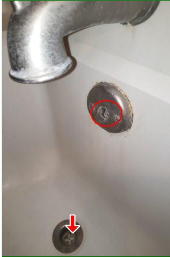
5.4.B Item 1(Picture) Damaged drain stop diverter is in need of repair.
