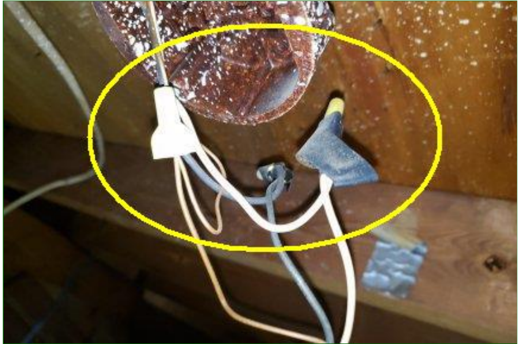
1.8 Item 1(Picture) Improper wire connections in attic of both units is in need of repair.
