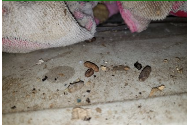
9.5 Item 4(Picture) Rodent droppings were discovered in Air handler closet
