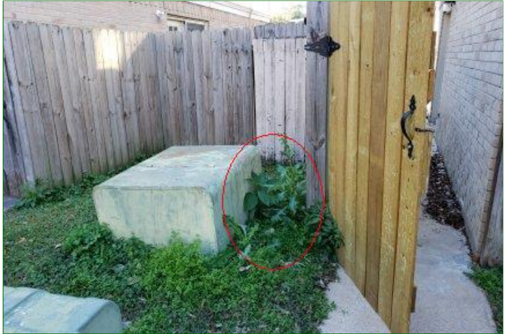
2.4 Item 6(Picture) Overgrown vegetation
