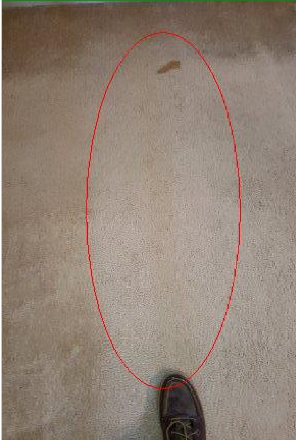
4.2 Item 9(Picture) uneven and creaking flooring on second floor
