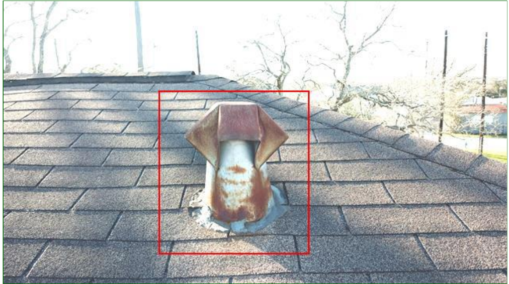
1.3 Item 1(Picture) Bonnet vents are improperly installed
