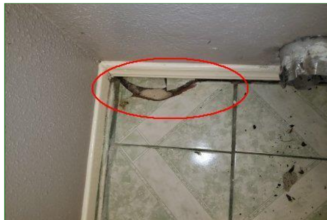
4.2 Item 6(Picture) Damaged tile
