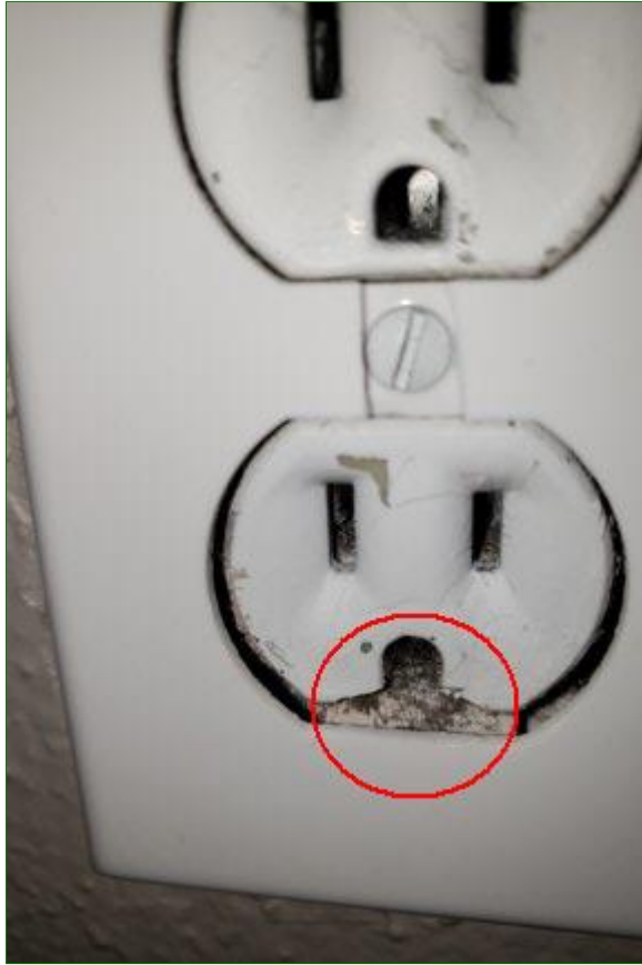
8.3 Item 3(Picture) Damaged receptacles
