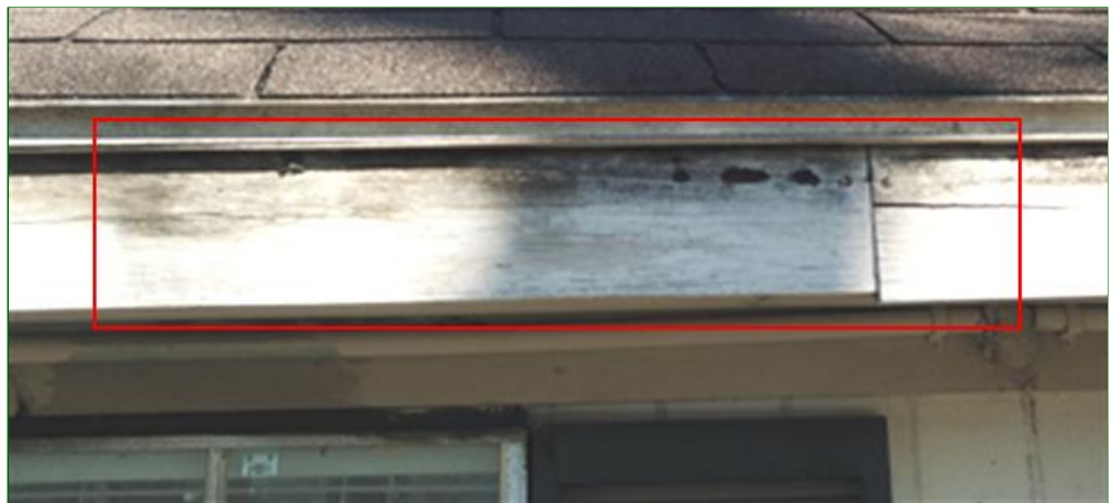
2.5 Item 6(Picture) Deteriorated soffit/fascia is in need of repair
