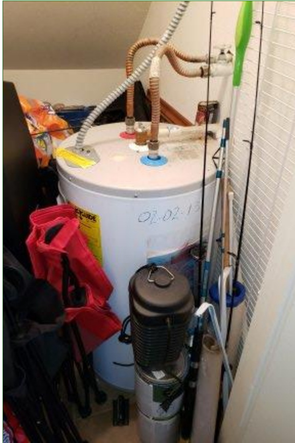
7.2 Item 1(Picture) Unit 1910 water heater
