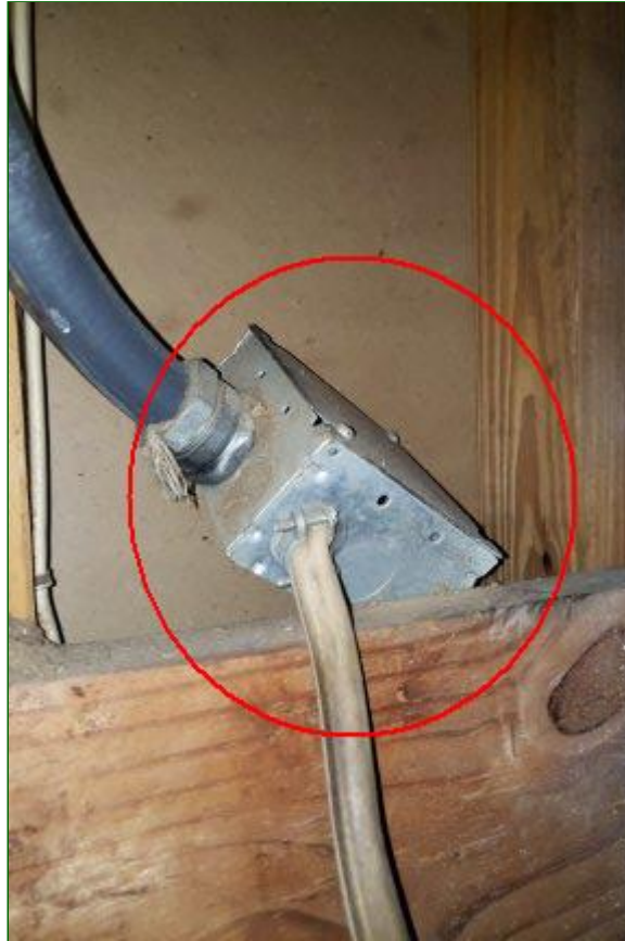
9.5 Item 8(Picture) Air handler power supply should be secured to structure and is in need of repair by a licensed electrician.
