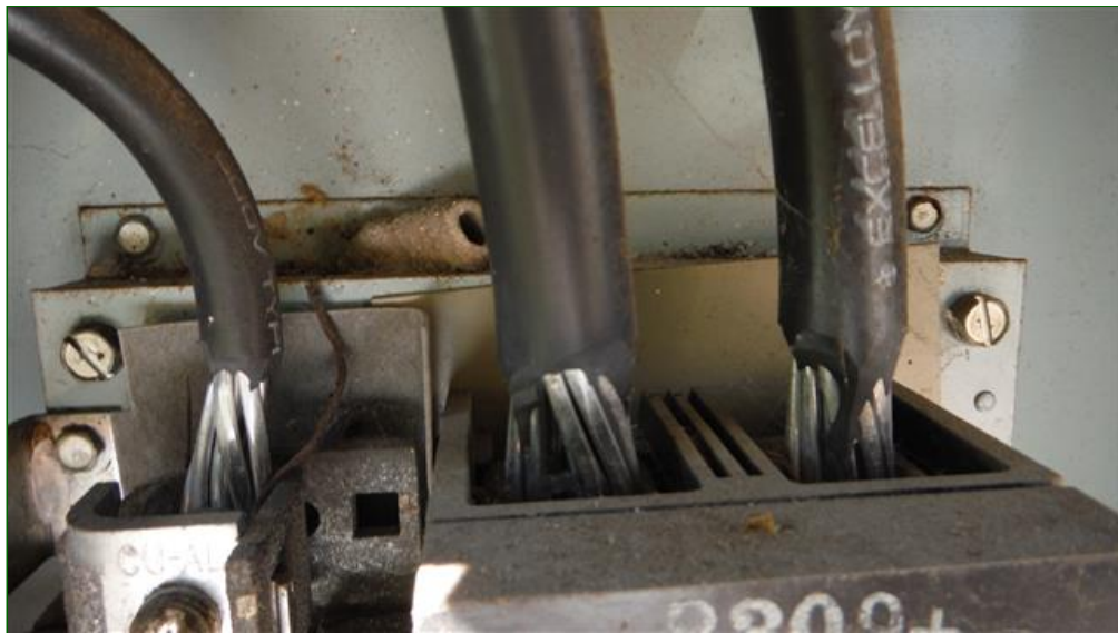
8.0 Item 2(Picture) Unit 1908 No visible dielectric grease on aluminum strand wiring should be corrected by a qualified contractor
