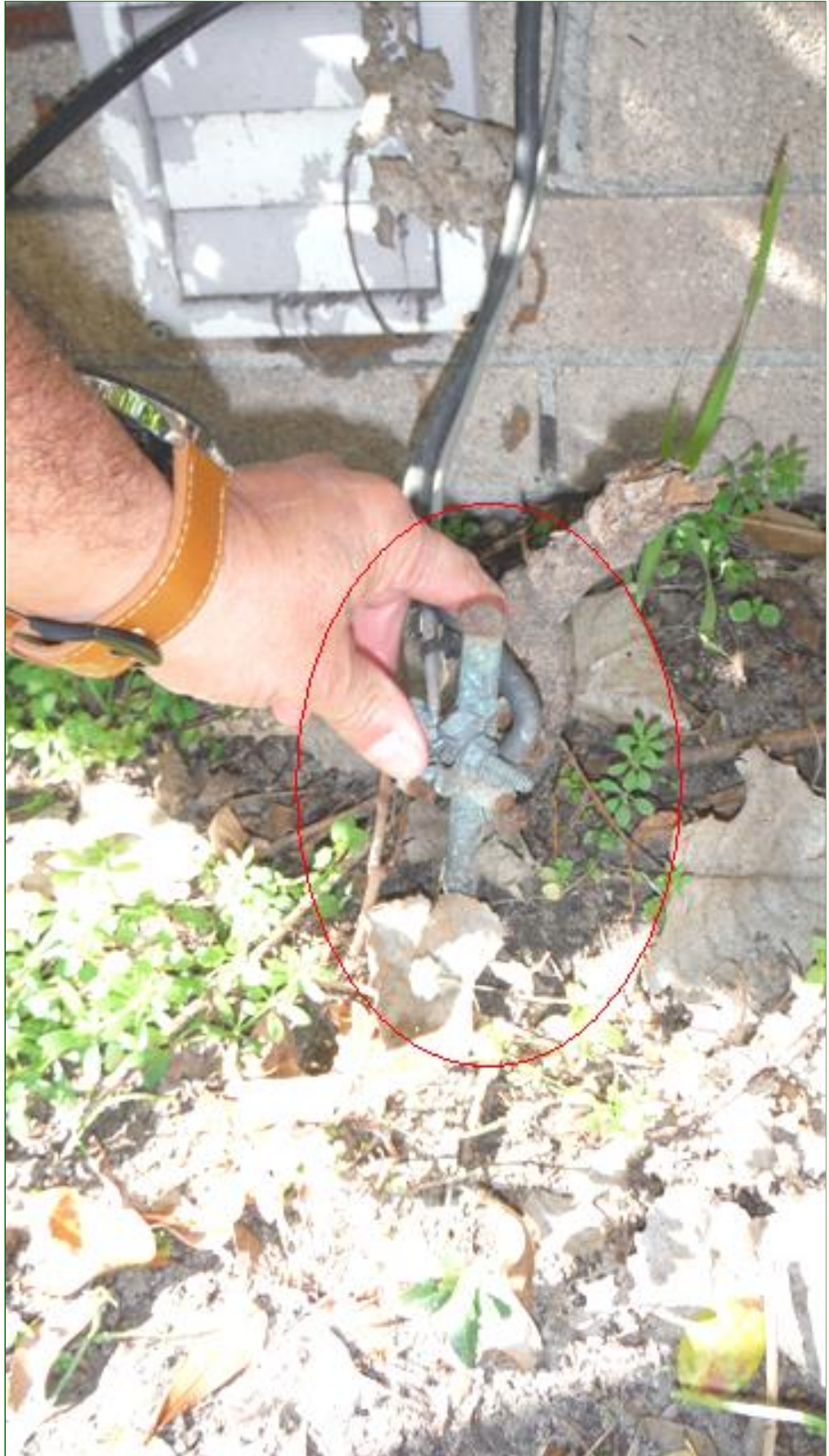
8.1 Item 2(Picture) Panel grounds to both panels are loose and in need of repair. Page 78 of 126
