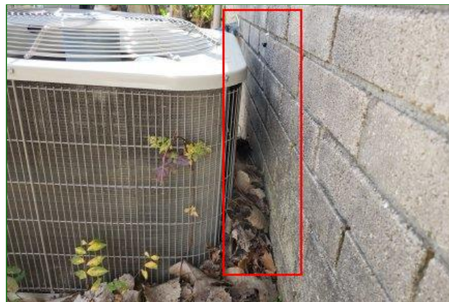
9.5 Item 18(Picture) Compressor should be installed 24 inches from wall as per manufacturers installation instructions.
