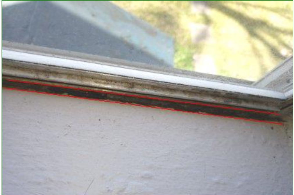
4.5 Item 1(Picture) Seal window sills
