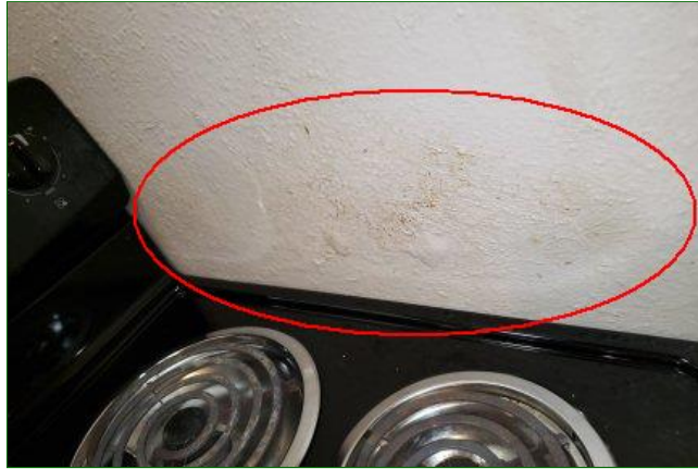
3.1 Item 1(Picture) Wall damage near range
