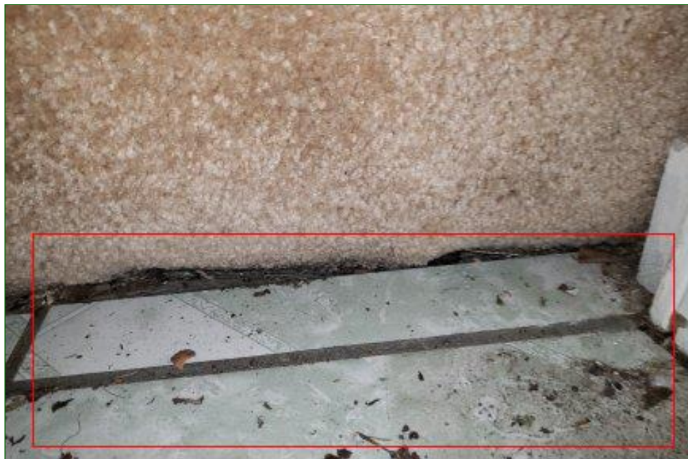
4.2 Item 3(Picture) Evidence of moisture entering front entry
