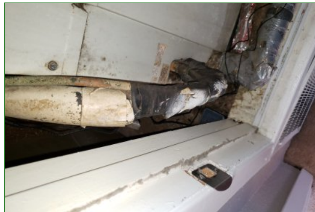
9.5 Item 7(Picture) Damaged insulation on cooling lines is in need of repair to prevent Cooling loss and condensation damage to materials
