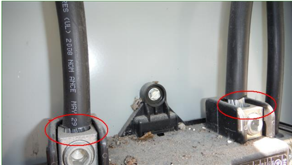
8.0 Item 1(Picture) Unit 1908 No visible dielectric grease on aluminum strand wiring should be corrected by a qualified contractor
