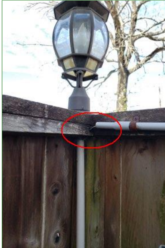
8.3 Item 1(Picture) Unit 1910 has improper electrical connections and are in need of repair.
