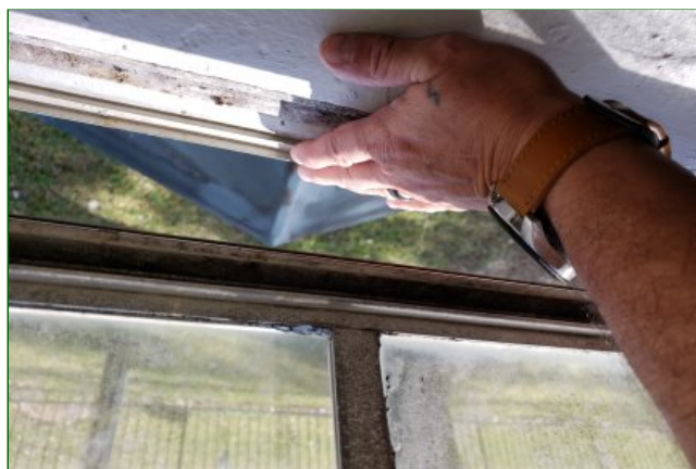
2.2 Item 1(Picture) Missing window screens throughout the units are in need of replacing
