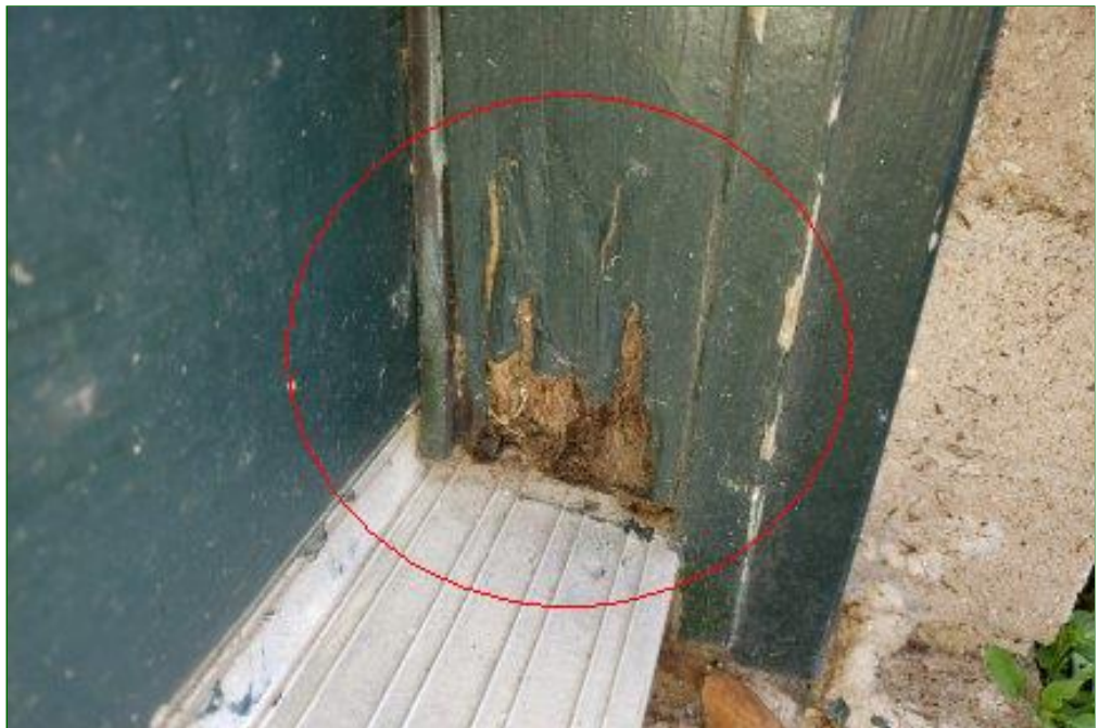
2.1 Item 2(Picture) Damaged/deteriorated door frame
