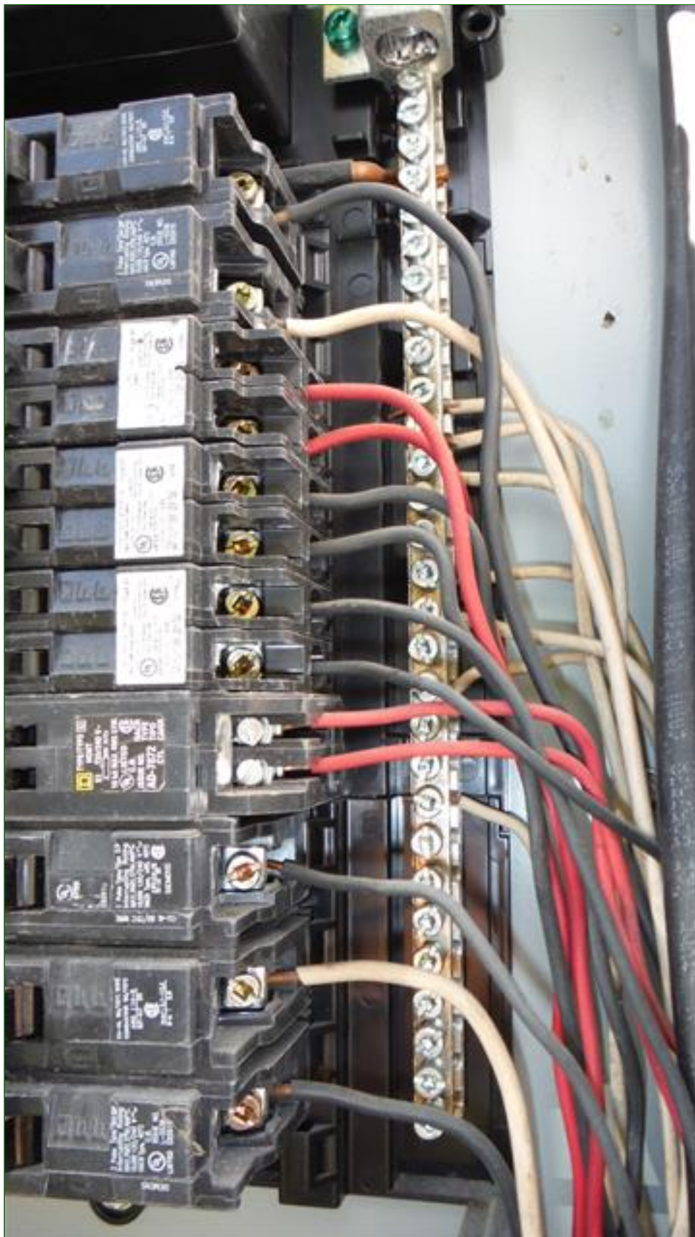
8.1 Item 7(Picture) 1908 circuit connections ok Page 83 of 126
