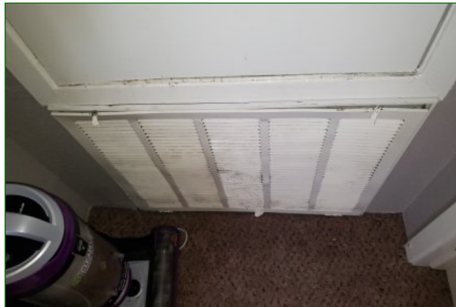
9.5 Item 22(Picture) Damaged filter grill is in need of repair
