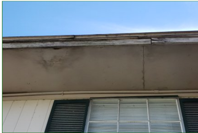
2.5 Item 2(Picture) Deteriorated soffit/fascia is in need of repair
