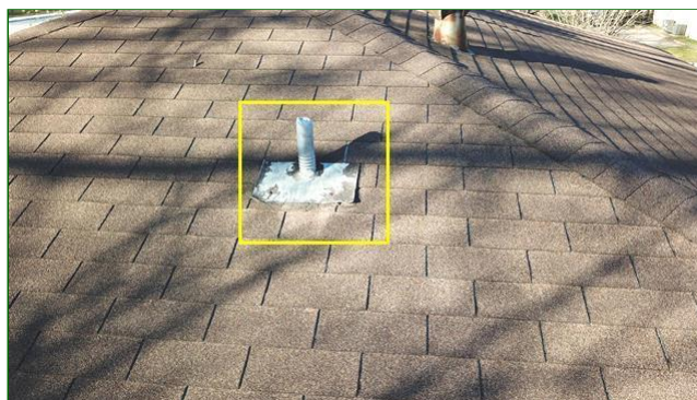
1.2 Item 2(Picture) Improperly installed vents
