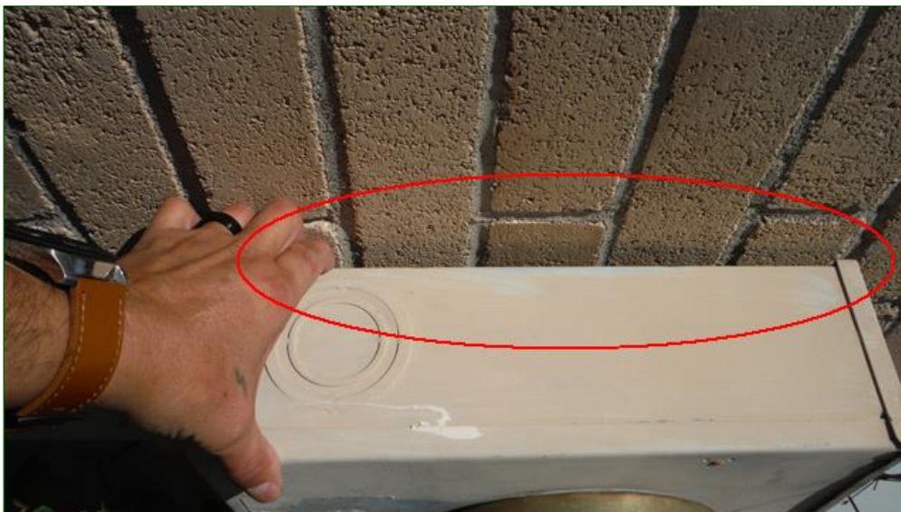
8.1 Item 22(Picture) Loose meter for 1910 is in need of repair.
