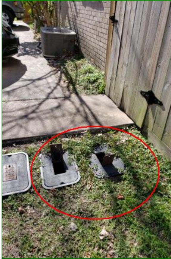
7.1 Item 1(Picture) Water meters located on right rear of building facing front
