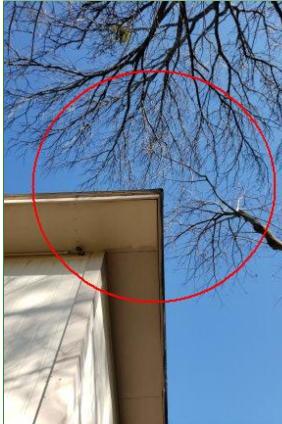
2.4 Item 4(Picture) Tree branches in need of trimming back from structure.
