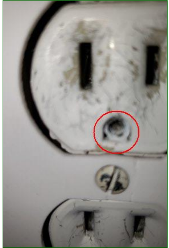
8.3 Item 4(Picture) Damaged receptacles
