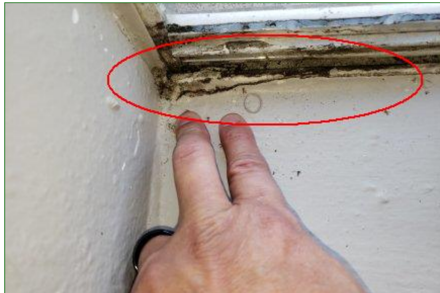
4.5 Item 2(Picture) Deteriorated window sill
