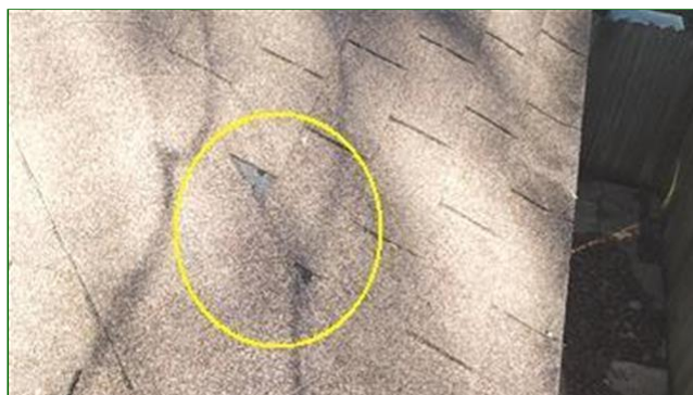
1.0 Item 10(Picture) Damaged shingles
