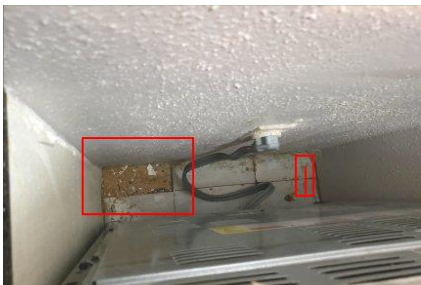
3.10 Item 6(Picture) Missing anti-tip bracket and missing floor covering
