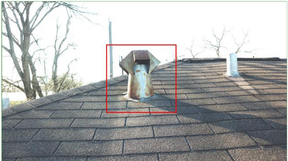
1.3 Item 2(Picture) Bonnet vents are improperly installed
