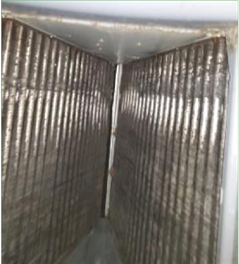
9.5 Item 17(Picture) Evaporator coils are not as bad as other unit but is in need of servicing.
