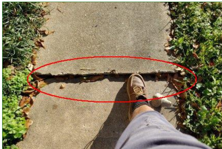
2.4 Item 5(Picture) Trip hazard in sidewalk at front of building is in need of repair.
