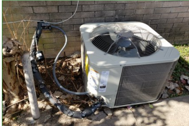
9.5 Item 13(Picture) Compressor should be installed 24 inches from wall as per manufacturers installation instructions
