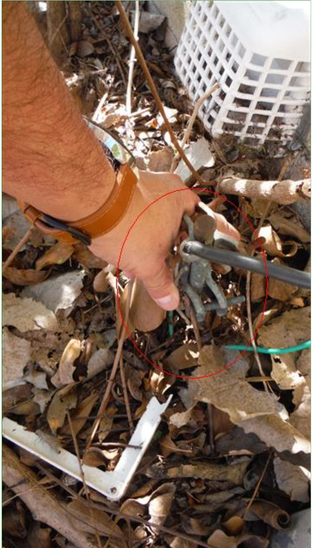
8.1 Item 12(Picture) 1910 panel ground loose and in need of repair. Page 88 of 126
