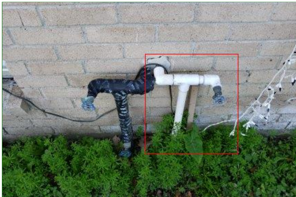
2.6 Item 2(Picture) Insulate all exterior water supply piping
