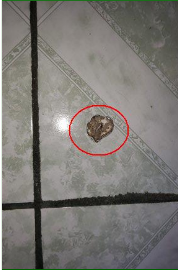
4.2 Item 5(Picture) Damaged floor tile
