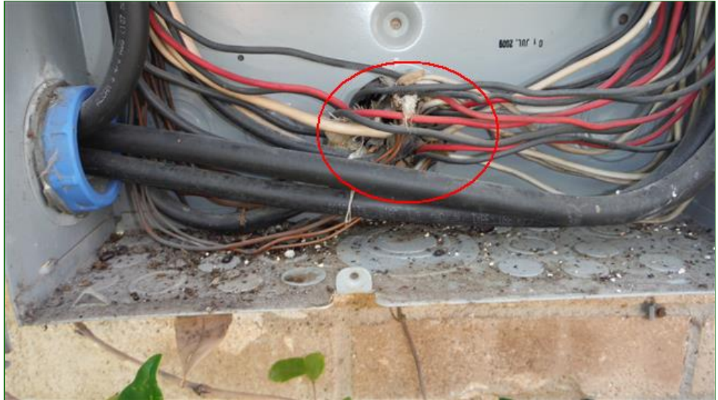
8.1 Item 8(Picture) 1908 Wire pass-through bushing is in need of repair
