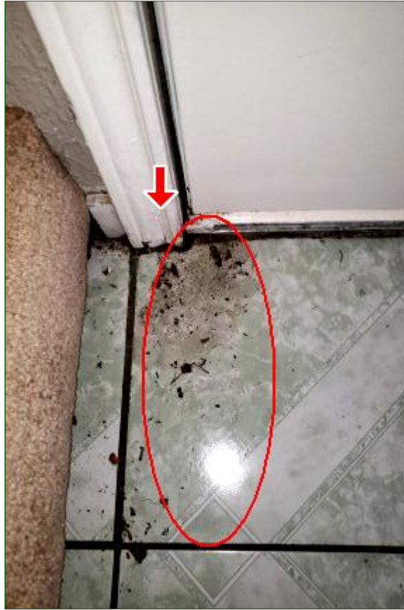
4.2 Item 2(Picture) Evidence of moisture entering front entry
