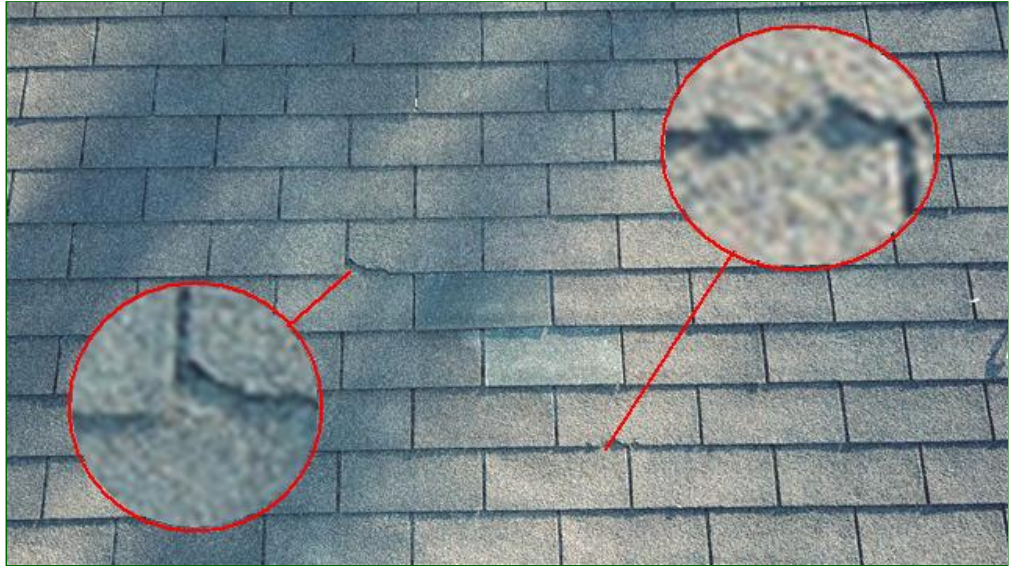
1.0 Item 3(Picture) Damaged shingles
