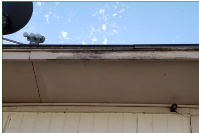
2.5 Item 3(Picture) Deteriorated soffit/fascia is in need of repair
