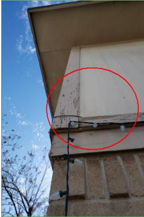
2.0 Item 1(Picture) Damaged/deteriorated siding/ trim
