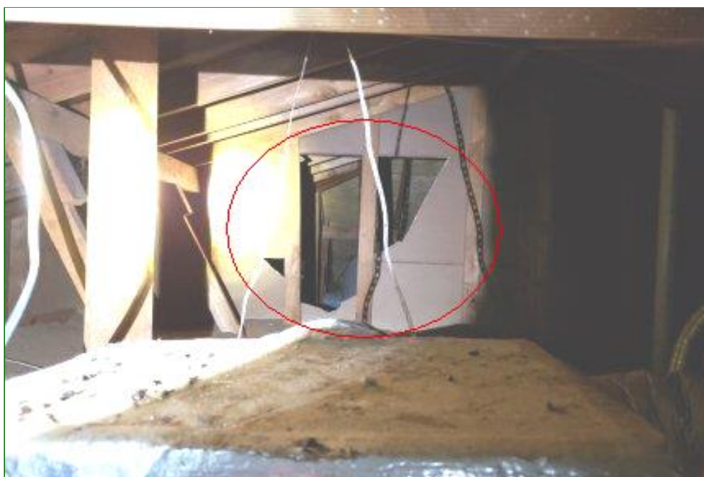
1.9 Item 2(Picture) Breach in firewall
