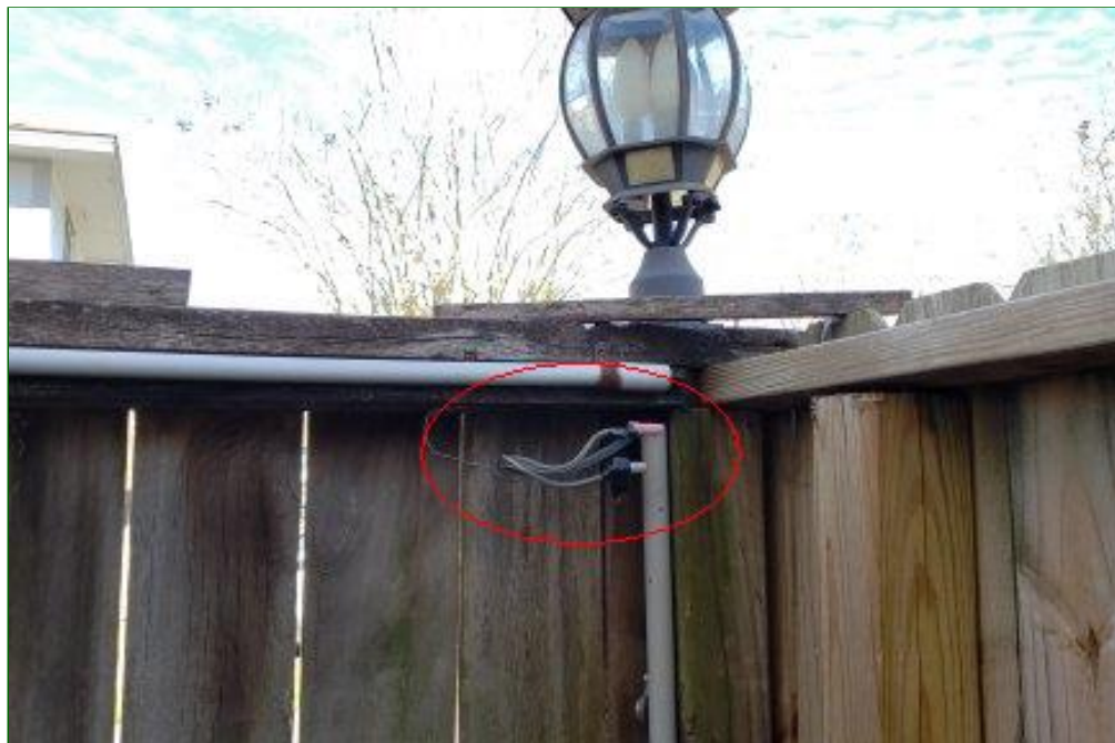
8.3 Item 2(Picture) Unit 1910 has improper electrical connections and are in need of repair.
