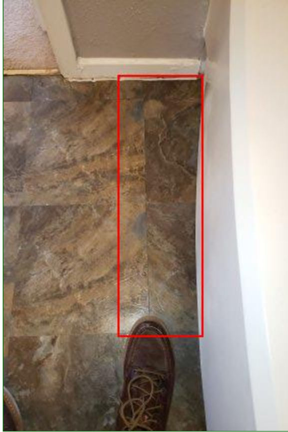
4.2 Item 1(Picture) Uneven flooring at tub
