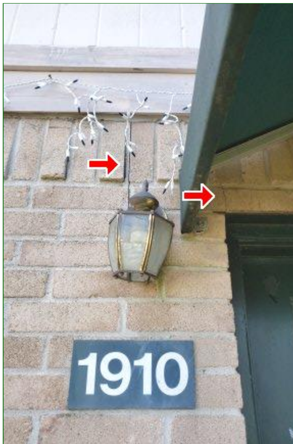
2.0 Item 5(Picture) Brick mortar cracks discovered on both units
