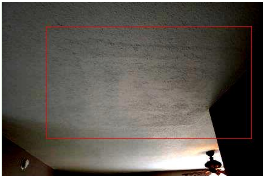
4.0 Item 6(Picture) Area below A/C unit in unit 1908 was dry at the time of inspection (2) Amateurish ceiling repairs discovered in both units are in need of repair by a drywall finisher
