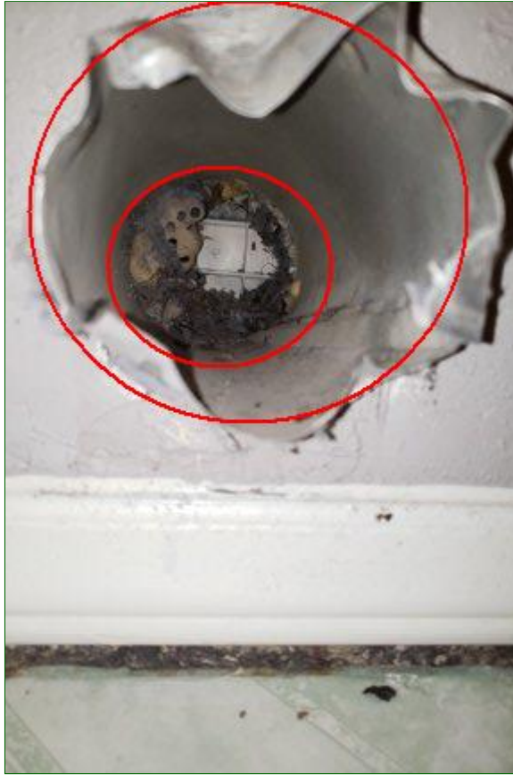
3.14 Item 2(Picture) Damaged dryer vent is in need of repair and cleaning
