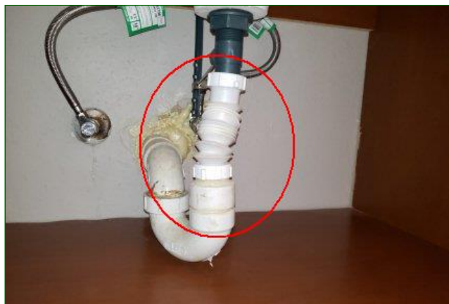
7.0 Item 1(Picture) accordion drain should be replaced by a qualified plumber
