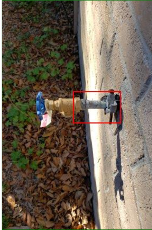
2.6 Item 3(Picture) Insulate all exterior water supply piping
