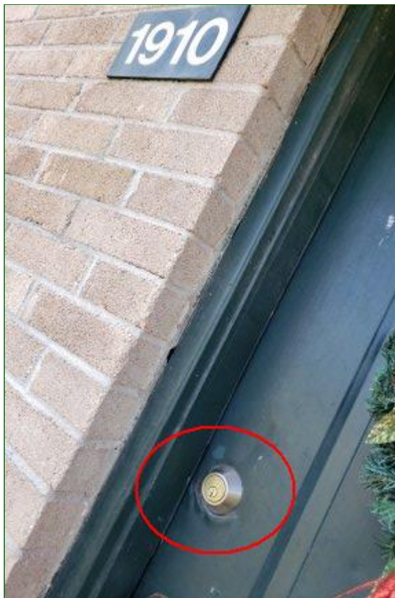
2.1 Item 4(Picture) Door damaged and in need of repair.
