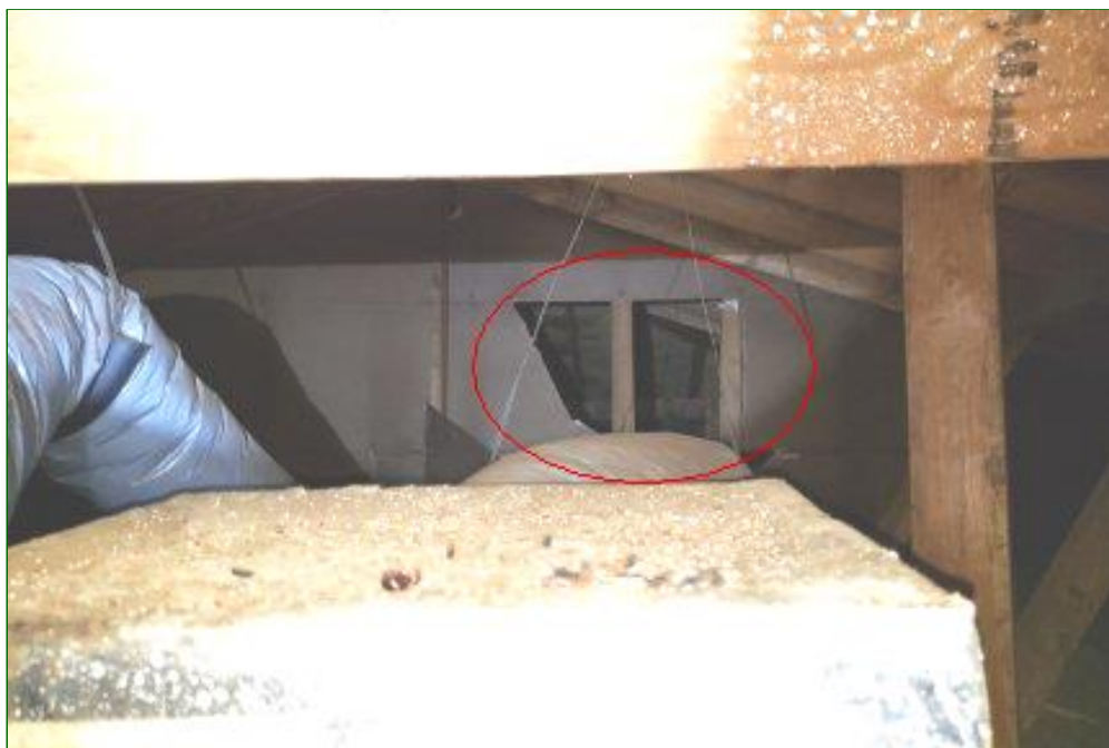
1.9 Item 1(Picture) Firewall damage between units
