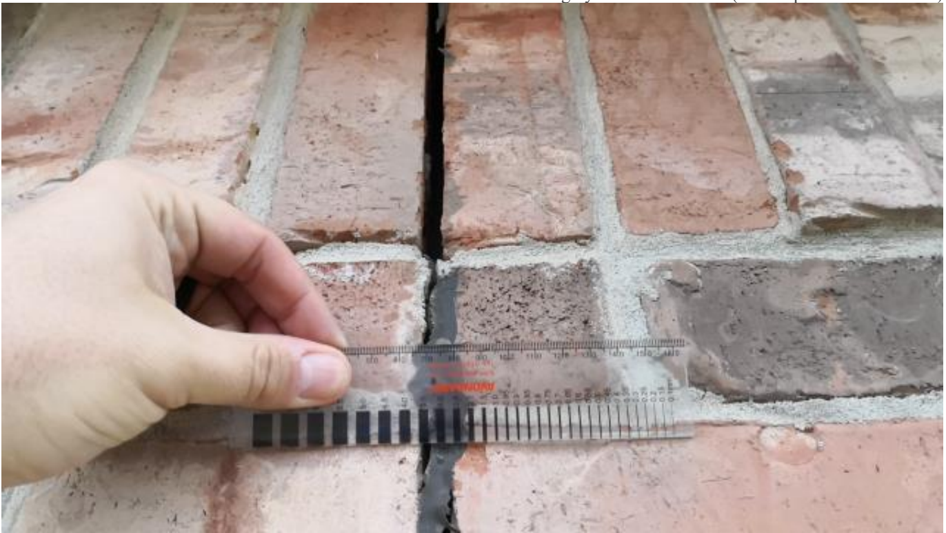
PIC 12 - Neighboring home has similar but not as pronounced defect in roughly the same location (not to open a can of worms)
