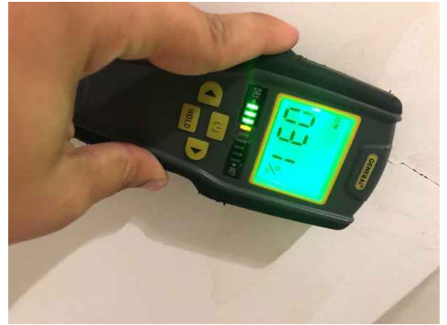
Stain in orange circle was wet at the time of inspection
