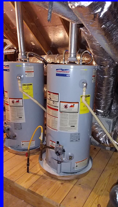
40 gallon water heaters attic
