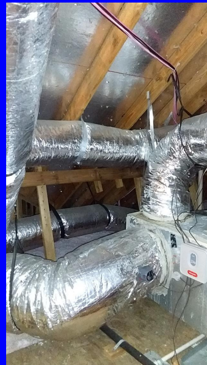
insulated ducts attic
