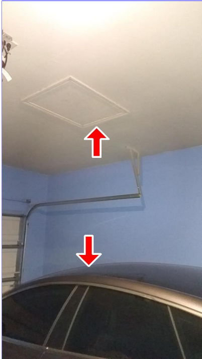
D. Item 1(Picture) unable to inspect garage attic
