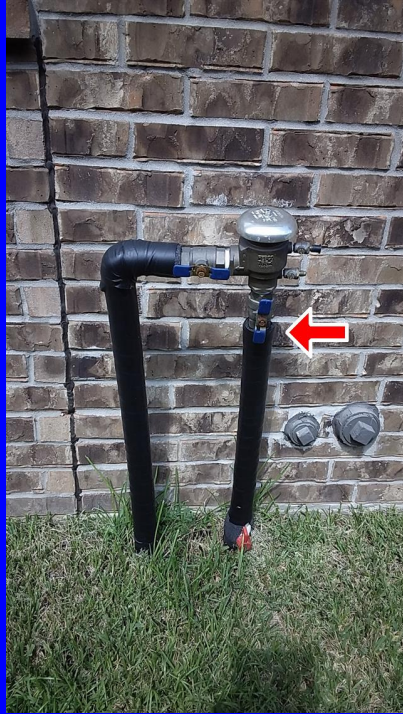
sprinkler shut off rear right
