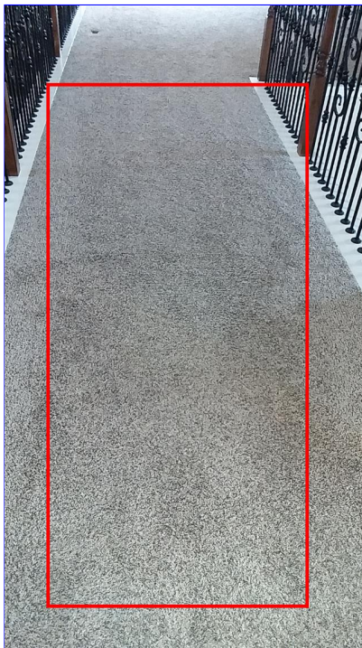
F. Item 2(Picture) multiple areas upstairs
