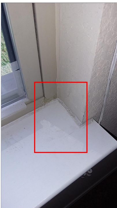
H. Item 3(Picture) primary bedroom
