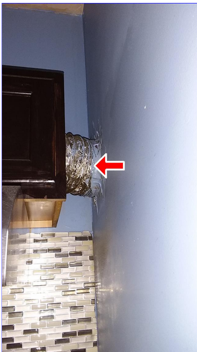
C. Item 2(Picture) incorrect vent pipe
