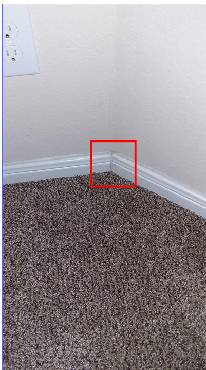
E. Item 14(Picture) multiple areas
