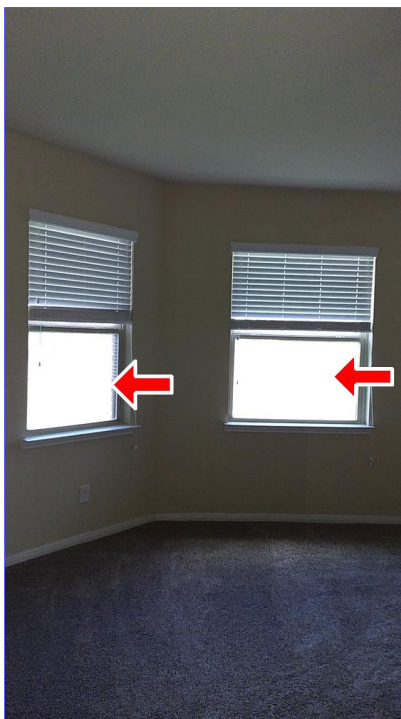
H. Item 8(Picture) primary bedroom
