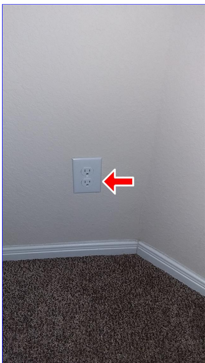
B. Item 6(Picture) multiple outlets interior
