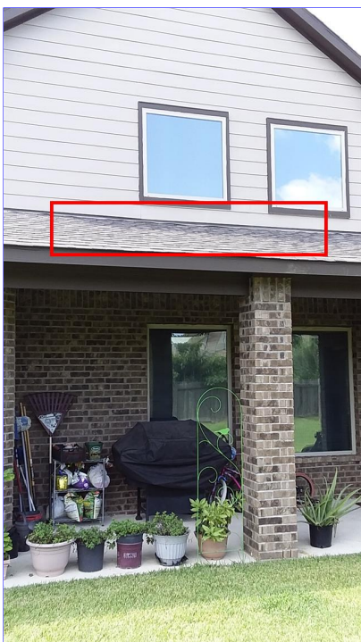
C. Item 5(Picture) rear
