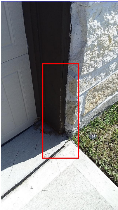
E. Item 4(Picture) multiple areas
