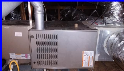
gas furnace attic
