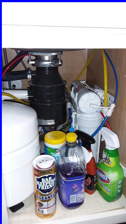
sediment filter kitchen sink
