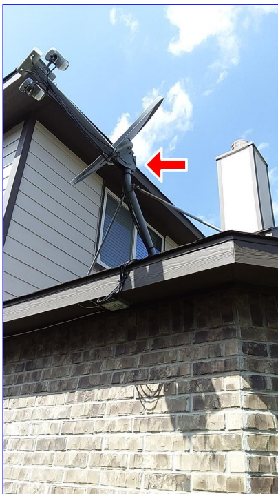
C. Item 4(Picture) rear
