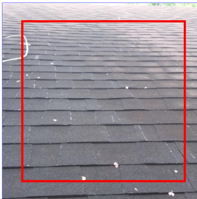
C. Item 6(Picture) Excessive wear
