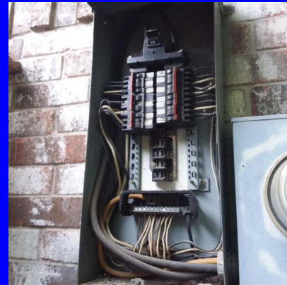
150 AMP main panel located at right side of home
