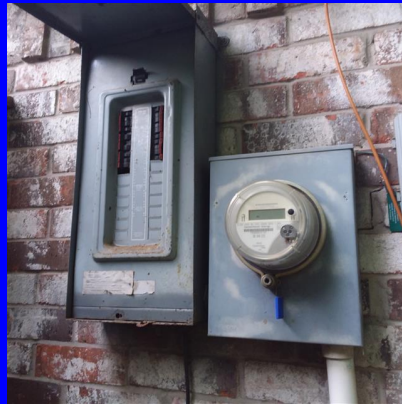
Below ground service located at right side of home
