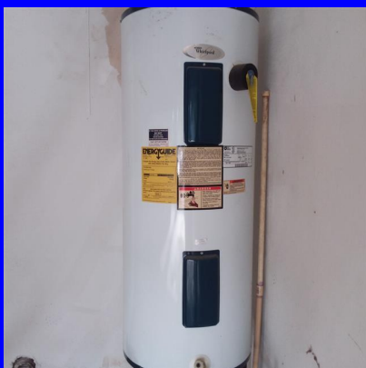
50 gallon electric water heater located in garage
