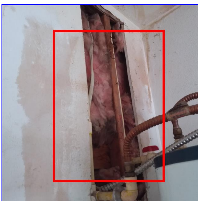
E. Item 36(Picture) Right rear of garage
