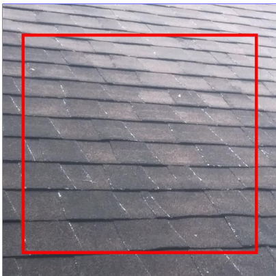
C. Item 5(Picture) Excessive wear
