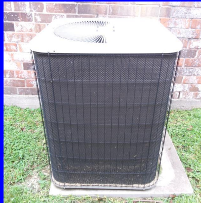
HVAC outside condenser
