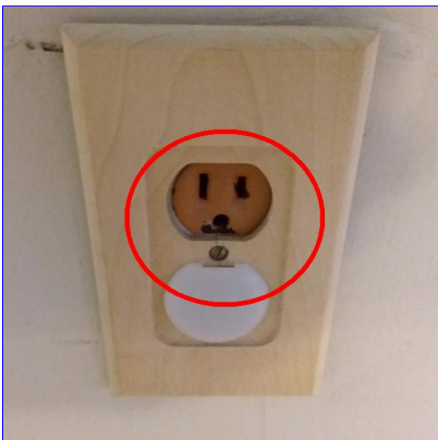
B. Item 12(Picture) Damaged outlets in multiple area's
