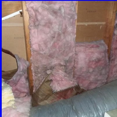
5 inches of batt insulation
