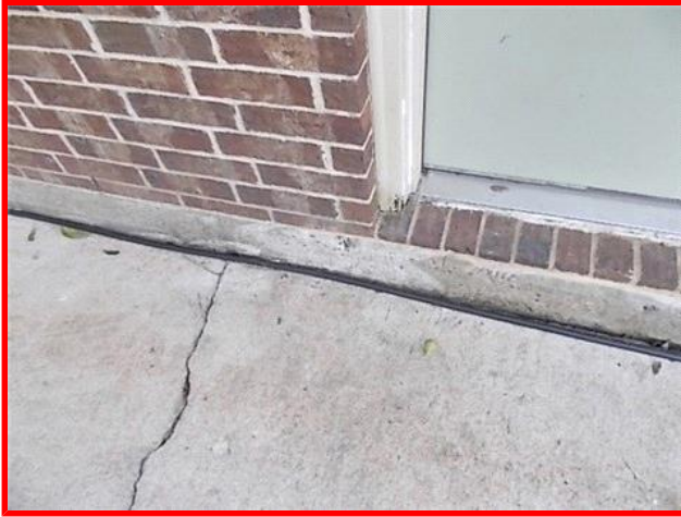
Rotted Trim at Rear Door & Crack in Rear Patio
