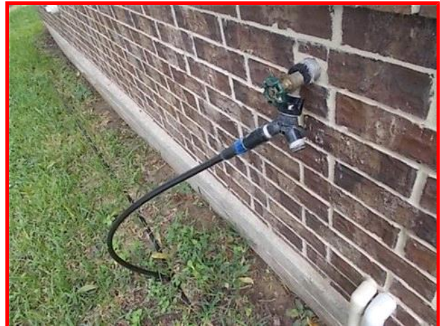
Missing Backflow Prevention at Hose Bib
