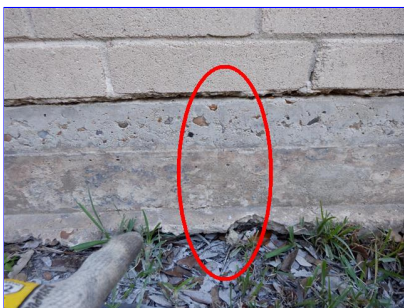
Right side foundation crack
