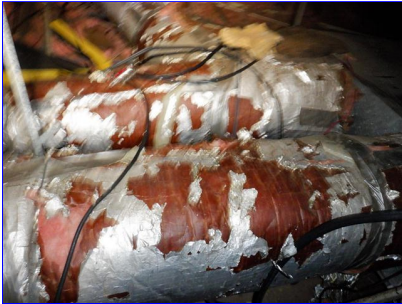
Attic duct lines
