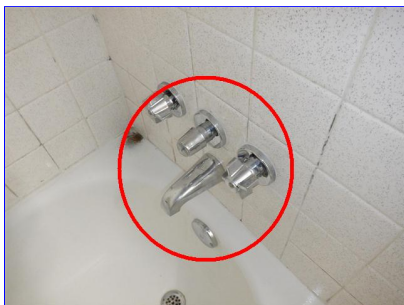
Full shower fixture bases
