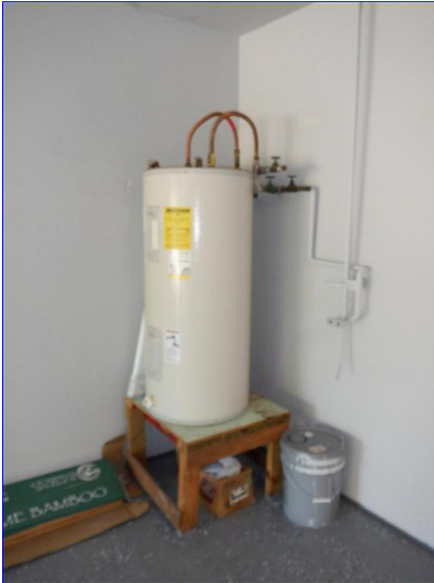
Garage WH unit
