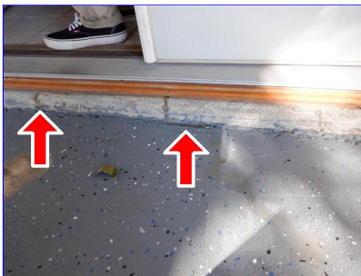
Water came from kitchen sink under tile out to the rear foundation
