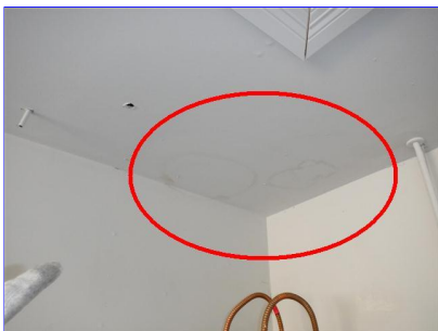
Garage ceiling stain
