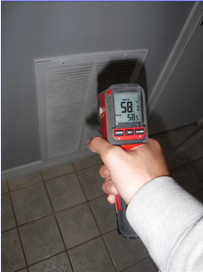
Hallway return air @58F
