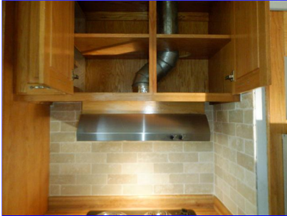
Kitchen exhaust vented to exterior
