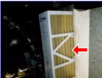
Attic air filter
