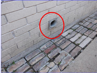
Dryer exterior vent
