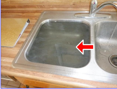
Kitchen sink piping clogged
