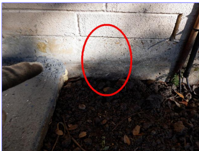
Rear foundation crack
