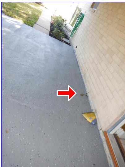
Water came out from within rear wall
