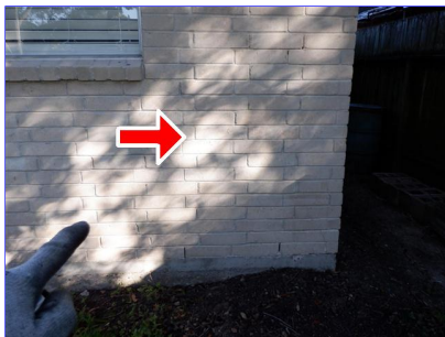
Rear brick wall crack
