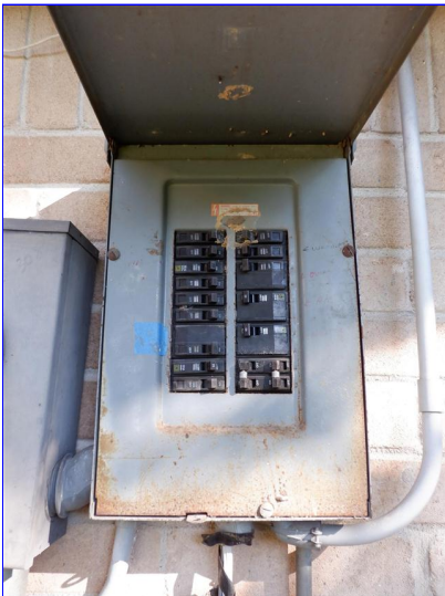
Square D, no main breaker, outside main elect panel
