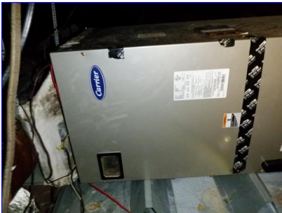
Attic furnace unit
