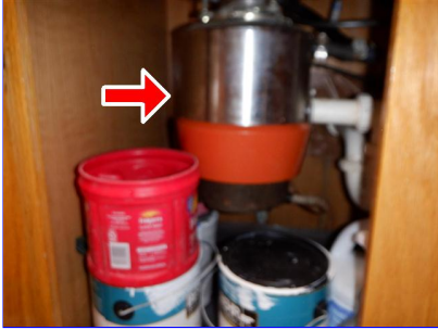
Kitchen disposal unit
