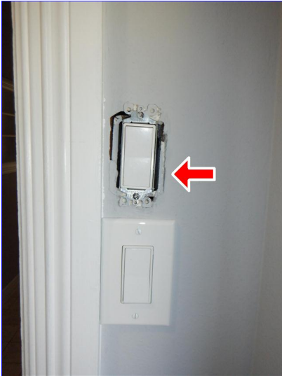
Bedroom lighting switch
