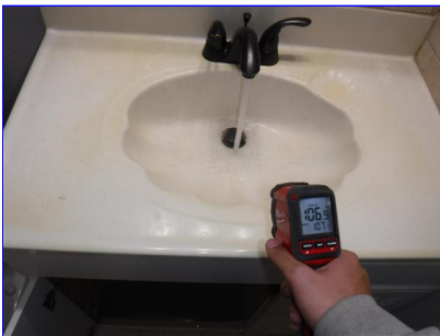
Hot water temperature @106F
