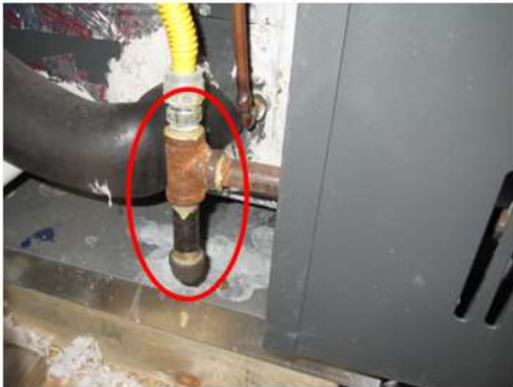
HEI file photo showing sediment trap
