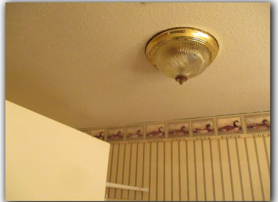
LIGHT FIXTURES TOO CLOSE TO BOTH BATH TUBS
