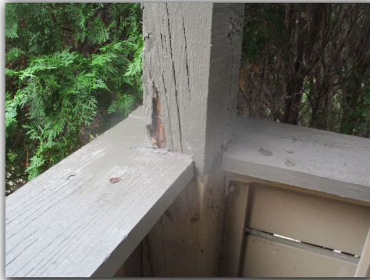
LITTLE WOOD ROT TO PATIO COLUMN
