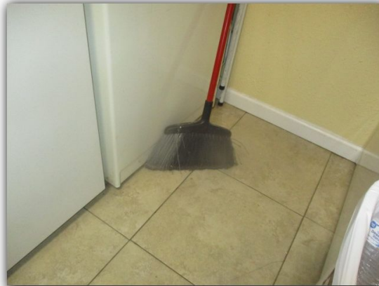
EMERGENCY DRAIN PAN AND DRAIN LINE MISSING FROM BENEATH WASHING MACHINE
