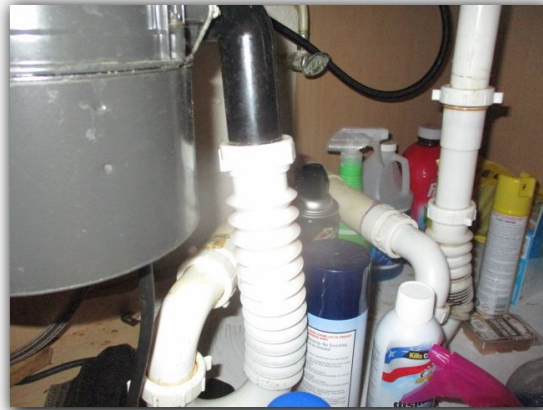
IMPROPER MATERIAL USED ON PARTS OF THE KITCHEN DRAIN LINES
