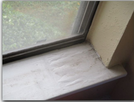
WATER PENETRATION TO GUEST BEDROOM WINDOW SILL
