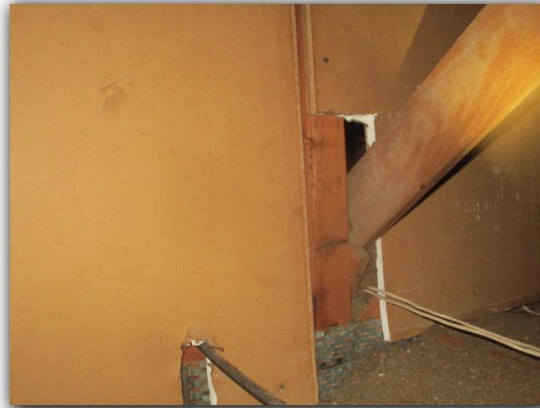
FIRE WALL NOT SEALED IN ATTIC
