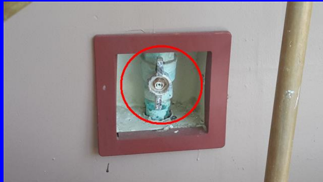
water shutoff inside garage right side
