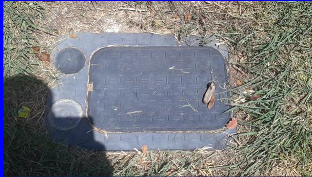
water meter front right of home
