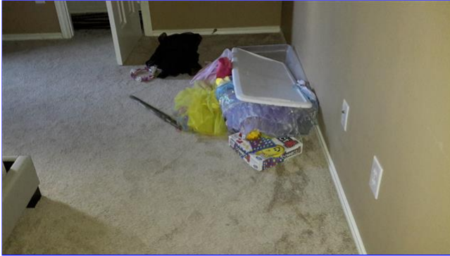
L. Item 14(Picture) front right bedroom
