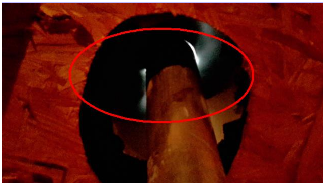
D. Item 1(Picture) water heater
