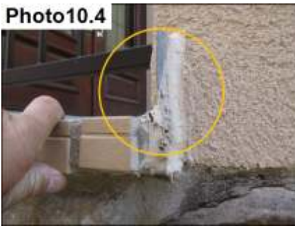
Porch Flashing Sealants/ Maintain
