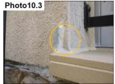
Porch Flashing Sealants/ Maintain
