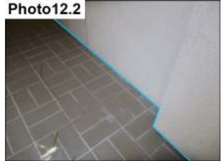
Stucco In Contact With Raised Flat Work/ Kant Bead Present/ Positive
