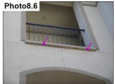
Rust Stains/ Clean And Paint
