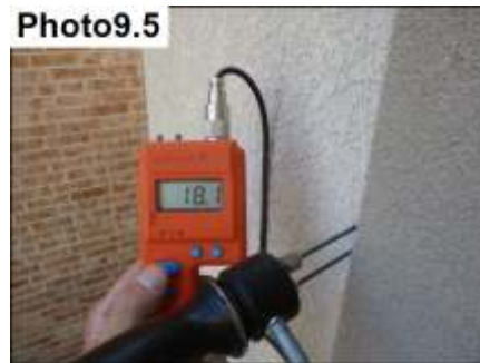
Moisture Probe/ Left Side Of Column Below Balcony
