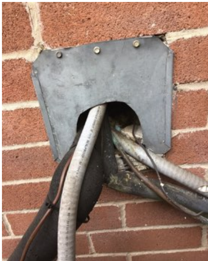
The area where the refrigerant lines enter the dwelling needs to be sealed to prevent insects and rodents from entering the premises
