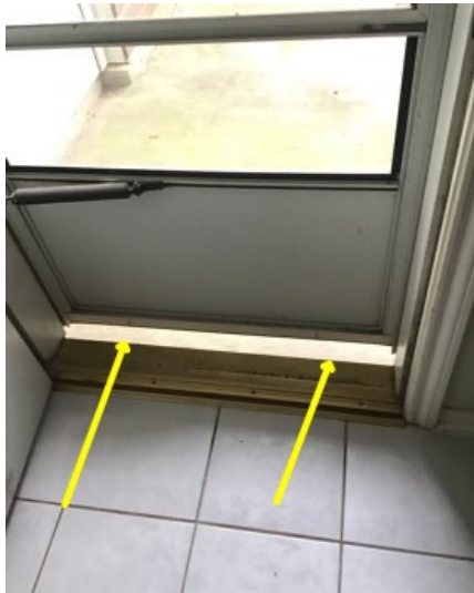
Screen door threshold missing
