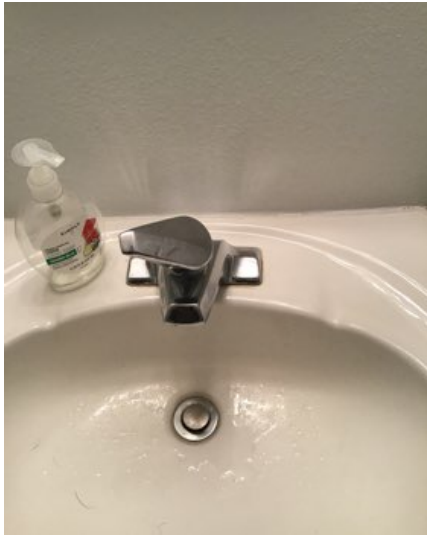
Cold side of faucet in downstairs guest bathroom does operate.
