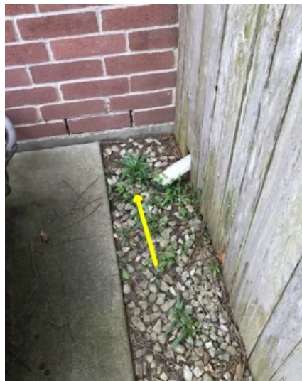
Splash pad missing
