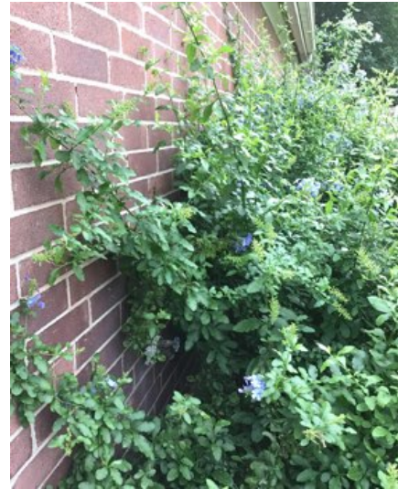
Shrubs are too close to the dwelling on the west side
