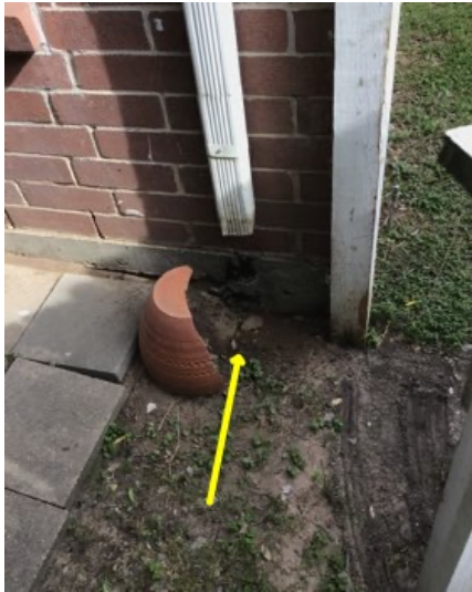
Splash pad is missing
