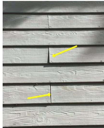
Siding on rear of dwelling needs to be caulked and re nailed on spots
