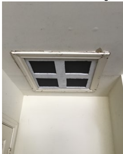
Garage ceiling has an opening which breaches the fire rated ceiling.
