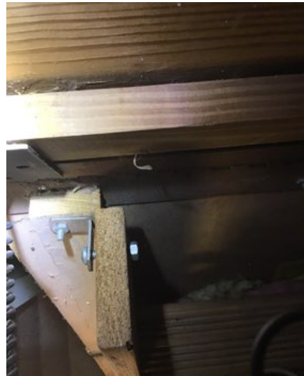
Attic access door photo shows screw and nut backing out. This could be a safety hazard
