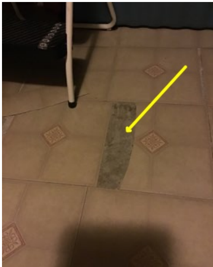
Flooring tile missing in master bedroom closet
