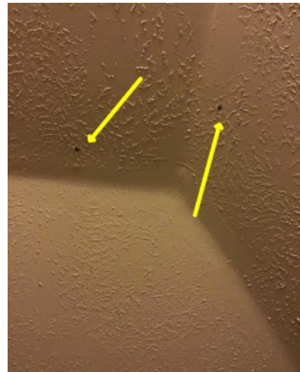
Ceiling nail pops in master bedroom closet
