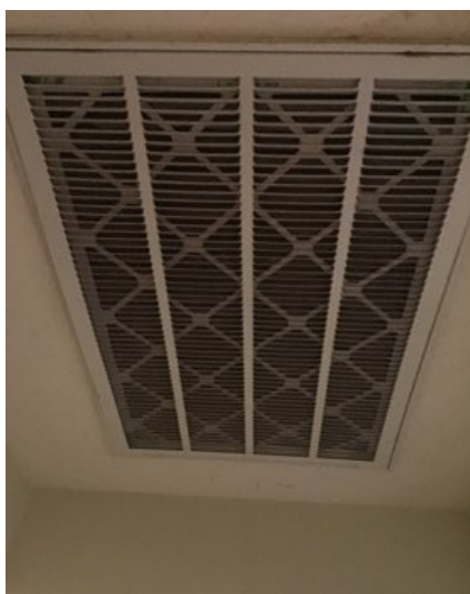
Air filter is dirty downstairs
