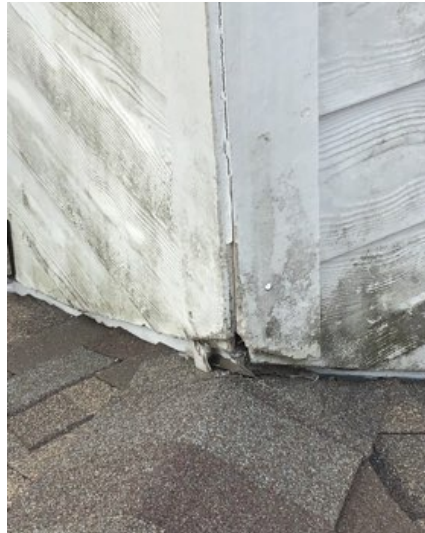
Chimney needs attention
