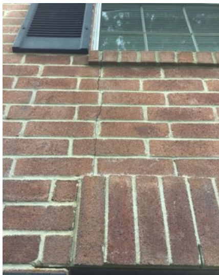
Crack in brick veneer on north side front of dwelling This is normal settlement for a home this age
