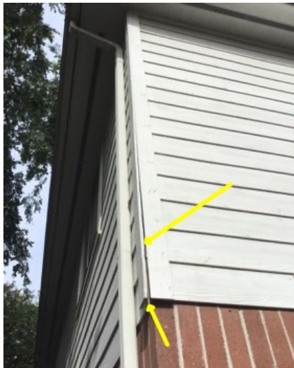
Trim board on east side rear needs to be repaired
