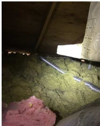
Bath fan is vented to the soffit
