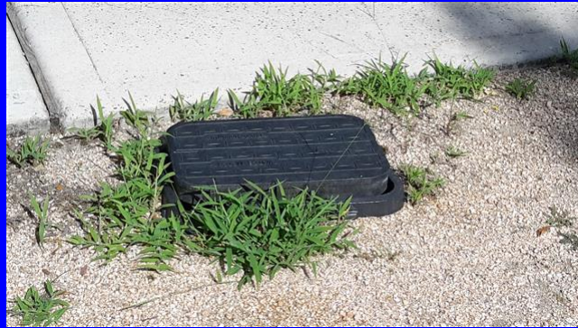
Water meter located at the street
