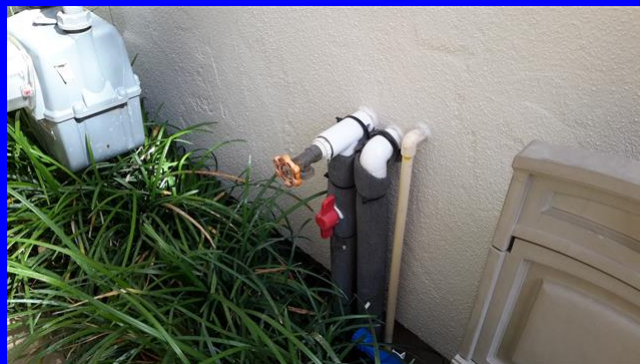
Main water shutoff valve located on the left side of the home
