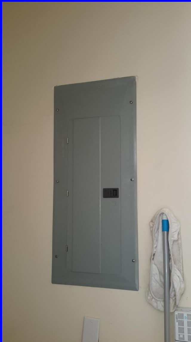
Electrical panel located inside the garage on the left wall
