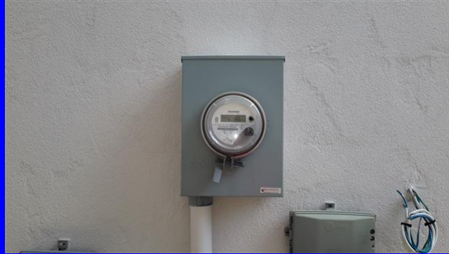
Underground electrical service entrance located on the left side of the home
