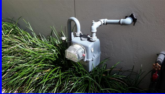
Gas meter located on the left side of the home
