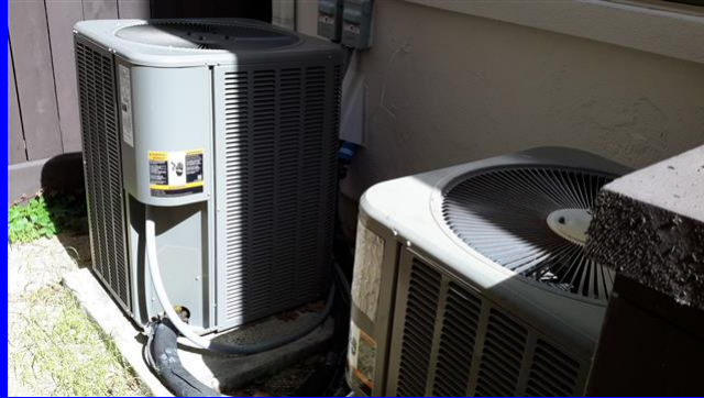
Two Lennox condensing units located on the left side of the home
