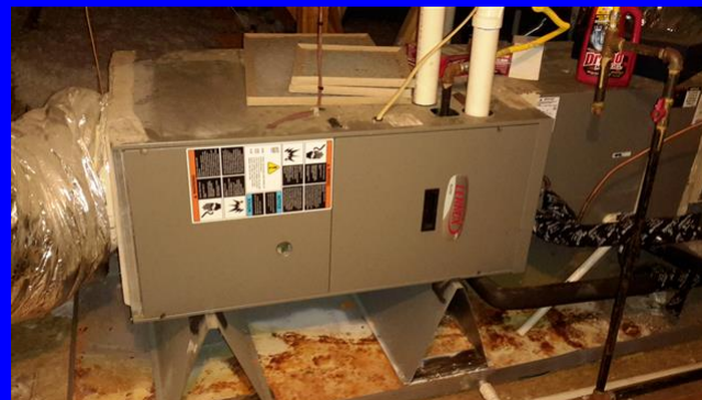
Lennox gas furnace located in the front of the attic. Heats and cools the 3rd floor
