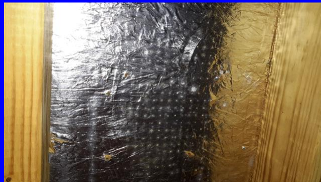
Radiant Barrier installed in the attic
