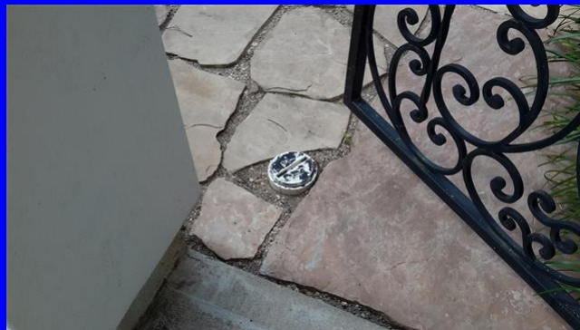
Sewer clean out located at the front gate
