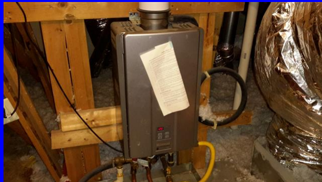
Rinnai tankless water heater located in the attic
