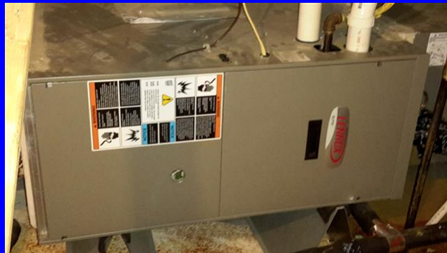
Lennox gas furnace located in the rear of the attic. Heats and cools the 1st and 2nd floor
