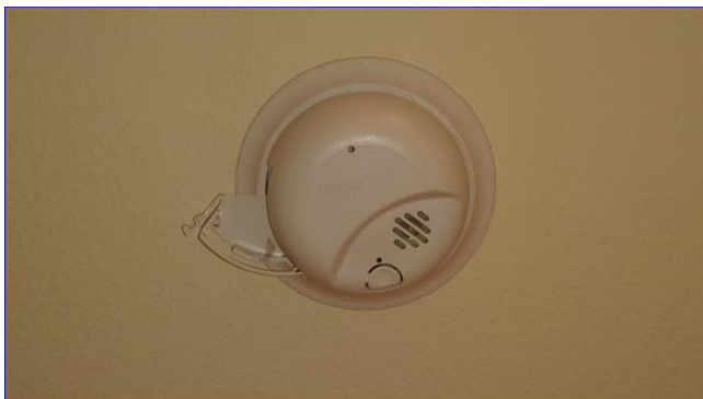
B. Item 1(Picture) battery missing. 3rd floor outside bedrooms
