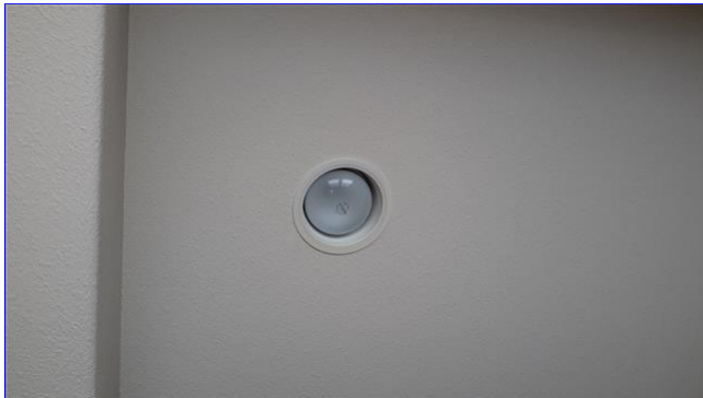
B. Item 4(Picture) front left corner of master bedroom ceiling
