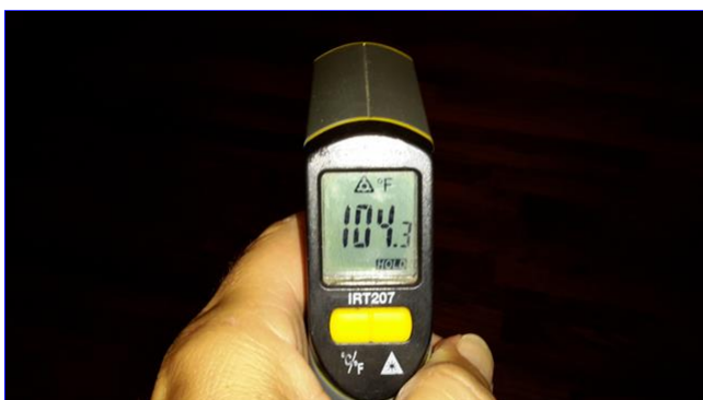
A. Item 2(Picture) kitchen vent temperature in heat mode
