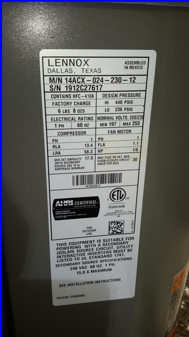
Front condensing unit label
