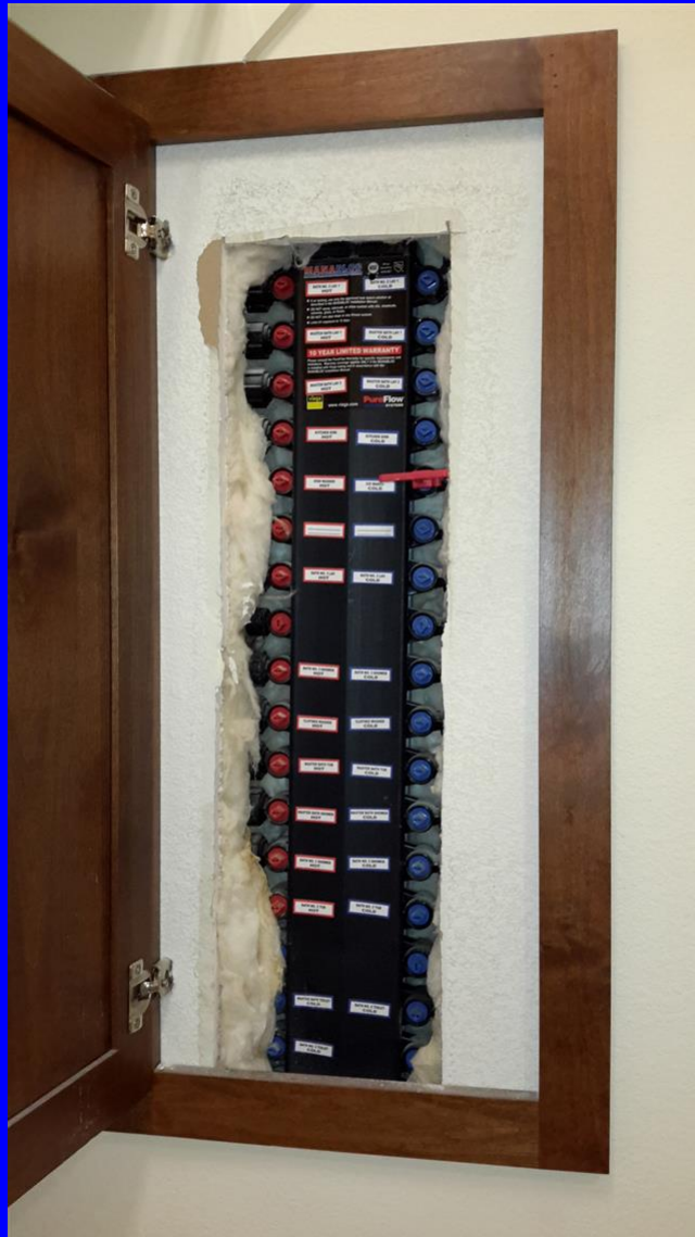
PEX water distribution manifold located in the laundry room
