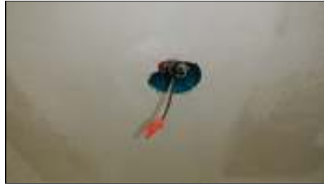
Open junction boxes located in the garage/shop should be properly enclosed.
