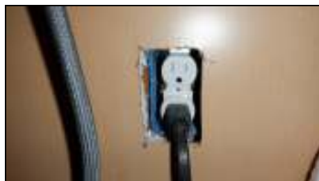
Missing outlet cover plates in the kitchen sink cabinet should be replaced.
