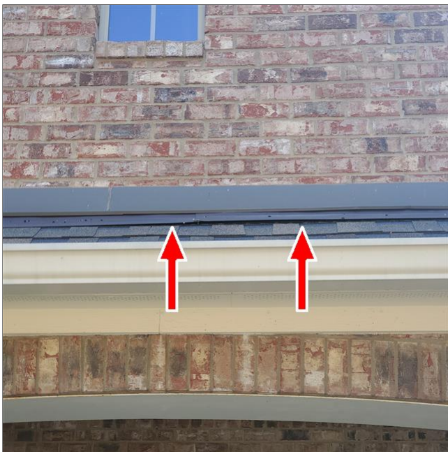
C. Item 4(Picture) Lifted flashing.
