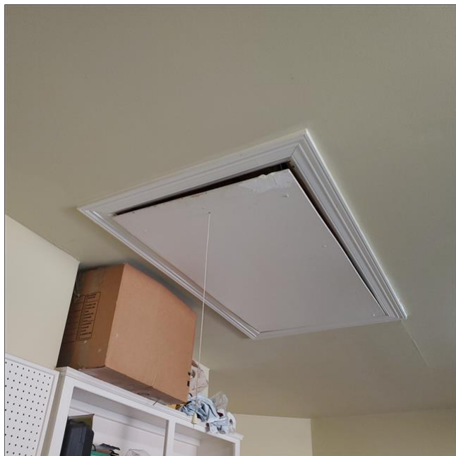
D. Item 1(Picture) Pull down not sealing.
