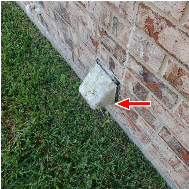
H. Item 1(Picture) Wall cap was loose.
