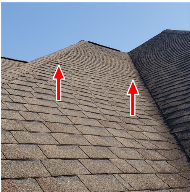
C. Item 6(Picture) Lifted shingles at the right slope.
