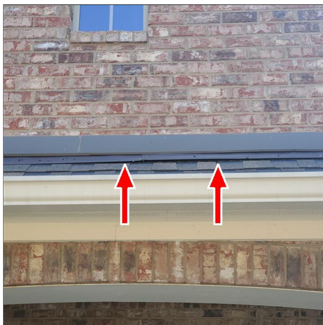
C. Item 4(Picture) Lifted flashing.
