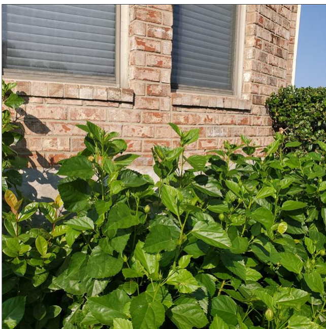
E. Item 2(Picture) Overgrown vegetation against the home at the back.
