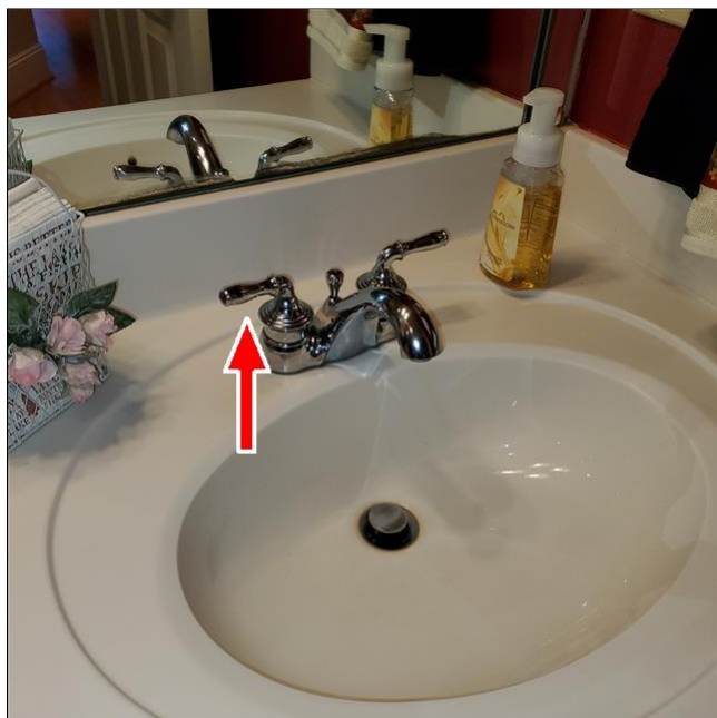
A. Item 1(Picture) Valve handle was difficult to turn.
