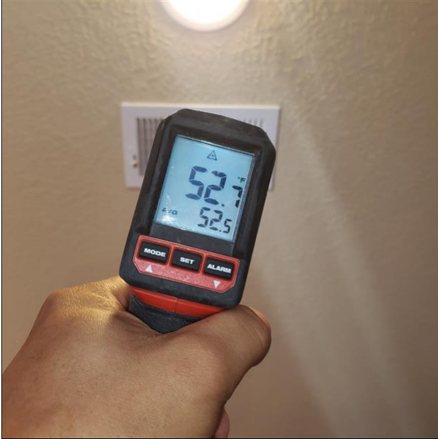
B. Item 5(Picture) 52.7 degree supply air.
