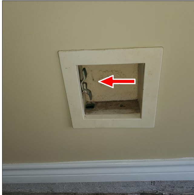
Main water valve in the garage.
