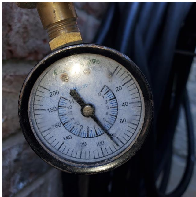
Water pressure was 84 psi (slightly high)
