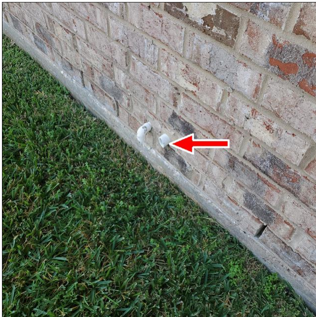
C. Item 2(Picture) Turndown was broken off.
