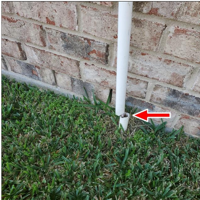
A. Item 3(Picture) Conduit was damaged.
