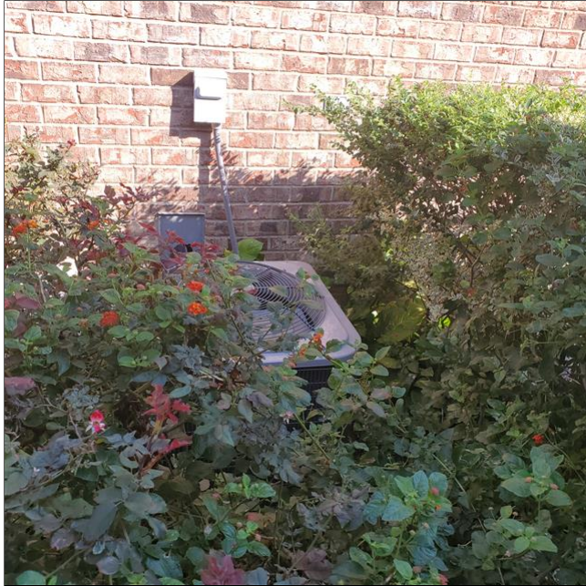
B. Item 2(Picture) Lots of vegetation growth around unit.
