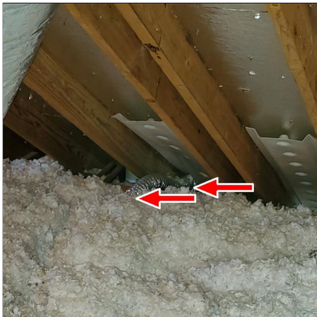
F. Item 1(Picture) Ducts terminate at soffit.
