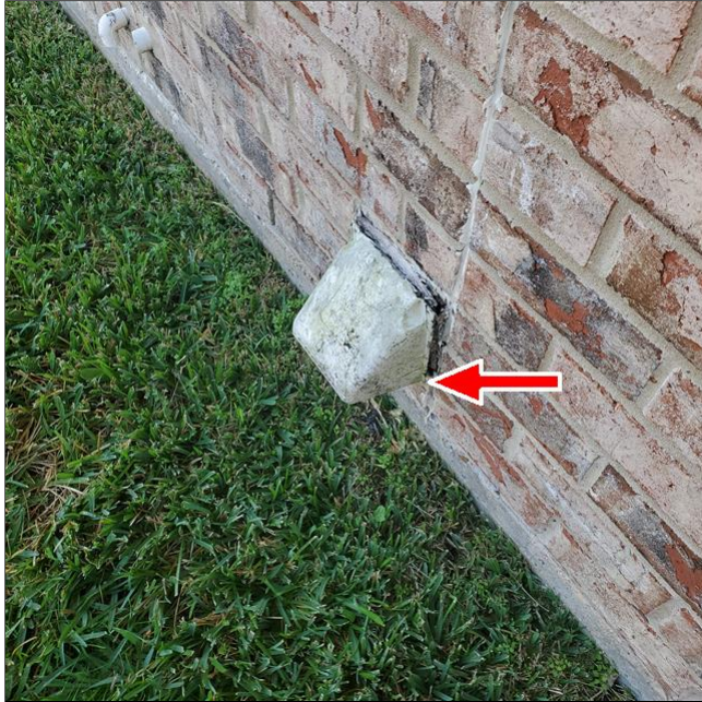
H. Item 1(Picture) Wall cap was loose.
