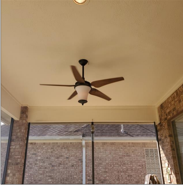
B. Item 1(Picture) Ceiling fan was wobbling.
