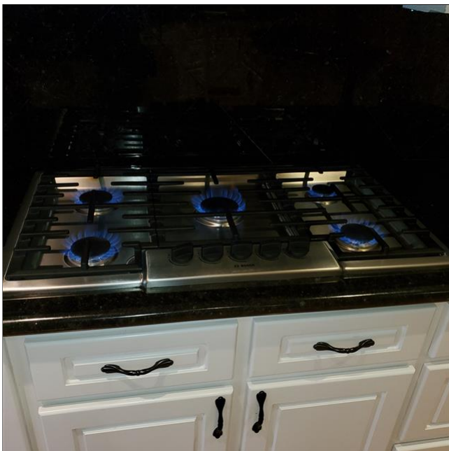
D. Item 1(Picture) Gas burners working.
