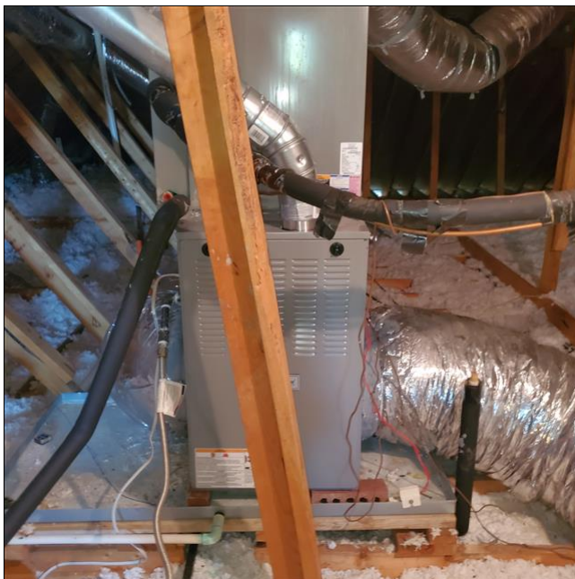
A. Item 1(Picture) Overview of heating system.
