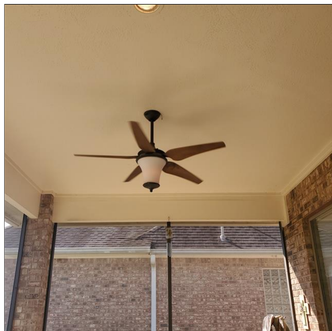
B. Item 1(Picture) Ceiling fan was wobbling.
