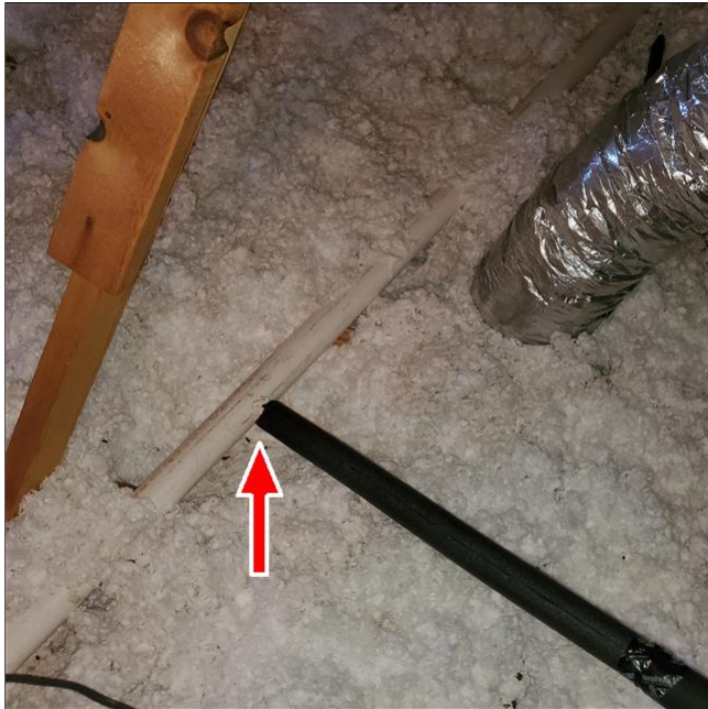
B. Item 3(Picture) Primary drain line terminates at a drain, waste, vent pipe.
