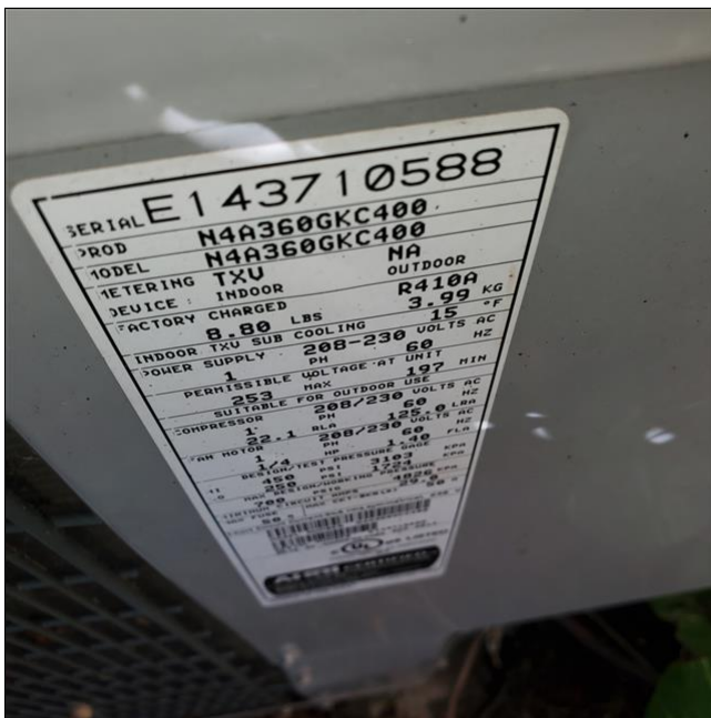
B. Item 1(Picture) AC was manufactured in 2014.
