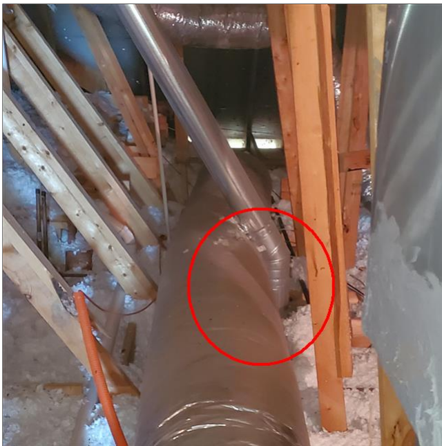
J. Item 1(Picture) Photo shows chimney flue in contact with duct.
