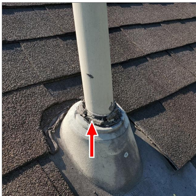
C. Item 8(Picture) This sealant deteriorates and leaks will occur here.
