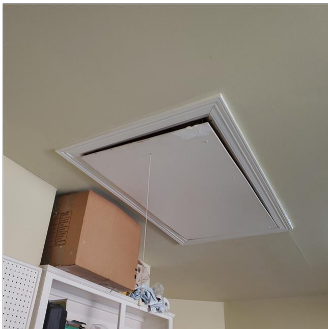
D. Item 1(Picture) Pull down not sealing.
