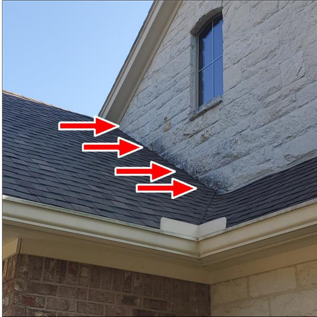
C. Item 5(Picture) Counterflashing not installed.
