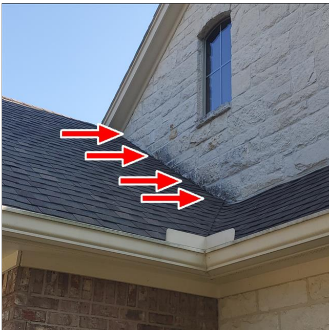
C. Item 5(Picture) Counterflashing not installed.
