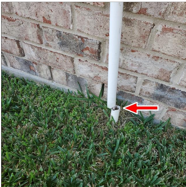
A. Item 3(Picture) Conduit was damaged.
