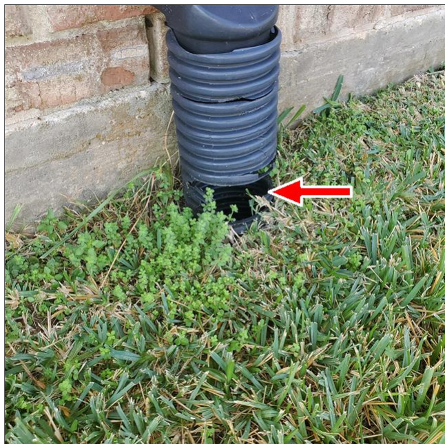
B. Item 2(Picture) Hole in black plastic downspout connector.
