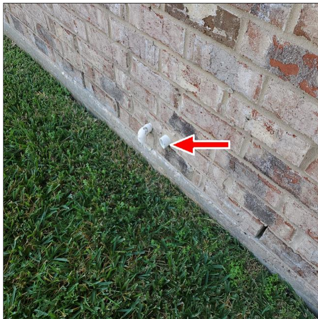
C. Item 2(Picture) Turndown was broken off.
