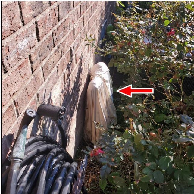
A. Item 2(Picture) Pipes were covered.
