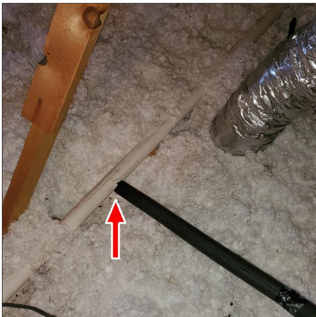
B. Item 3(Picture) Primary drain line terminates at a drain, waste, vent pipe.
