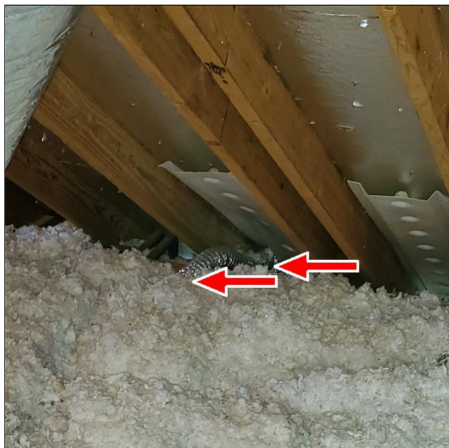
F. Item 1(Picture) Ducts terminate at soffit.
